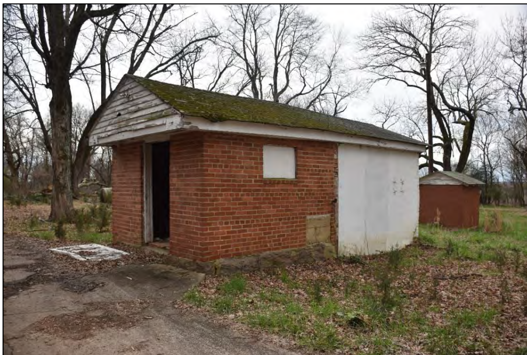
Figure 2.9. Boxwood Manor (CA0322), circa-1850/1910 dairy/well house and circa 1930 pump house, facing southwest.
