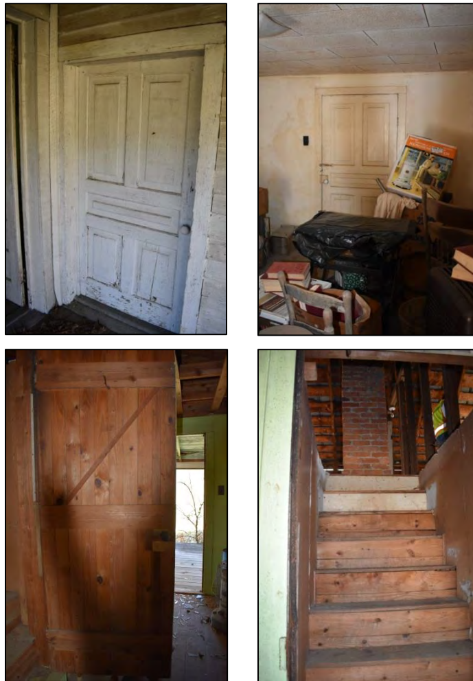
Figure 35: Left, five-panel door connecting ell and west room: right, door to attic and stairs
