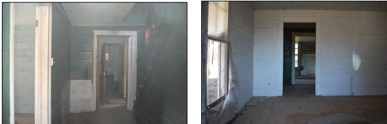
Figure 11: Left, view through front sidelight into stair hall and, beyond, ell and added bathroom—north parlor through opening at left; right, view through side window of south parlor with hall and north parlor beyond—note enclosure of hearth and removal of mantel in north parlor
