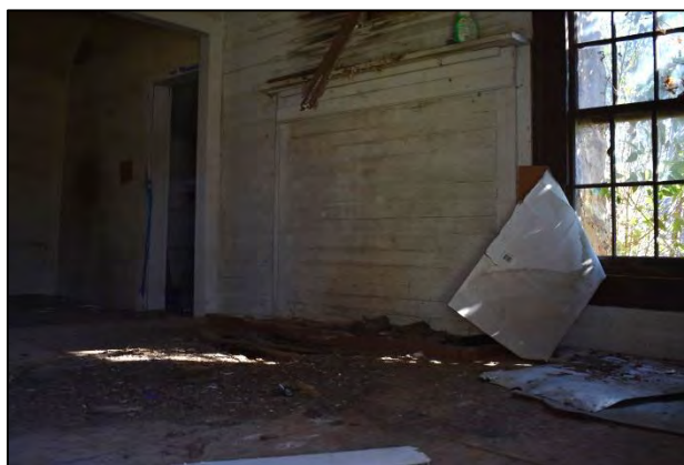
Figure 12: Mantel remaining on rear wall of ell; entry to later-added bathroom at left
