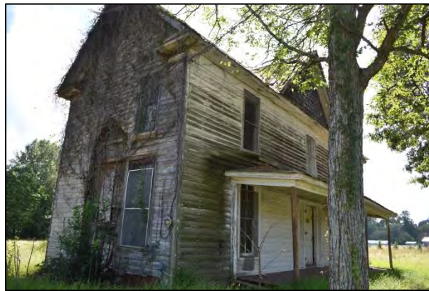
Figure 8: North side and west front elevations; note loss of chimney and boarding over of hearth opening
