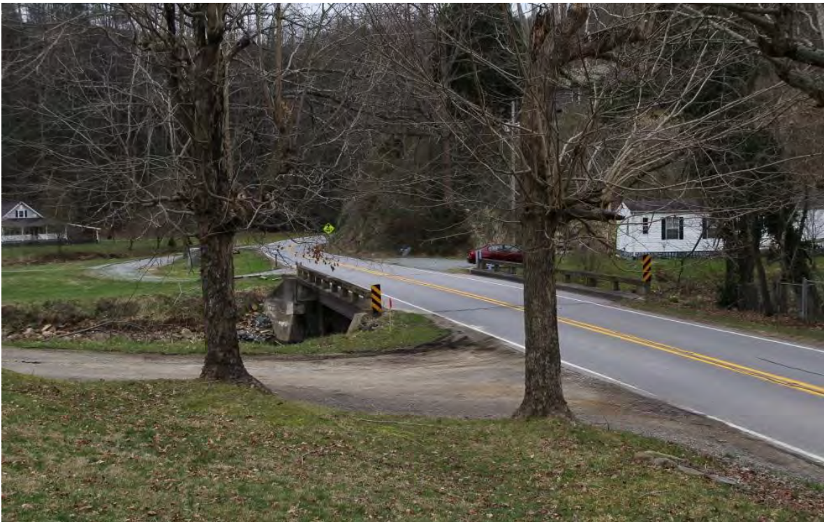
Bridge No. 15 on NC 212 over Shelton Laurel Creek, view southwest from Gentry-Tweed Homestead
