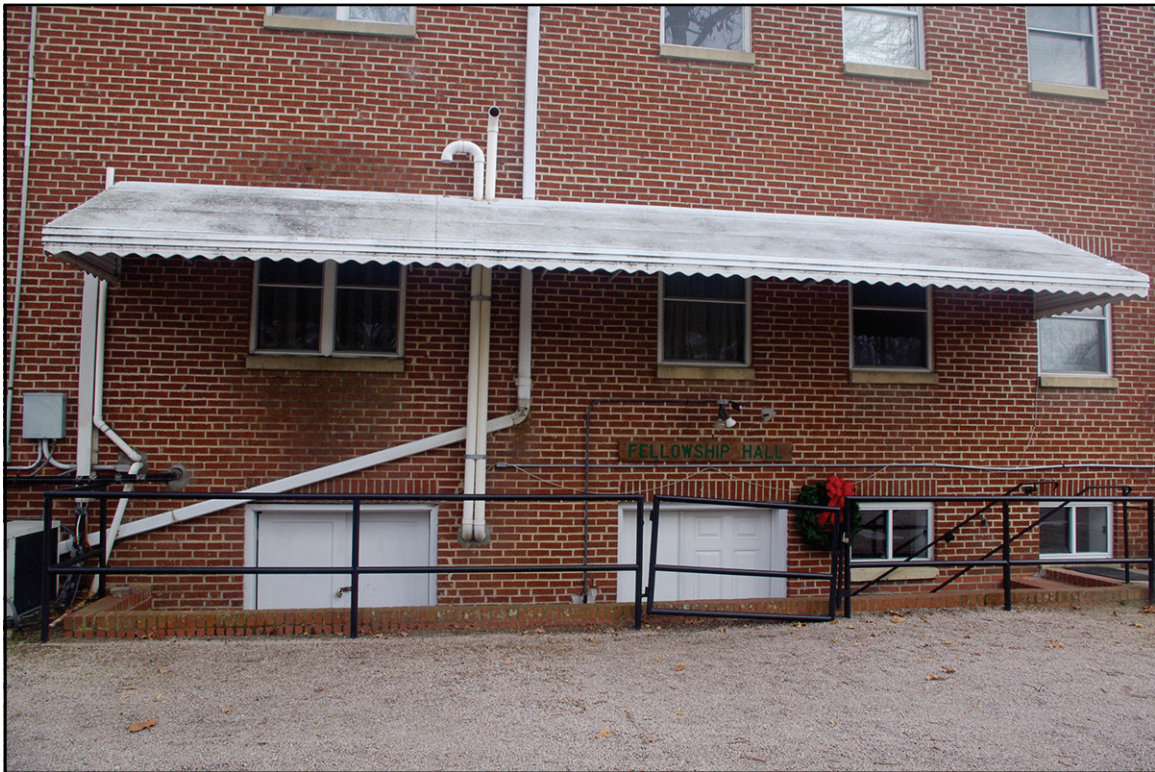
PLATE 7: Detail of Fellowship Hall Entrance, West Elevation, White Oak Baptist Church (JT1994), Johnston County, North Carolina
