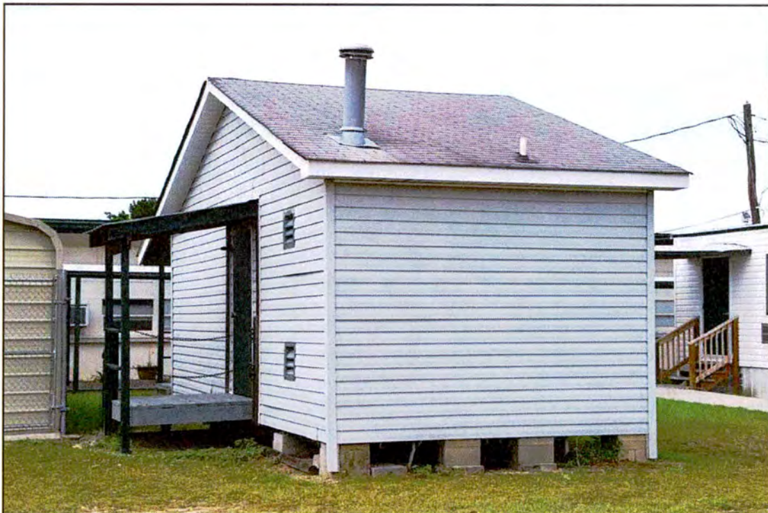
Figure 37. RB0701, Oxendine Elementary School, Portable Classroom 1, south and west elevations, view to the northeast.
