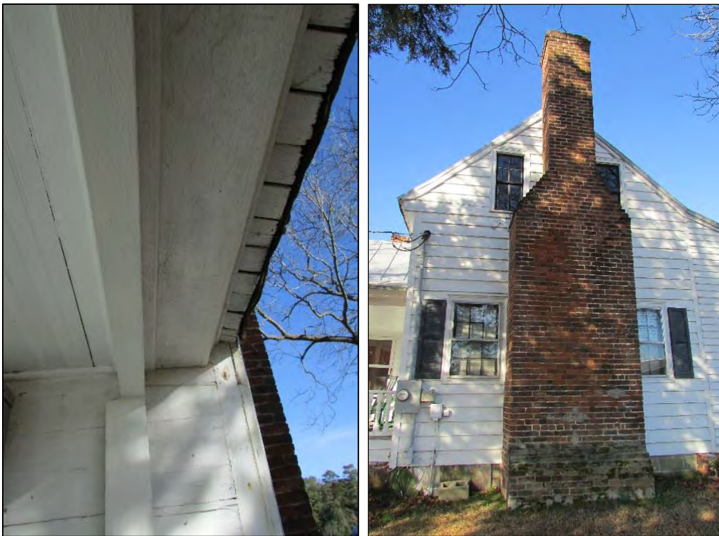
Photo 4: View of Original Shingles Underneath Metal Roof, East Elevation (Left) and View of Original Chimney on East Elevation (Right).
