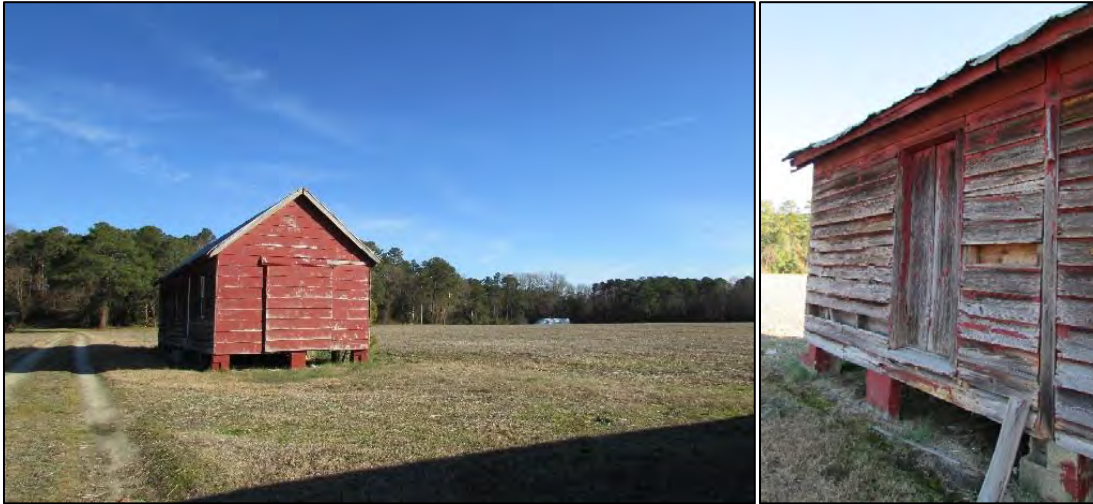
Photo 10: Tenant House, Looking North (Left); Detail of Door on Primary Elevation, Looking Northeast (Right).
