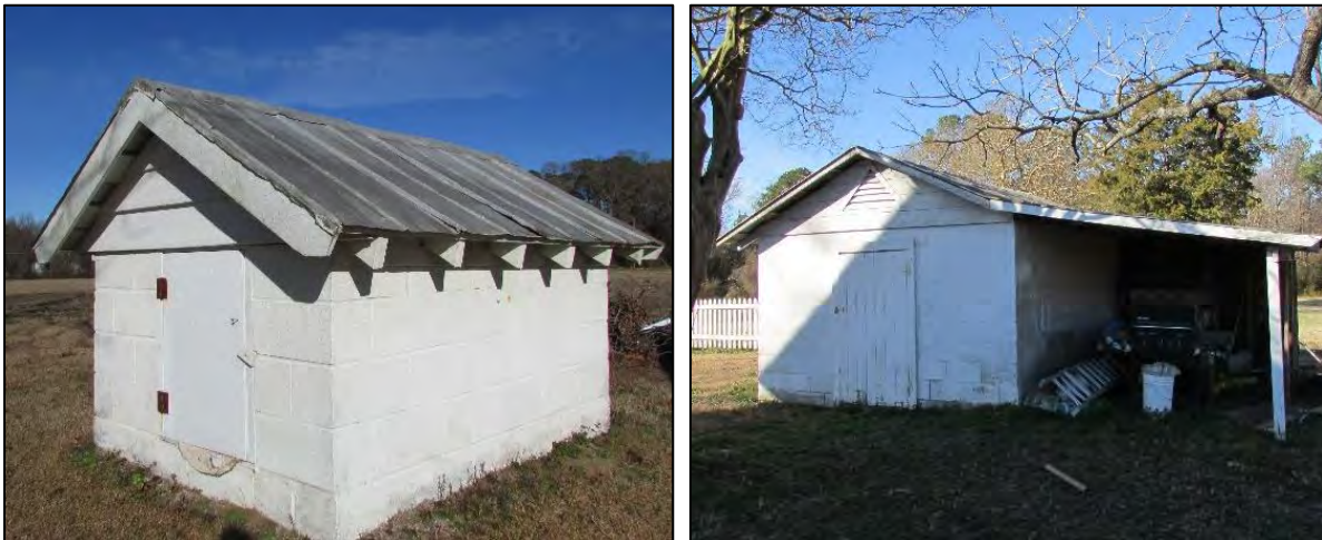
Photo 13: Northwest Oblique of Well-House, Looking Northwest (Left) and Primary (East) Elevation of Shed, Looking West (Right).
