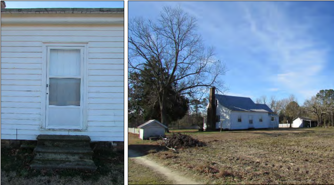
Photo 9: View of Door on North Elevation, Looking South (Left) and View of North Elevation, Looking Southwest (Right).
