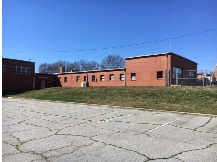
Figure 105. Facing southwest to main building's east elevation; assembly hall attaches via brick hyphen (Source: ALPHA Facilities Solutions)
