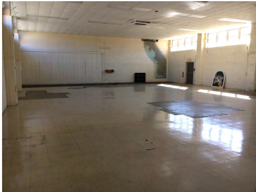
Figure 112. Assembly hall interior (Source: ALPHA Facilities Solutions)
