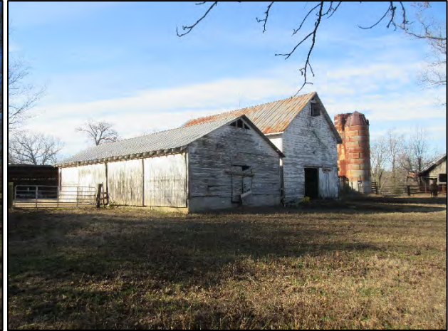
Equipment shed 3 (left), double crib barn and silos (right), view to the northwest
