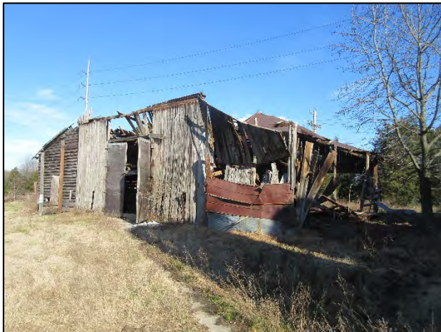
Hay barn (collapsed), view to northeast
