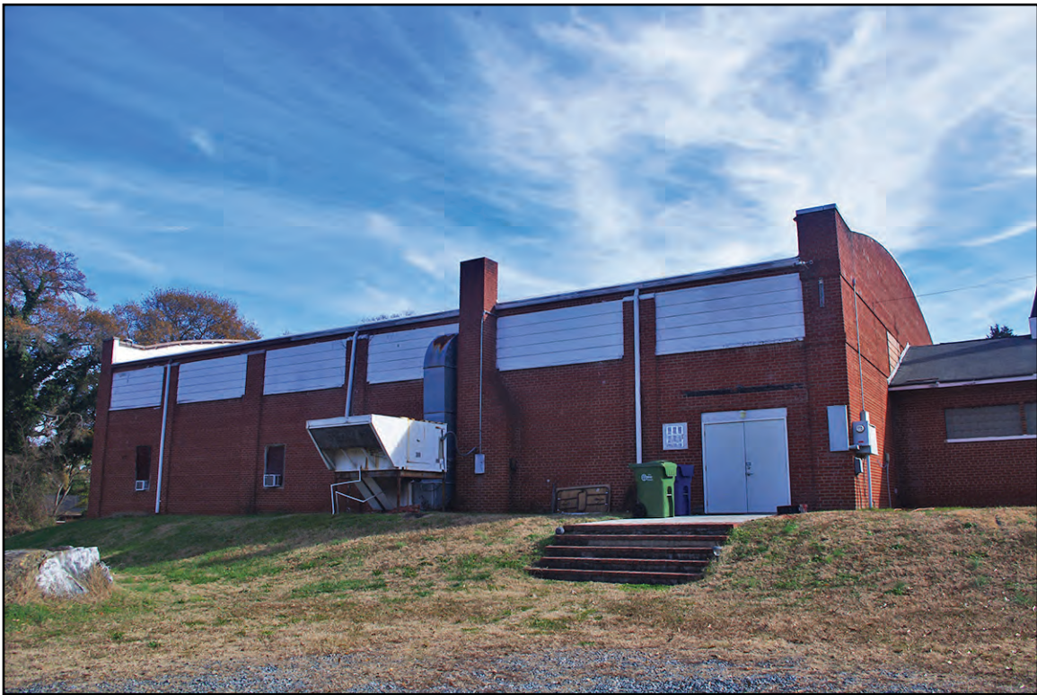
PLATE 31: West Elevation, Former Junior Chamber of Commerce Community Building (GS2423), Mount Holly, North Carolina
