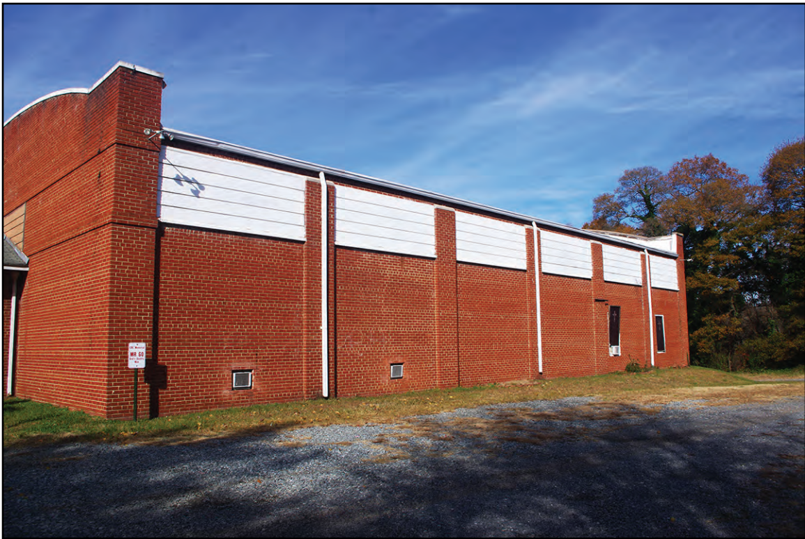
PLATE 21: East Elevation, Former Junior Chamber of Commerce Community Building (GS2423), Mount Holly, North Carolina
