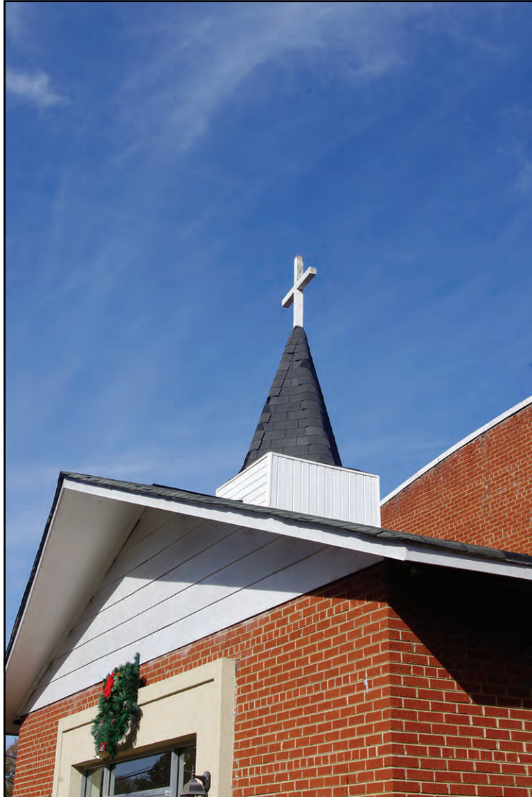
PLATE 20: Entrance Wing Roof Detail, South Elevation, Former Junior Chamber of Commerce Community Building (GS2423), Mount Holly, North Carolina
