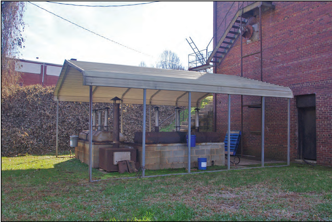
PLATE 6: Detail of Barbecue Pit Located off North Elevation, Mount Holly Lodge 544 AF & AM (GS2422), Mount Holly, North Carolina
