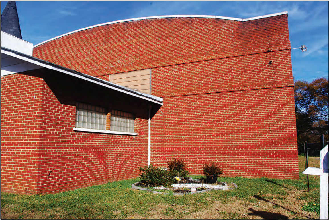
PLATE 32: Detail of New Roofline on Entry Wing of South Elevation, Former) Junior Chamber of Commerce Community Building (GS2423), Mount Holly, North Carolina
