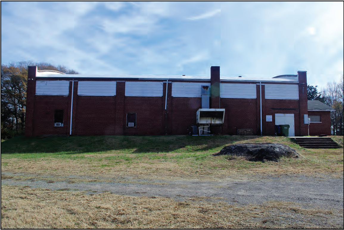
PLATE 22: West Elevation, Former Junior Chamber of Commerce Community Building (GS2423), Mount Holly, North Carolina
