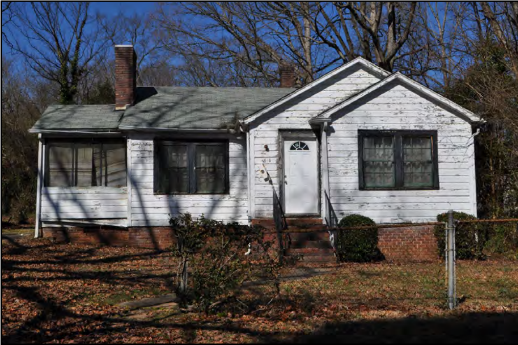
Plate 11.3: Typical Minimal Traditional house with original wood siding in Graham Heights (2905 Dogwood Avenue).
