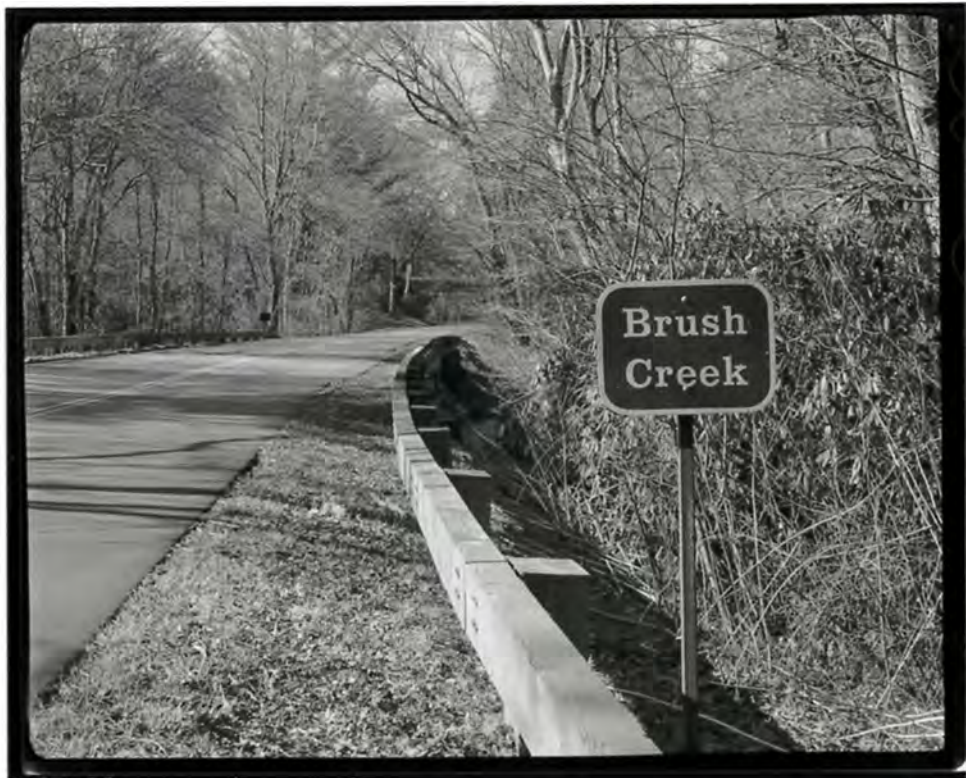
Photograph 27. View of Brush Creek Bridge #1, southbound on the Blue Ridge Parkway, looking west-northwest (NC-42-E-2).
