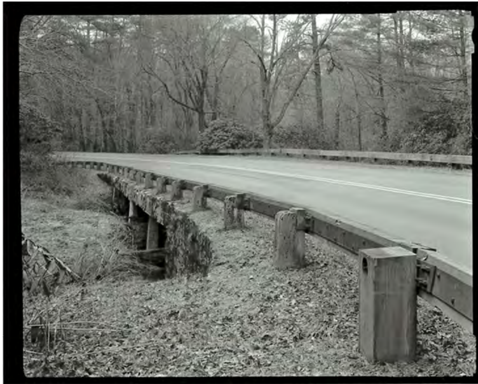
Photograph 17. View of the deck and guardrail of Big Pine Creek Bridge #3, looking west-northwest (NC-42-C-7).
