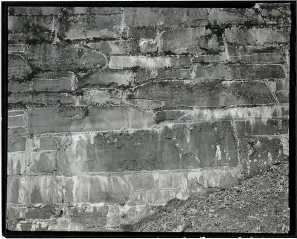
Photograph 34. Detail view of Brush Creek Bridge #1, showing the stonework at the abutment wall, looking northeast (NC-42-E-9).
