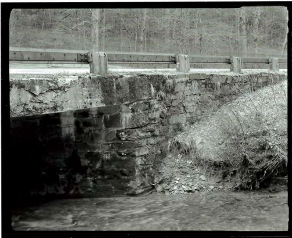
Photograph 24. Three-quarter view of Big Pine Creek Bridge #6, showing the south abutment, looking southwest (NC-42-D-6).
