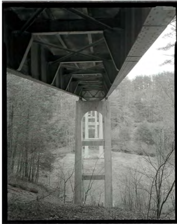
Photograph 7. Detail view of the girders of the Laurel Fork Viaduct, looking east-southeast (NC-42-B-9).
