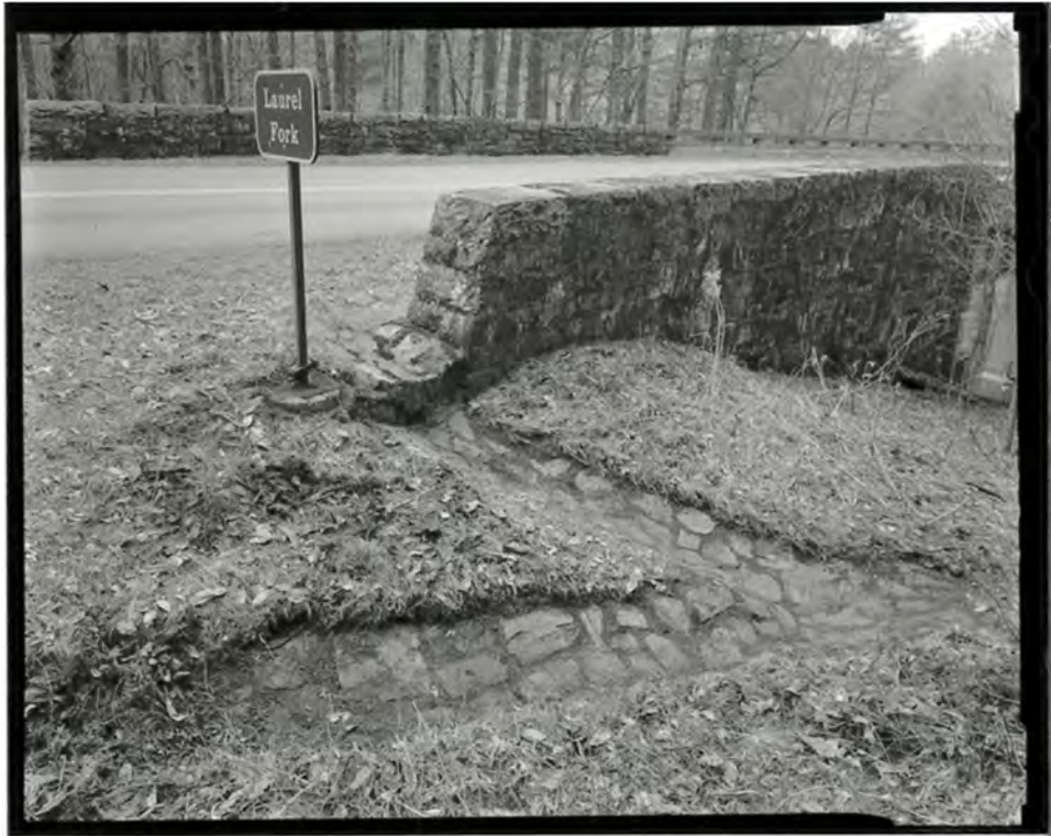
Photograph 9. View of the stone-faced parapet wall and detail of a stone-lined drainage channel, looking southwest (NC-42-B-12)
