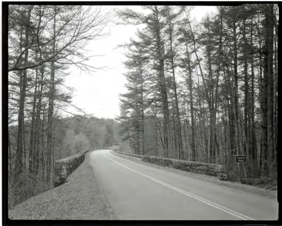
Photograph 10. View of the approach to the Laurel Fork Viaduct, showing the parapet, deck, and guardrails, looking west-northwest (NC-42-B-13).
