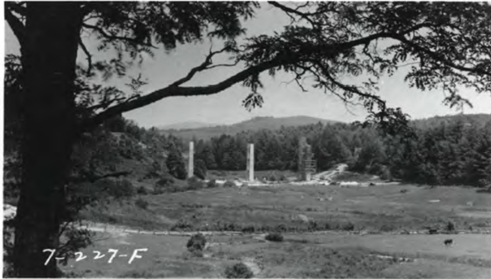
Figure 5. Photograph, ca. 1938, showing the construction of the piers for the Laurel Fork Viaduct (USDA BPR 1938).
