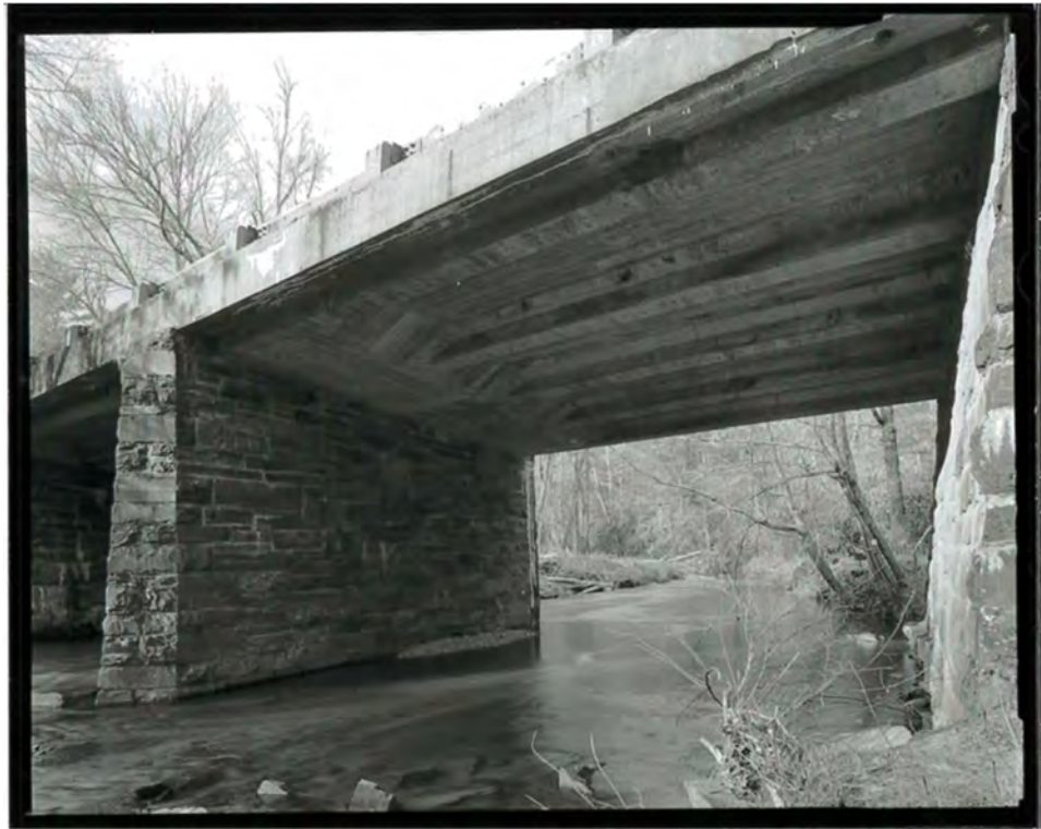
Photograph 30. Detail view of Brush Creek Bridge #1, showing the beams at the underside of the deck, looking north-northeast (NC-42-E-5).
