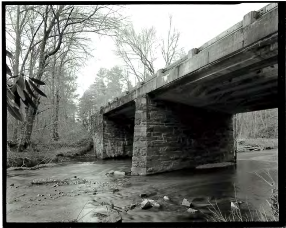
Photograph 31. Detail view of Brush Creek Bridge #1, showing the beams at the underside of the deck and the central pier, looking north (NC-42-E-6).
