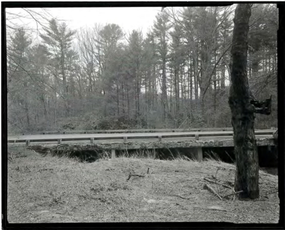
Photograph 12. View of the Big Pine Creek Bridge #3, showing the south-facing elevation, looking north (NC-42-C-2).
