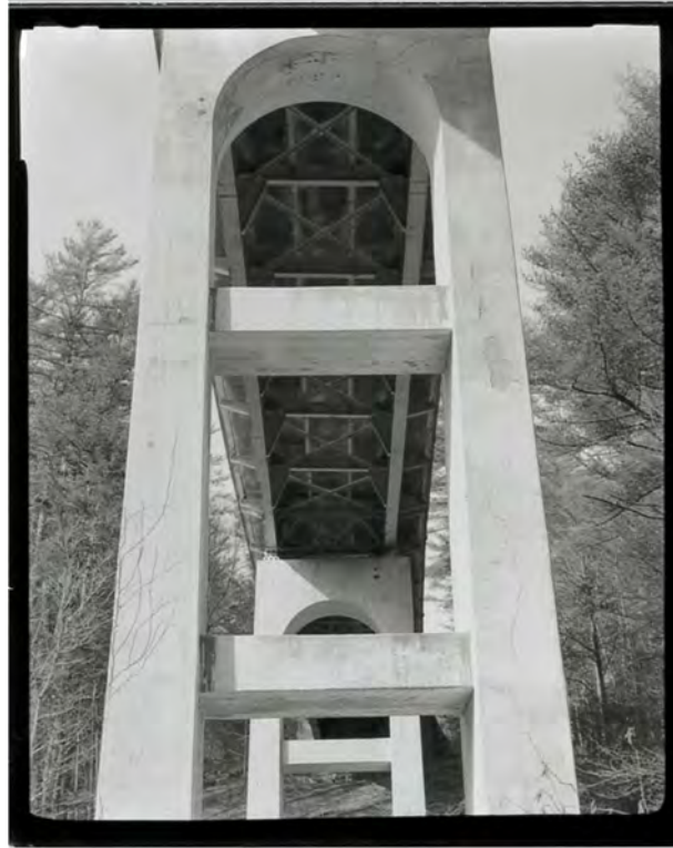
Photograph 3. View of the underside of the Laurel Fork Viaduct, showing the piers and girders, looking west-northwest (NC-42-B-3).
