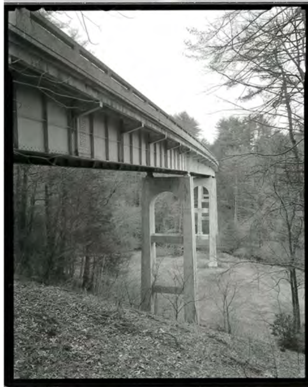
Photograph 6. Three-quarter view of the Laurel Fork Viaduct, showing the girders and piers, looking east (NC-42-B-8).
