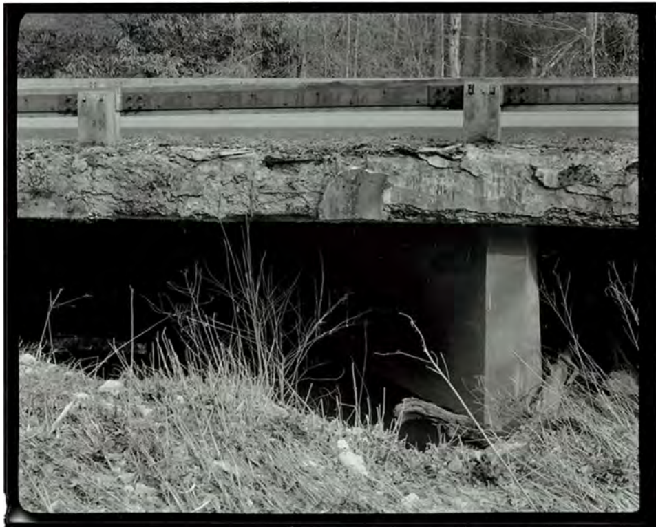
Photograph 14. Detail view of Big Pine Creek Bridge #3, showing the pier and deck, looking west (NC-42-C-4).
