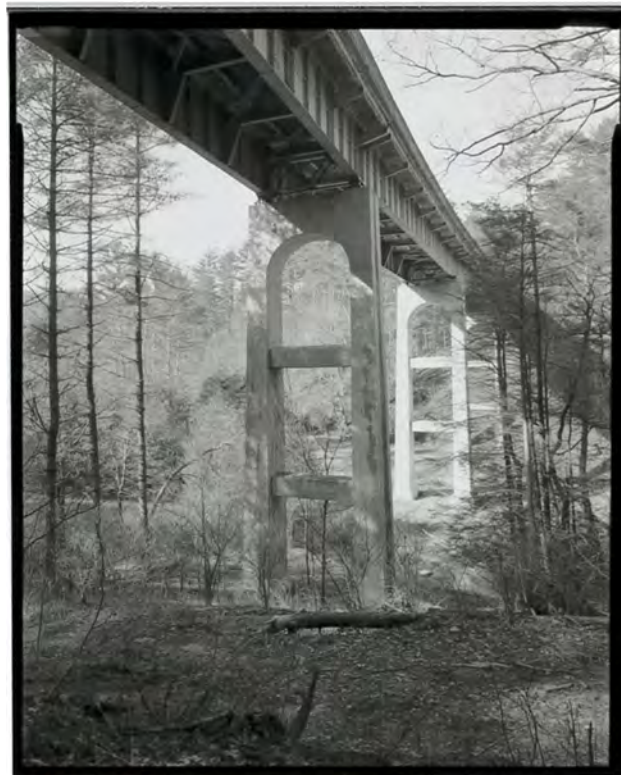
Photograph 2. Detail view of the piers of the Laurel Fork Viaduct, showing the girders and floor structure, looking southwest (NC-42-B-2).
