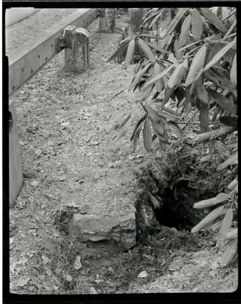
Photograph 25. View of Big Pine Creek Bridge #6, showing a stone drainage channel, looking northeast (NC-42-D-7).
