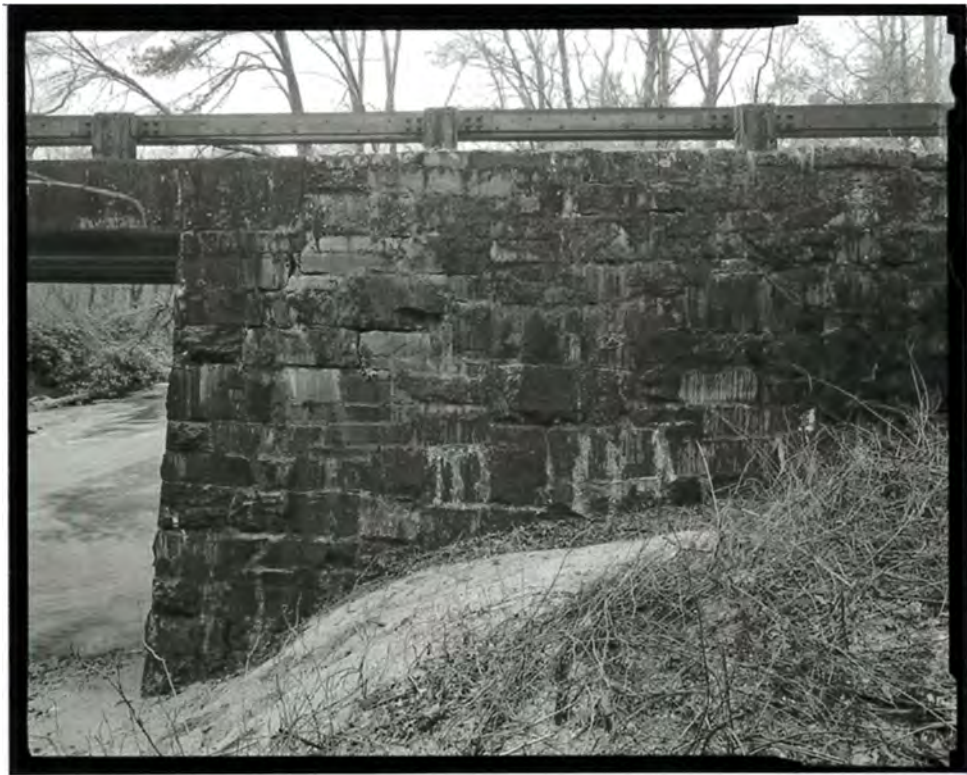
Photograph 29. Detail view of Brush Creek Bridge #1, showing the east abutment wall, looking northeast (NC-42-E-4).
