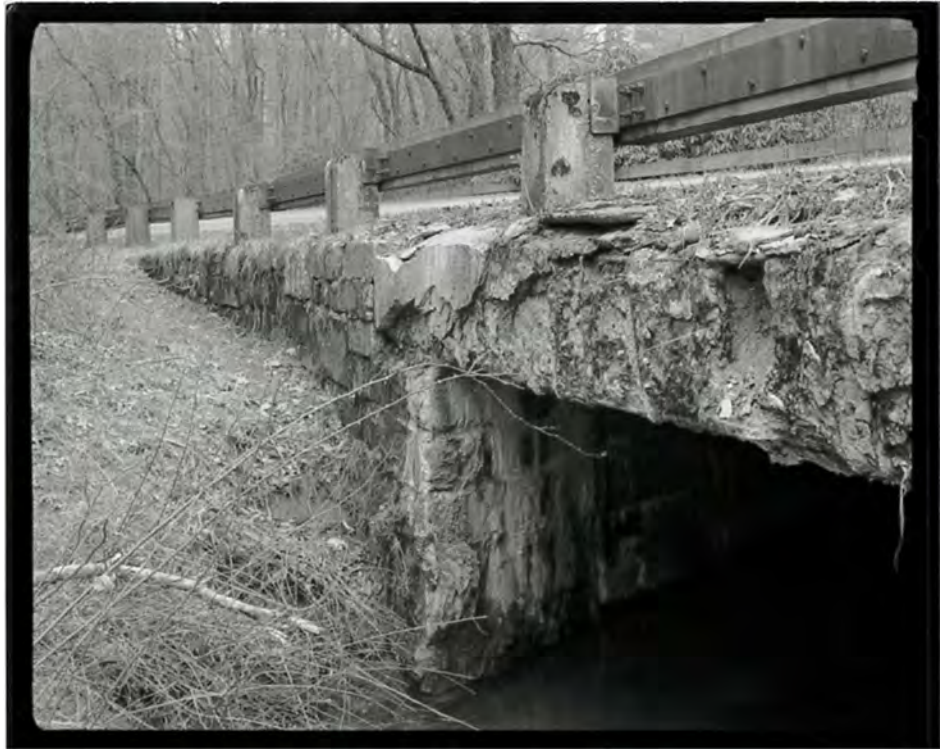
Photograph 15. Detail view of Big Pine Creek Bridge #3, showing the south abutment, looking northwest (NC-42-C-5).
