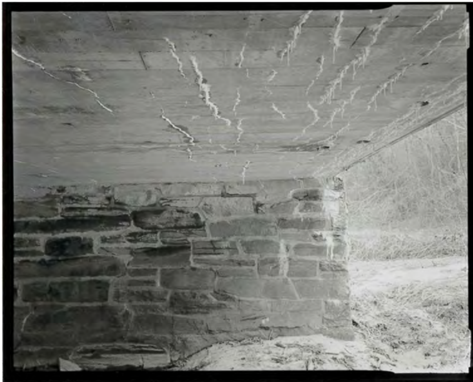
Photograph 22. Detail view of Big Pine Creek Bridge #6, showing the pier and underside of the deck, looking west (NC-42-D-4).
