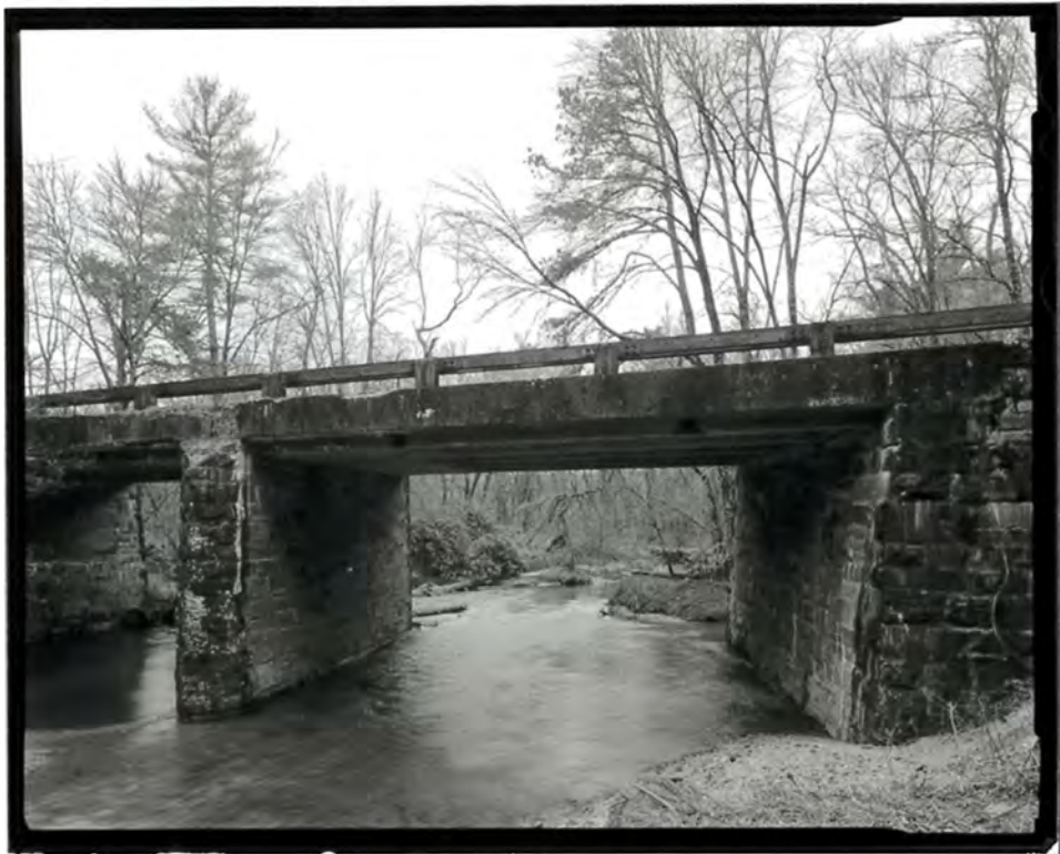
Photograph 33. View of Brush Creek Bridge showing east abutment and center pier, looking north (NC-42-E-8).
