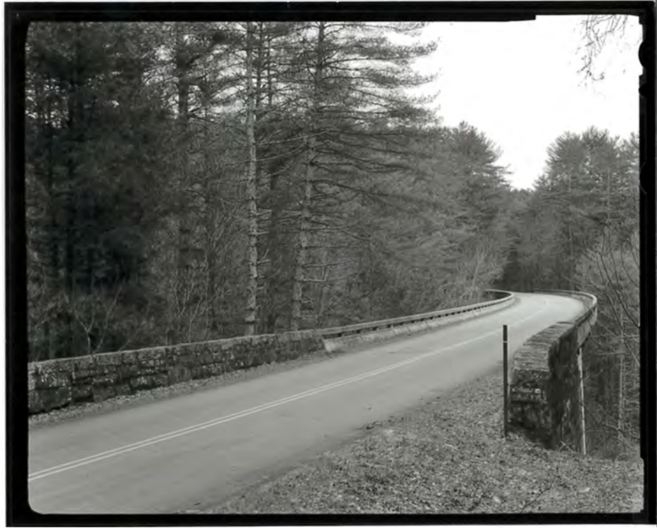
Photograph 5. View of the deck of the Laurel Fork Viaduct, looking east (NC-42-B-7).
