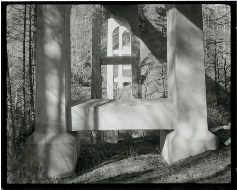
Photograph 1. Detail view of the bases of the piers of the Laurel Fork Viaduct, looking west (NC-42-B-1).
