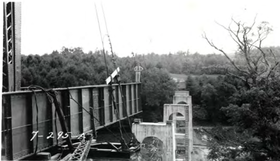
Figure 6. Photograph, ca. 1938, showing the erection of the girders for the Laurel Fork Viaduct (USDA BPR 1938).
