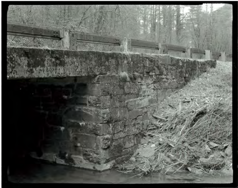
Photograph 16. Detail view of Big Pine Creek Bridge #3, showing the north abutment, looking east-northeast (NC-42-C-6).
