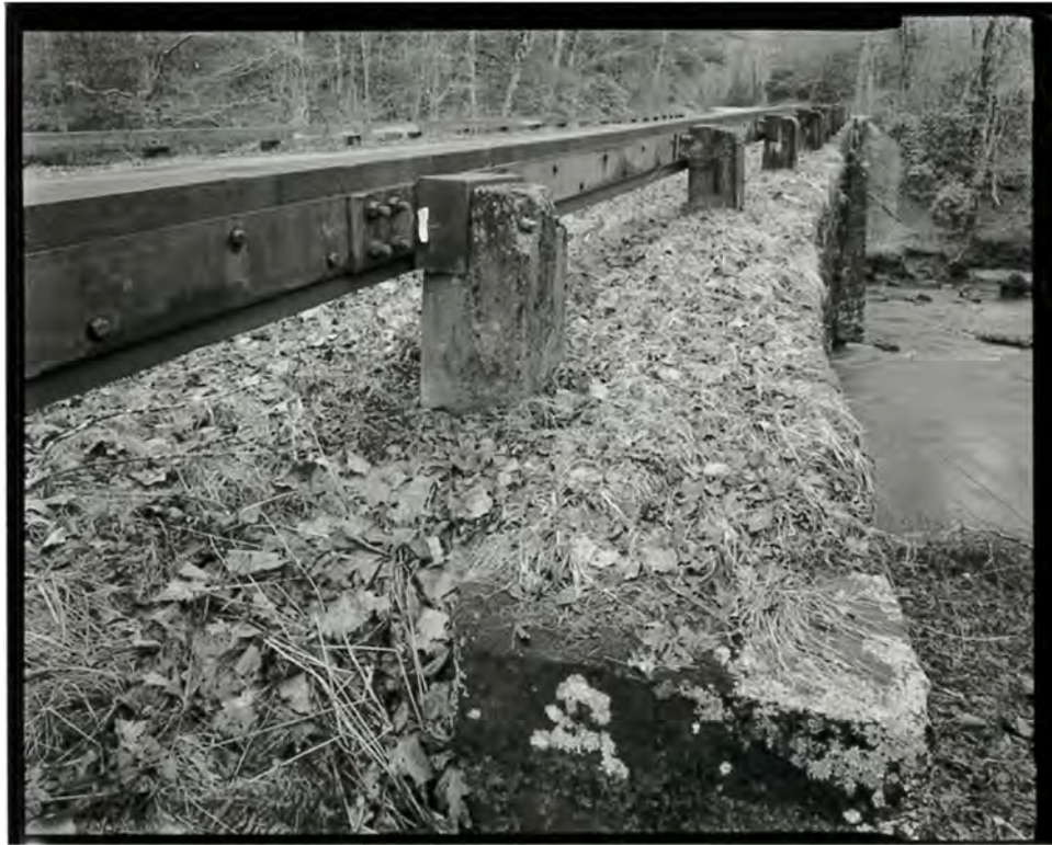
Photograph 28. Detail view of Brush Creek Bridge #1, showing the guardrail, looking northeast (NC-42-E-3).
