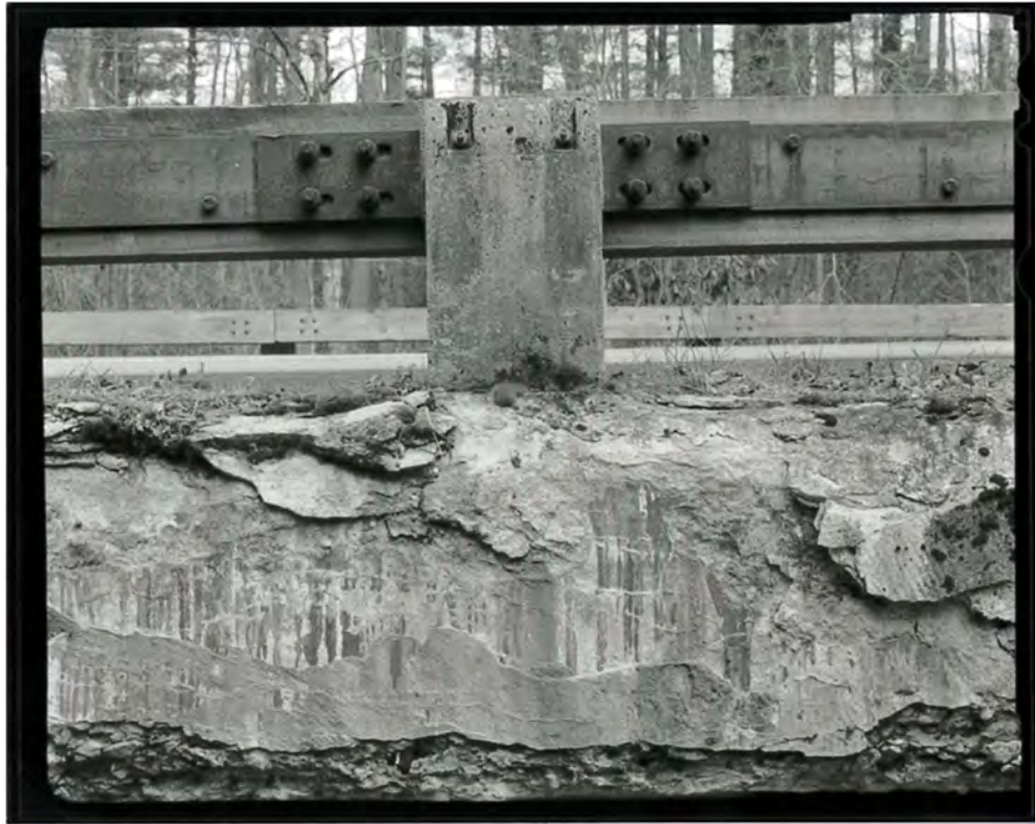
Photograph 13. Detail view of Big Pine Creek Bridge #3, showing the deck and guardrail, looking north (NC-42-C-3).
