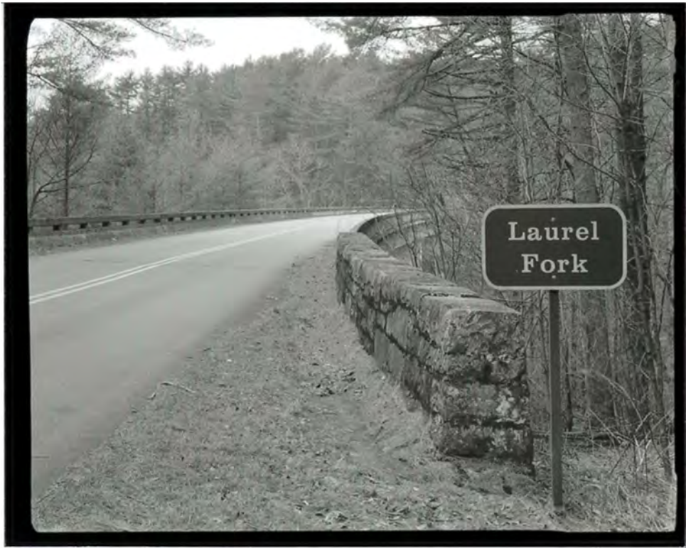
Photograph 8. View of the deck of the Laurel Fork Viaduct, looking west. The stone-faced parapet wall and concrete guardrail are visible (NC-42-B-11).
