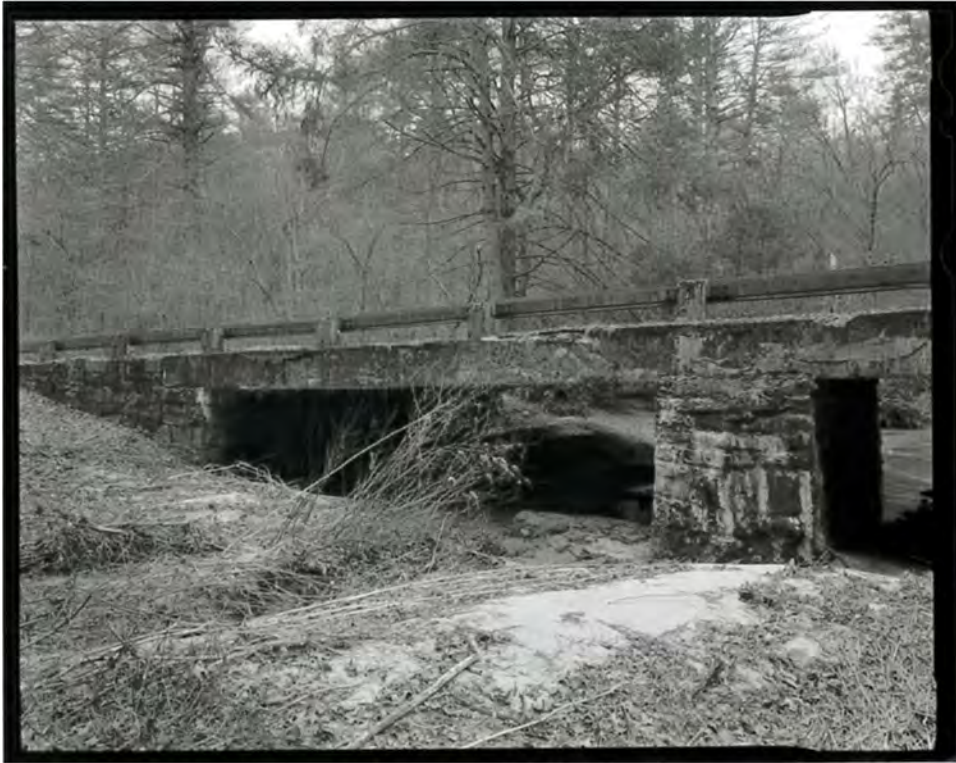
Photograph 23. Three-quarter view of Big Pine Creek Bridge #6, showing the north abutment, looking east-southeast (NC-42-D-5).
