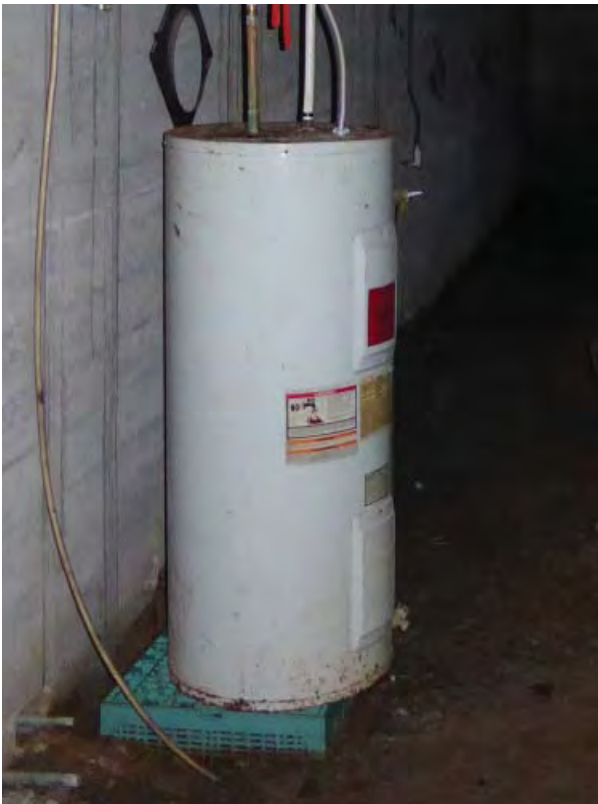
Figure C44. Electric hot water heater in Room 000.
