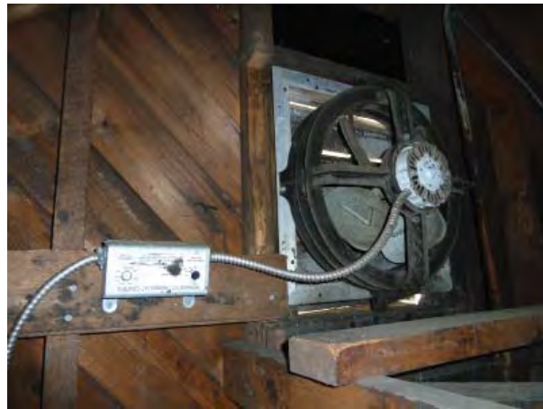
Figure C42. Electric attic ventilation fan. Note thermostat at left.
