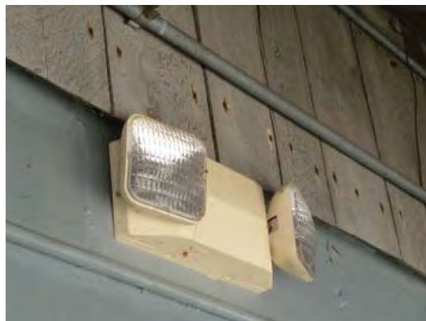
Figure C50. Typical emergency lighting fixture.
