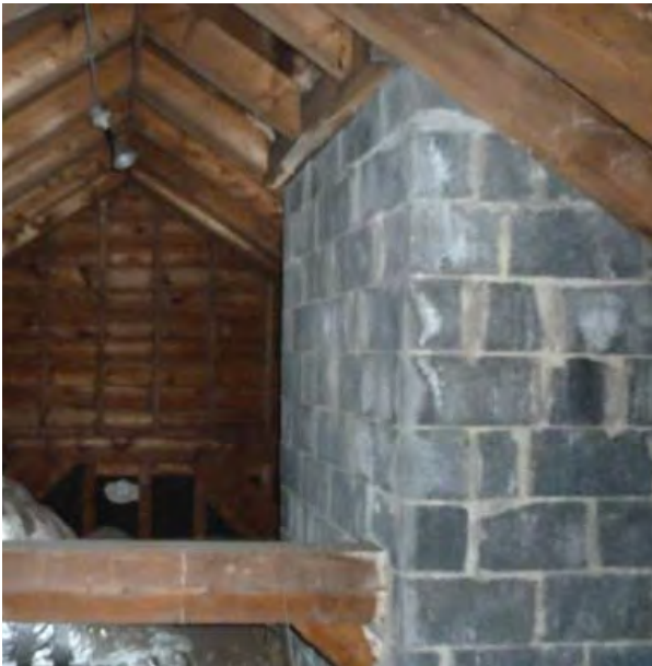
Figure C105. View of chimney in the attic. Note water damage left of the chimney, and signs of moisture on CMU.
