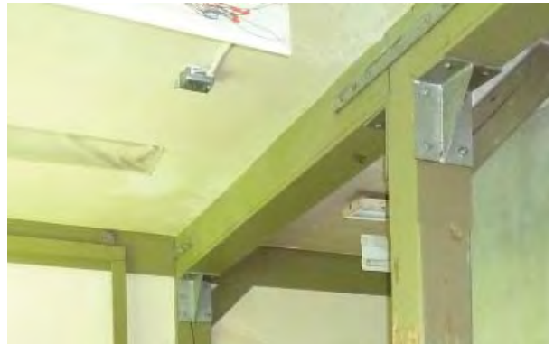
Figure C27. Metal plates and ties at ceiling beam in Room 102.
