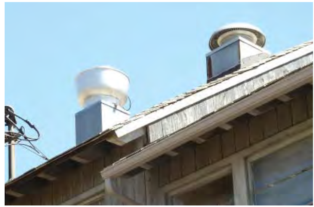
Figure C107. Commercial vents on north roof slope.
