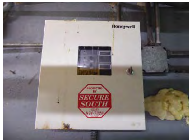
Figure C54. Honeywell alarm system panel in Room 006.
