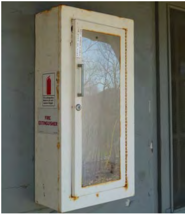
Figure C51. Empty fire extinguisher cabinet on north elevation.
