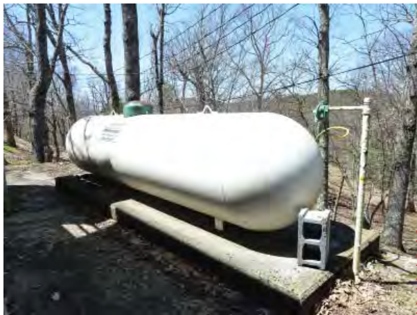
Figure C11. Propane tank at base of exterior stair.
