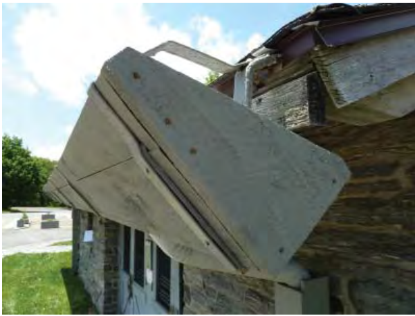
Figure C110. Larger aluminum-lined wood gutter above entrance. Gutter on west wing is similar.
