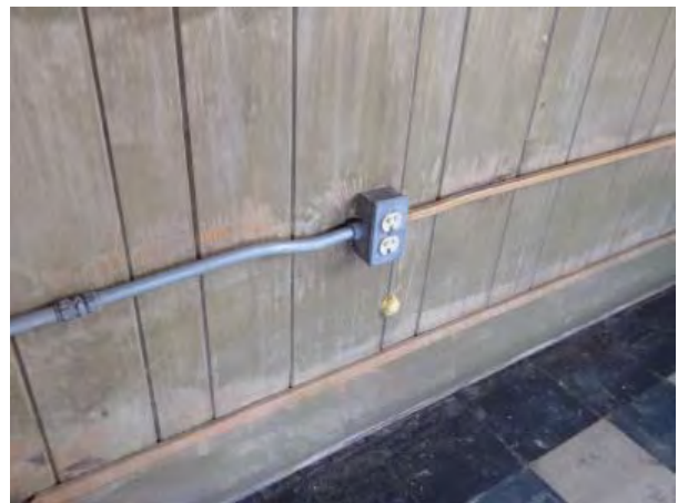
Figure C183. Typical v-groove paneling and baseboard in Room 101A. This area at the east end of the north wall is likely an example of the original wall finish.
