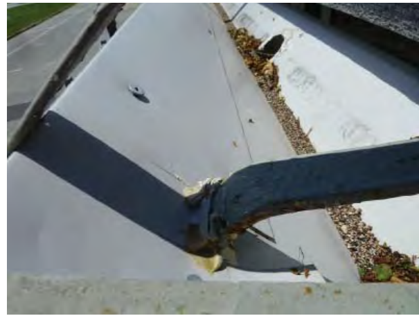
Figure C112. Bracket passing through aluminum liner on large gutter.
