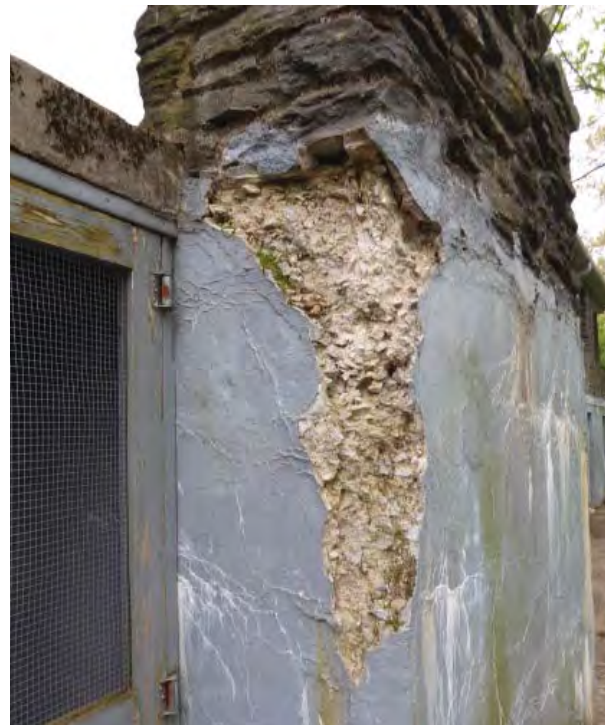
Figure II-8. Example of severe spalling at far east end of retaining wall, adjacent to exterior staircase.
