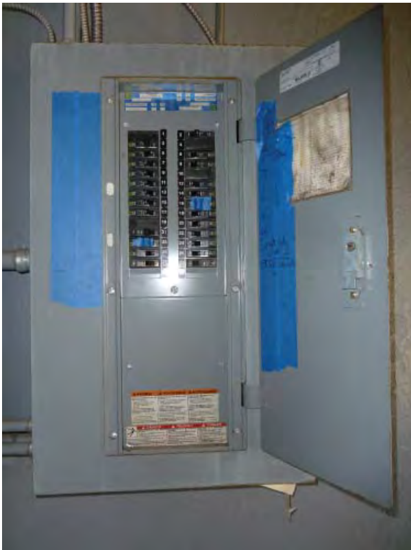
Figure C40. Electrical panel on west wall of Room 007.
