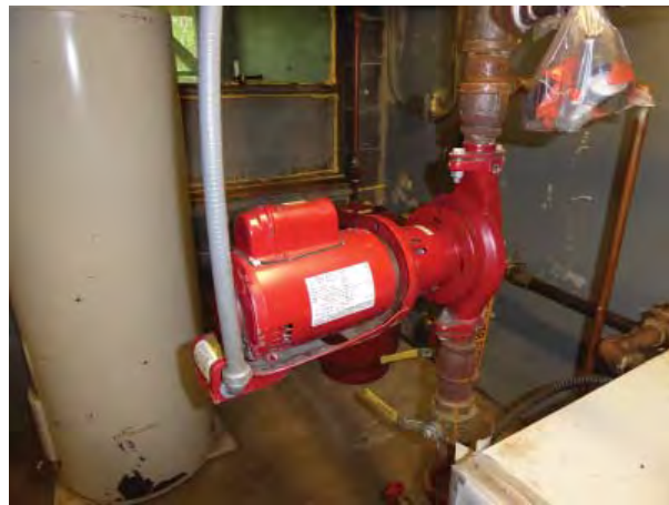
Figure C33. Typical boiler pump.
