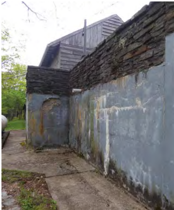
Figure II-7. Concrete retaining wall between coffee shop and service station. Note extensive deterioration.
