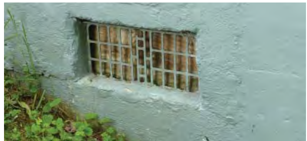
Figure C137. Blocked crawl space vent, viewed from exterior.
