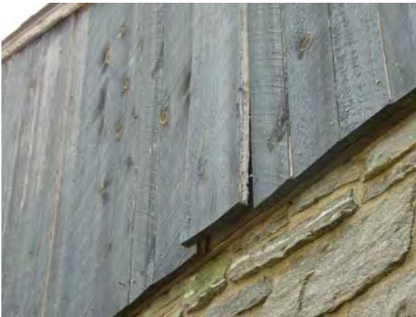
Figure C60. Recently-replaced siding on west gable end of main body. Note warped board; also note popped nails.
