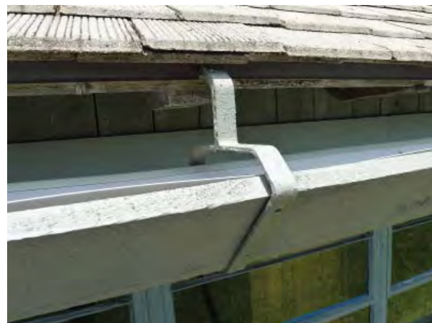
Figure C114. Metal bracket supporting small gutter.
