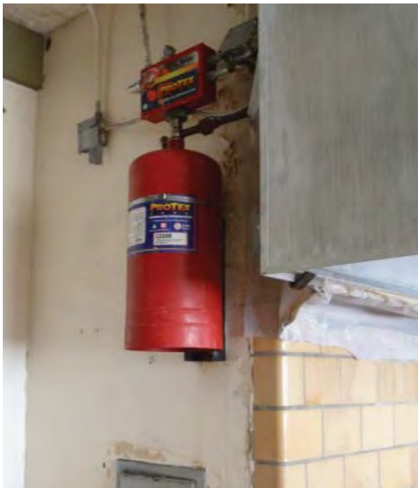
Figure C52. Remaining fire extinguisher near vent hood in Room 102.
