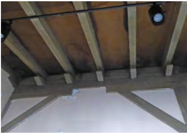
Figure C207. Water damage along north wall in Room 101B.
