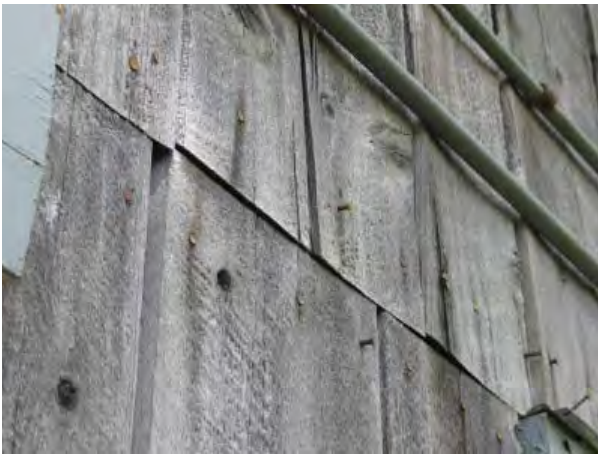
Figure C59. Detail of siding at top of window and door openings on east elevation. Note popped nails.
