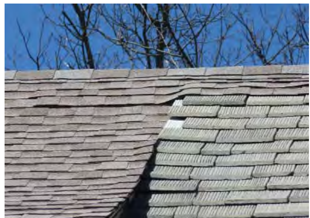
Figure C101. Temporary composition shingles meeting cement shingles east of chimney.
