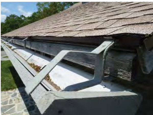
Figure C111. Metal bracket supporting large gutter.
