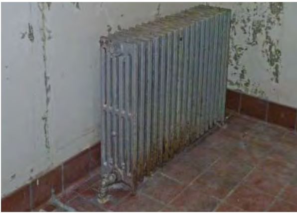
Figure C35. Floor-mounted radiator in Room 105A.
