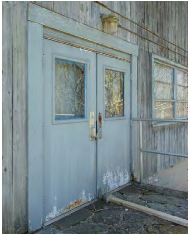
Figure II-10. Deteriorated, poorly-detailed replacement doors in east doorway.
