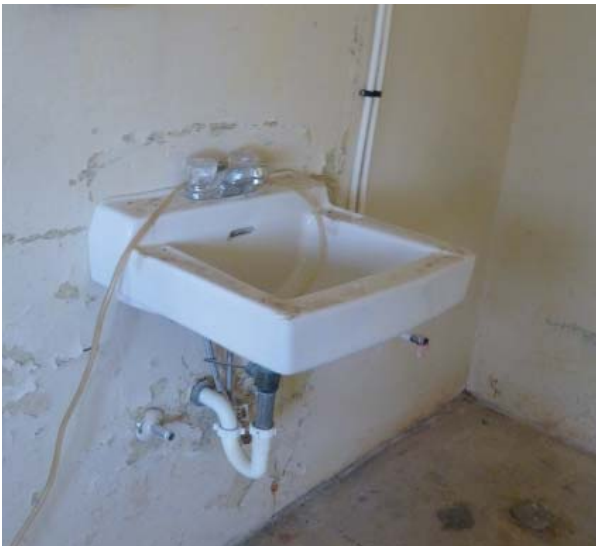
Figure C147. Disconnected lavatory on east wall.
