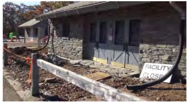
Figure B29. Drainage work in progress in November 2016. Note excavated foundation wall left of the doors. ( https://goo.gl/images/UbnngBb )
