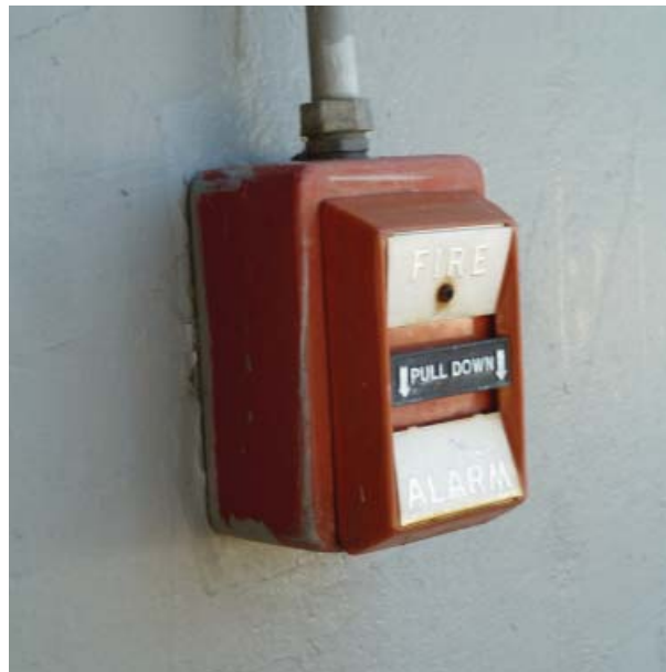
Figure C49. Fire alarm pull station on north elevation near doorway to Room 009.
