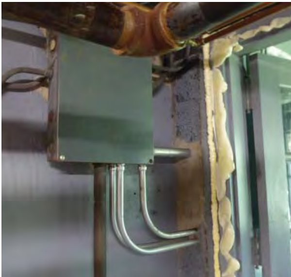
Figure C41. Junction box in Room 006.
