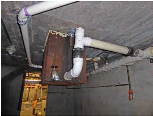
Figure C168. Grease trap on ceiling.
