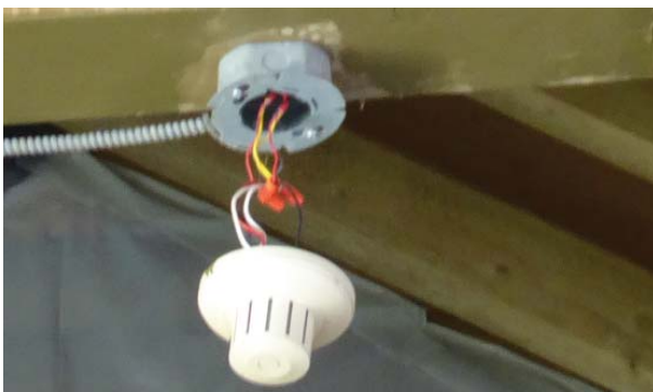
Figure C47. Typical wired smoke detector, detached from fixture box.
