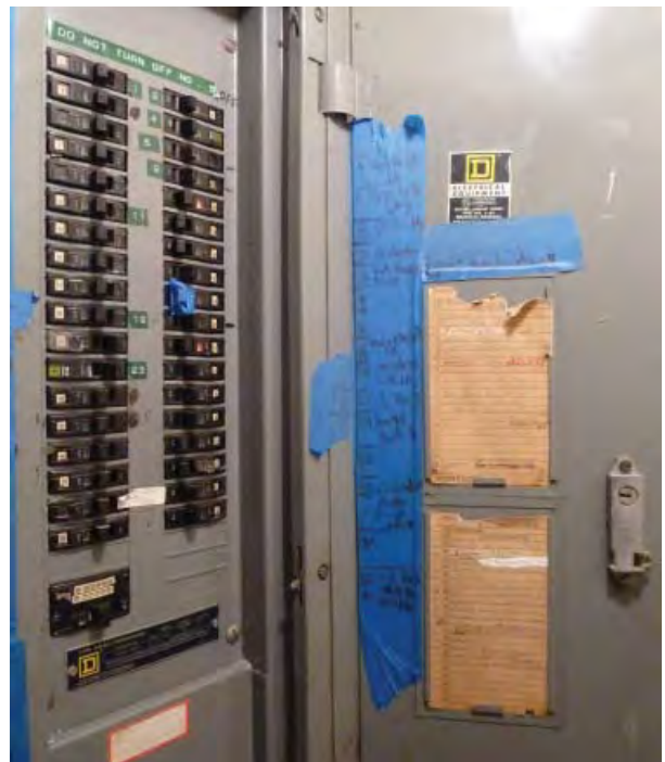
Figure C39. Electrical panel in closet of Room 101B.
