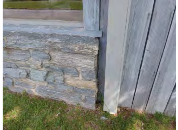
Figure C21. Termination point of stone exterior wall at eastern end of south dining room windows. Wood-framed exterior wall at right.
