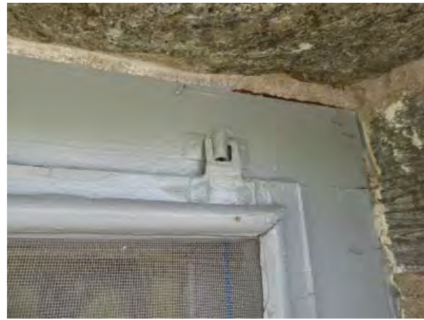
Figure C75. Typical screen and casing detail. Note rusted lintel at top right.
