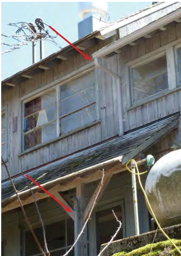
Figure C116. Aluminum gutter and downspout on north elevation of west wing. Note downspout for rear porch.
