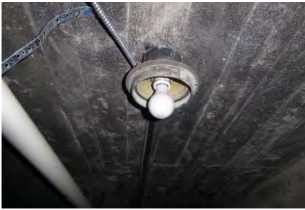
Figure C167. Typical ceiling fixture in Room 008.
