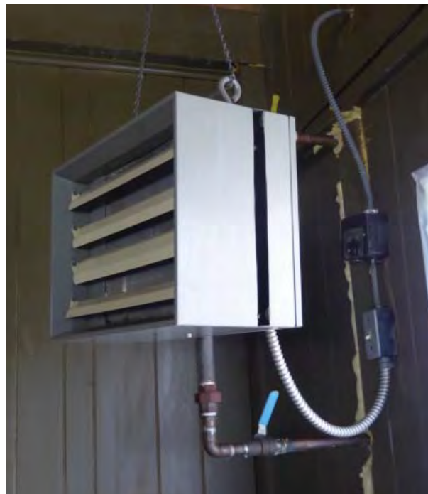
Figure C34. Typical wall-mounted unit in Room 101A
