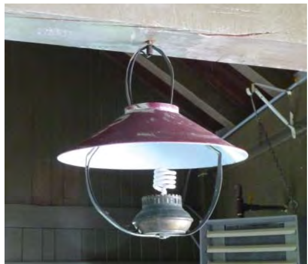
Figure C200. Typical early one-lamp fixture.
