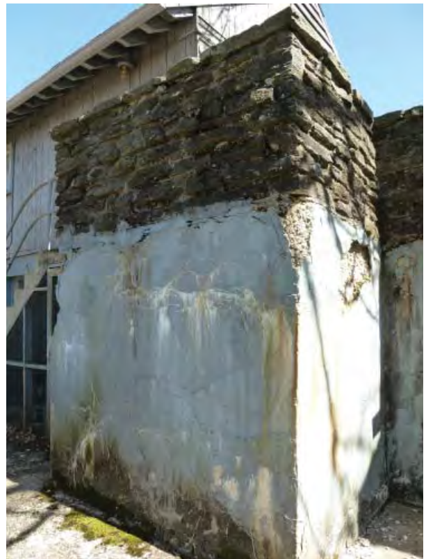
Figure C8. Concrete retaining wall and stone railing. Note heavy deterioration of concrete due to moisture.
