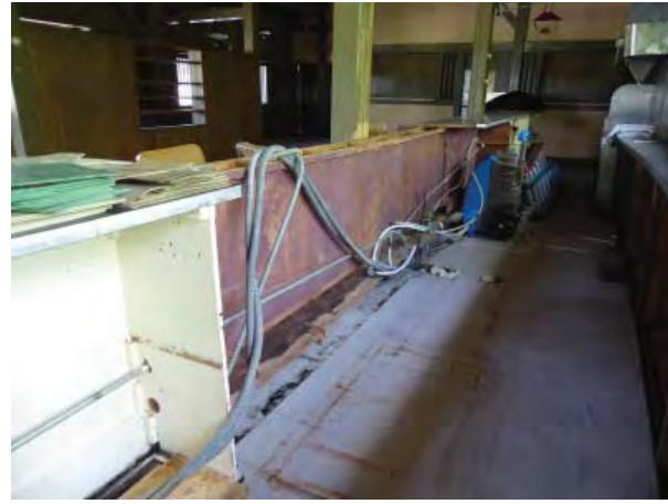
Figure C195. Back of serving counter showing general condition. Note replacement tile.
