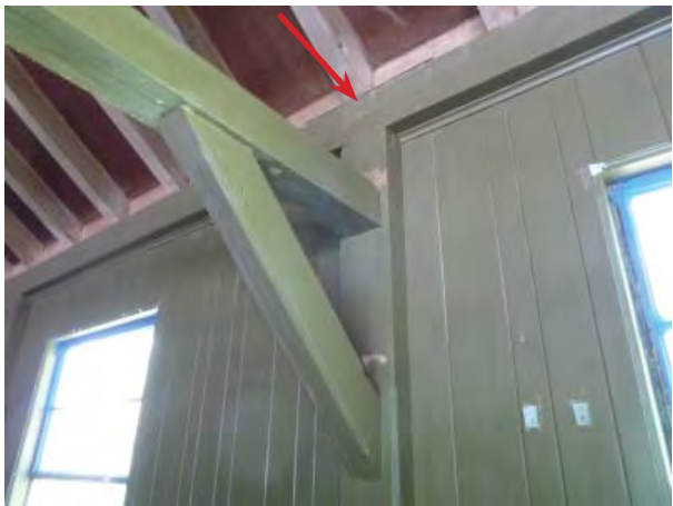
Figure C25. Typical chamfered bracket and embedded timber post on north wall. Note lap joint at top of post.
