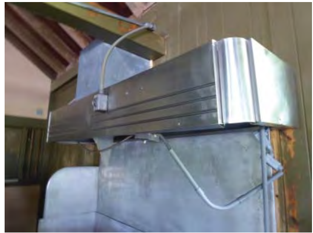
Figure C198. Original stainless steel hood on north wall.
