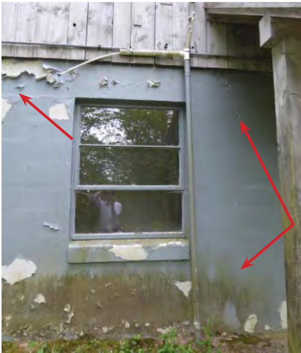
Figure C55. Foundation wall on north elevation. Note seam for concrete header and floor slab (left), and seam for concrete column (right).
