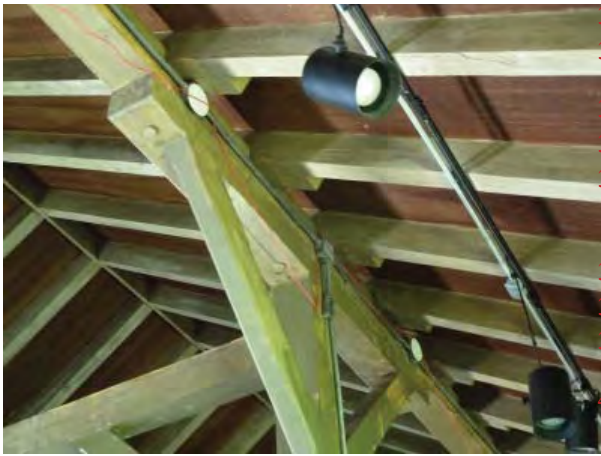
Figure C201. Typical track lighting fixtures. Note earlier fixture boxes mounted on side of beam.
