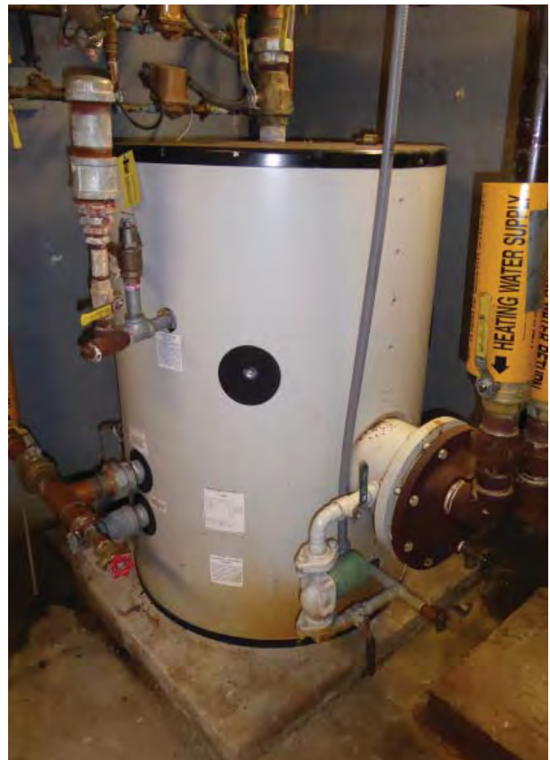
Figure C46. Indirect hot water heater connected to boiler in Room 006.
