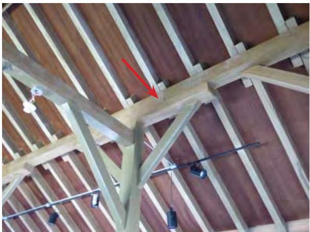
Figure C26. Typical beam at main center aisle post. Arrow indicates a wood key. Note exposed rafters.
