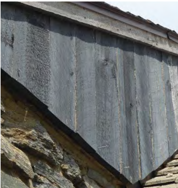
Figure C61. Recently-replaced siding on east wall of projecting south bay. Note popped nails.
