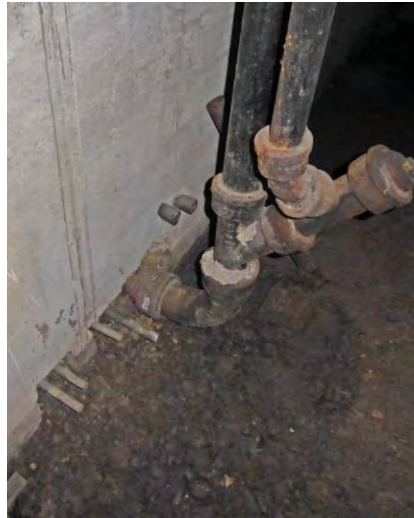
Figure C133. Cast iron drain pipe and severed plumbing and heating pipes at base of north wall.
