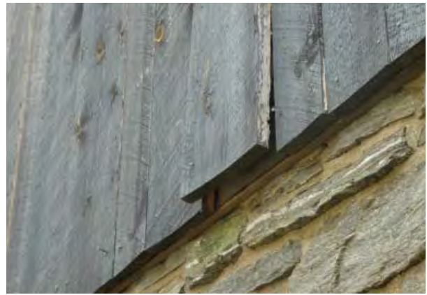
Figure II-9. Example popped fasteners and warped board on west wall of south bay.
