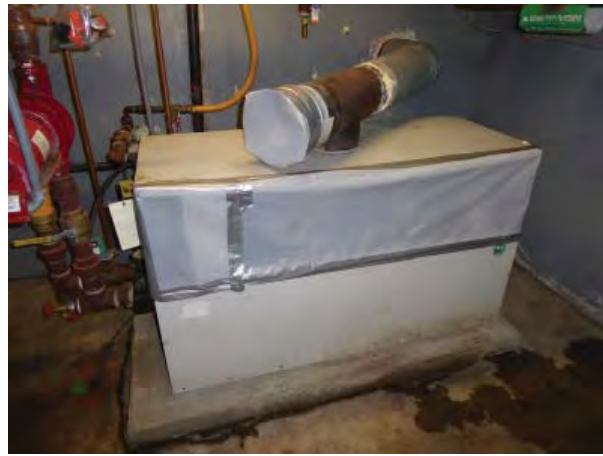
Figure C32. Hot-water boiler in Room 006.
