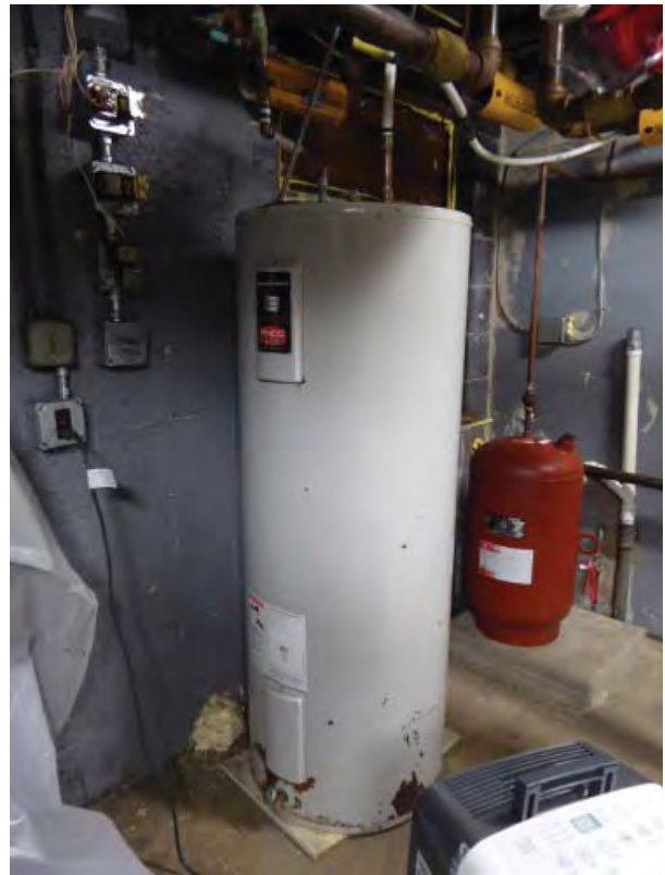
Figure C45. Electric hot water heater in Room 006.
