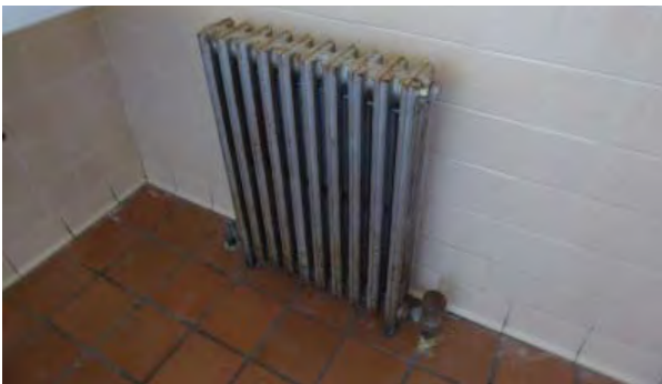
Figure C36. Floor-mounted radiator in Room 106B.
