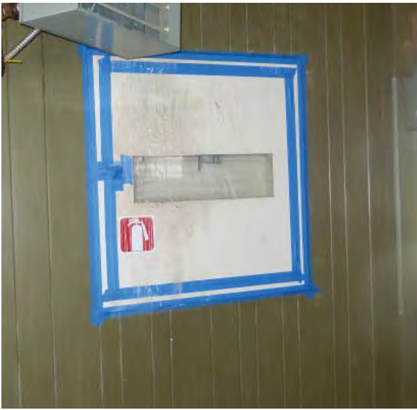
Figure C204. Firehose cabinet on south wall.
