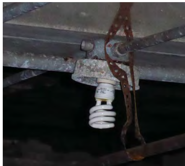
Figure C134. Typical surface-mounted fixture in Room 000.
