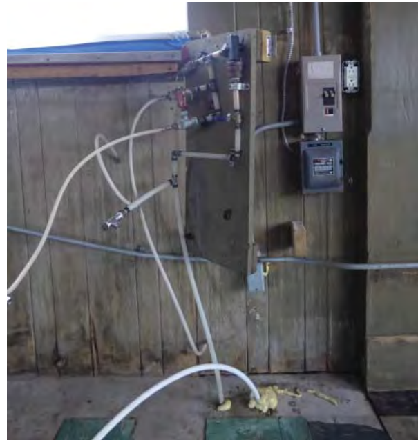
Figure C202. Flexible water lines and disconnect switches on north wall.
