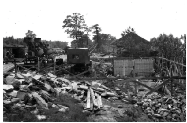
Figure B6. The coffee shop under construction in September 1948, looking west. The service station, appearing near completion is visible in the distance. (BLRI Coll.)
