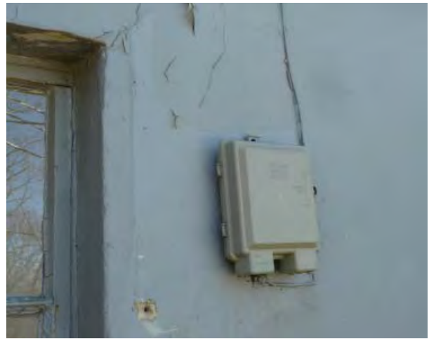
Figure C53. Telephone network interface box at west end of north elevation.
