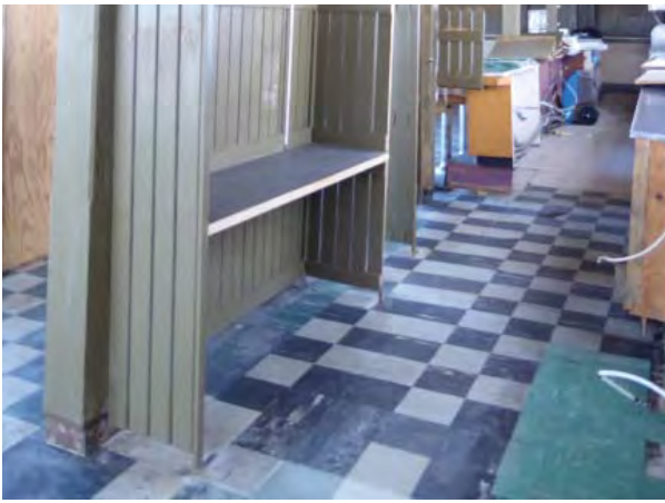
Figure B17. Asphalt tile patch where original section of counter was removed (JKOA, 2018)
