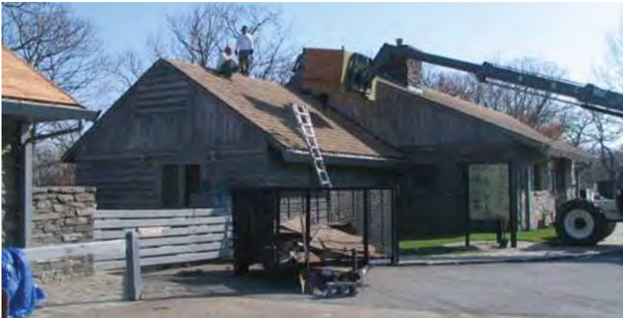
Figure B28. Re-roofing underway in 2010. Exposed sheathing is visible on the service station at left. (Superintendents Annual Report, 2010)
