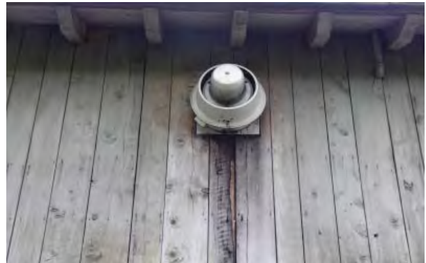
Figure C108. Wall vent on north elevation. Note discoloration of siding beneath.
