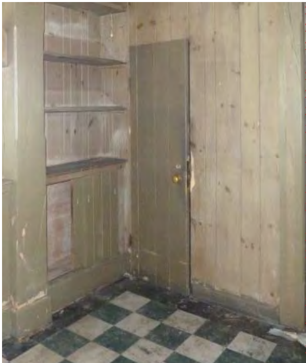
Figure C209. Concealed closet door in southeast corner. Note damage to right jamb.
