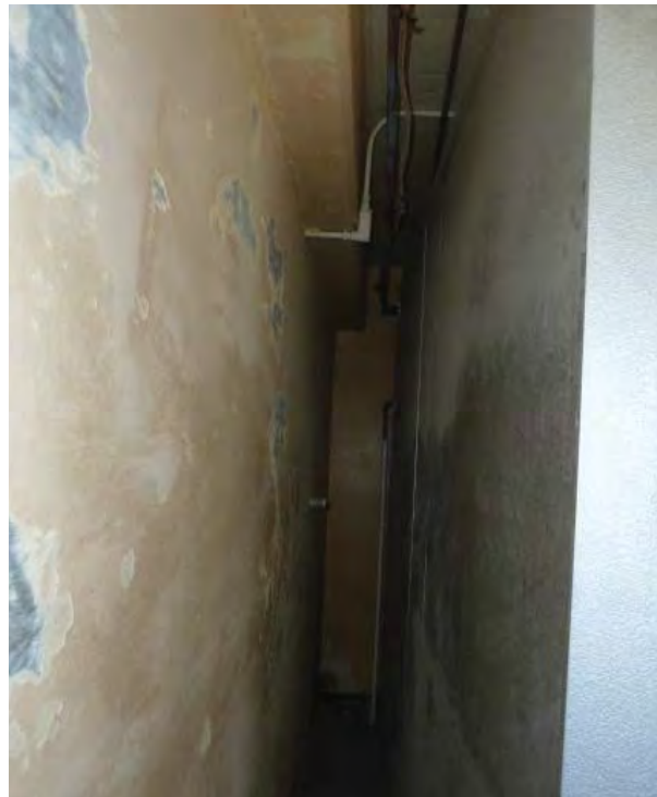
Figure C149. Room 005 - View looking south along side of walk-in cooler.
