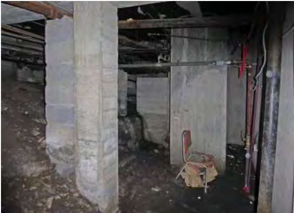
Figure C18. Concrete column in crawl space. CMU column to immediate left is not structural.
