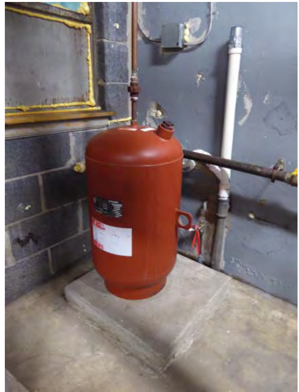
Figure C159. Pressurized tank in northeast corner.
