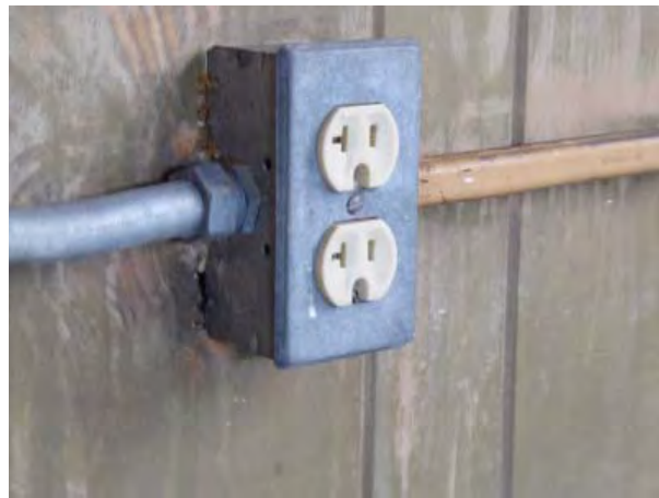
Figure C43. Example of typical surface-mounted receptacle.
