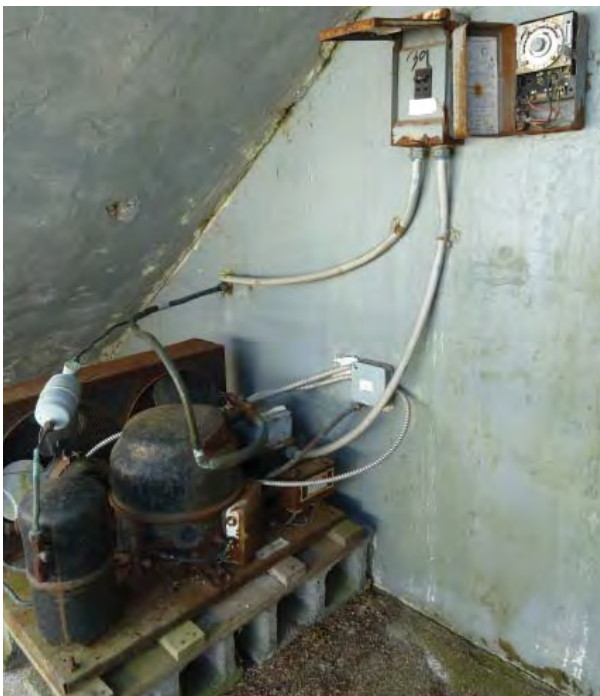
Figure C98. Compressor unit for walk-in cooler on main level (Room 105B).
