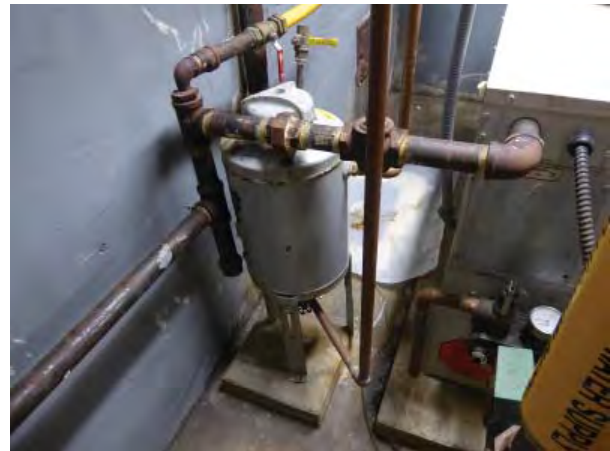
Figure C157. Pressure tank east of boiler.
