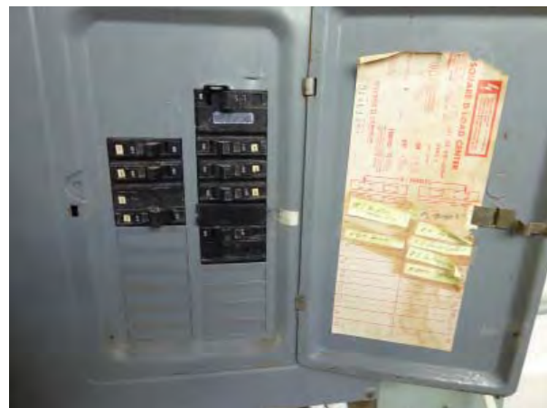
Figure C203. Electrical sub panel beneath east end of serving counter.
