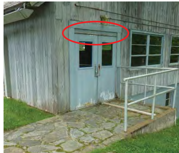
Figure B25. Current flagstone-paved ramp, railing, and replacement steel doors. Blocking at the top of the doorway suggests the height of the original doors. (JKOA, 2018)
