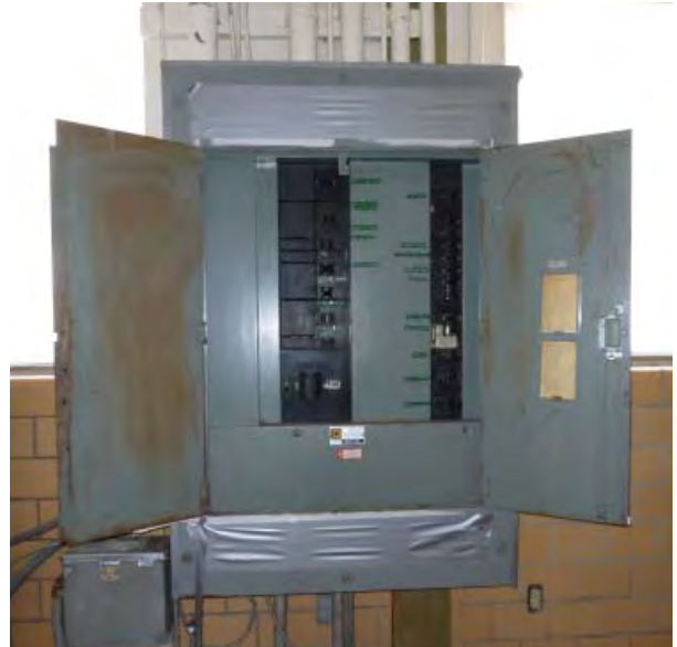
Figure C38. Main electrical panel on north wall of Room 102.
