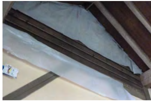
Figure C187. Louvered gable on west wall, partially obscured by plastic.
