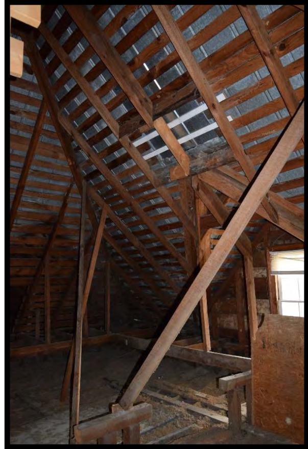
Figure 56: George Hinton House, Location of Removed Chimney Stack.
