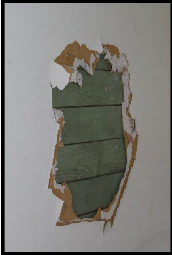
Figure 10: Barnes House, Exposed Flush Boards.
