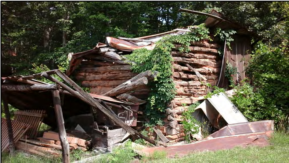
Figure 5.97. Architectural resource RK1682; view is northeast featuring collapsed Tobacco Barn #1.
