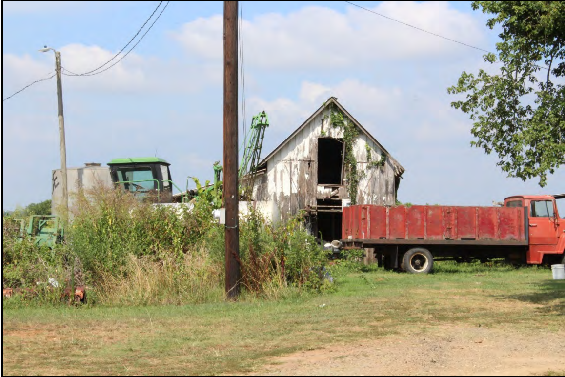
Figure 6.17. Architectural resource AM1522; view is west showing deteriorated storage shed.
