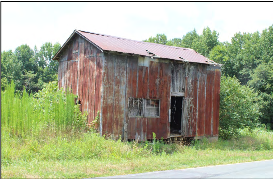
Figure 6.48. Architectural resource AM2499; view is northeast featuring the façade and west elevation.
