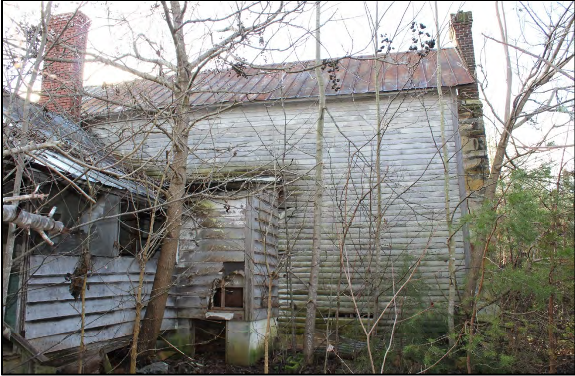
Figure 6.2. Architectural resource AM1520; view is south featuring the north (rear) elevation of the main block and attached ell.
