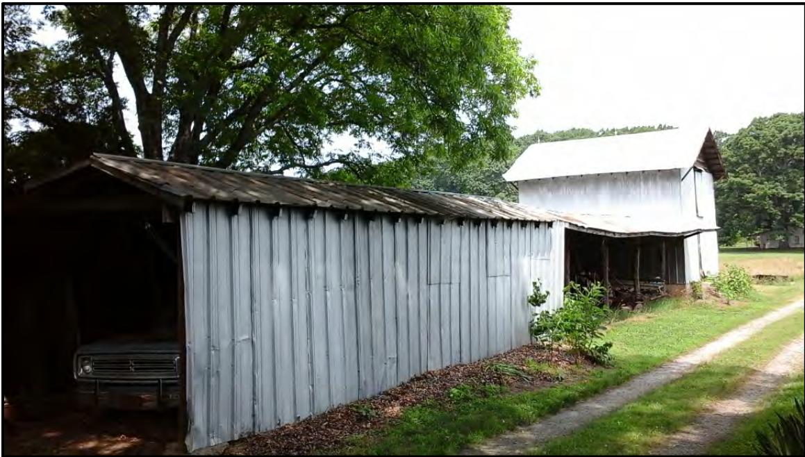
Figure 5.109. Architectural resource RK1684; view is northwest featuring the vehicle and equipment shed connected to the tobacco barn.
