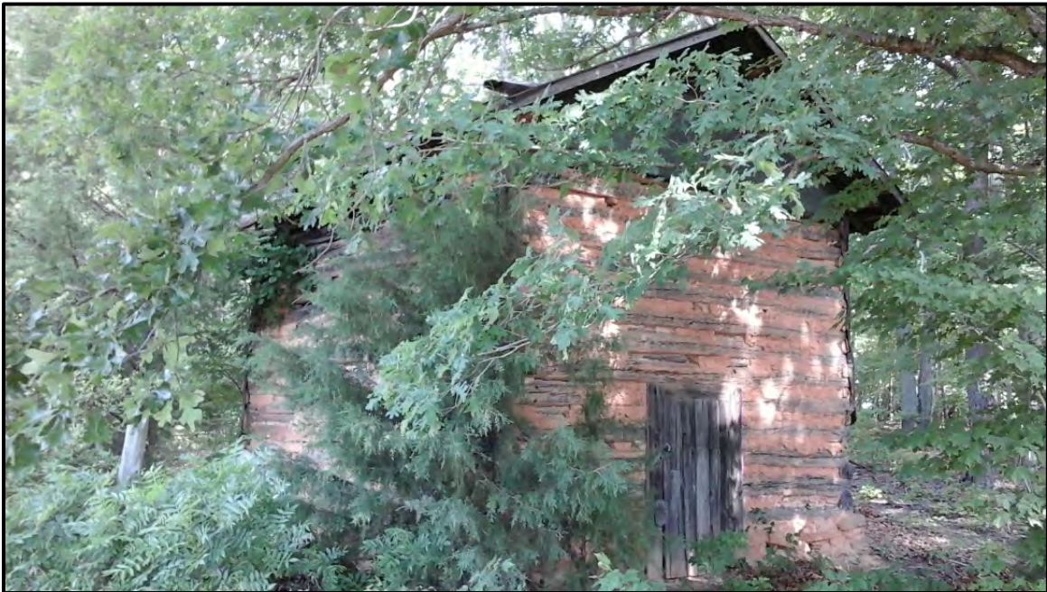
Figure 5.103. Architectural resource RK1682; view is northeast featuring the ca. 1932 gable-front roof tobacco barn.
