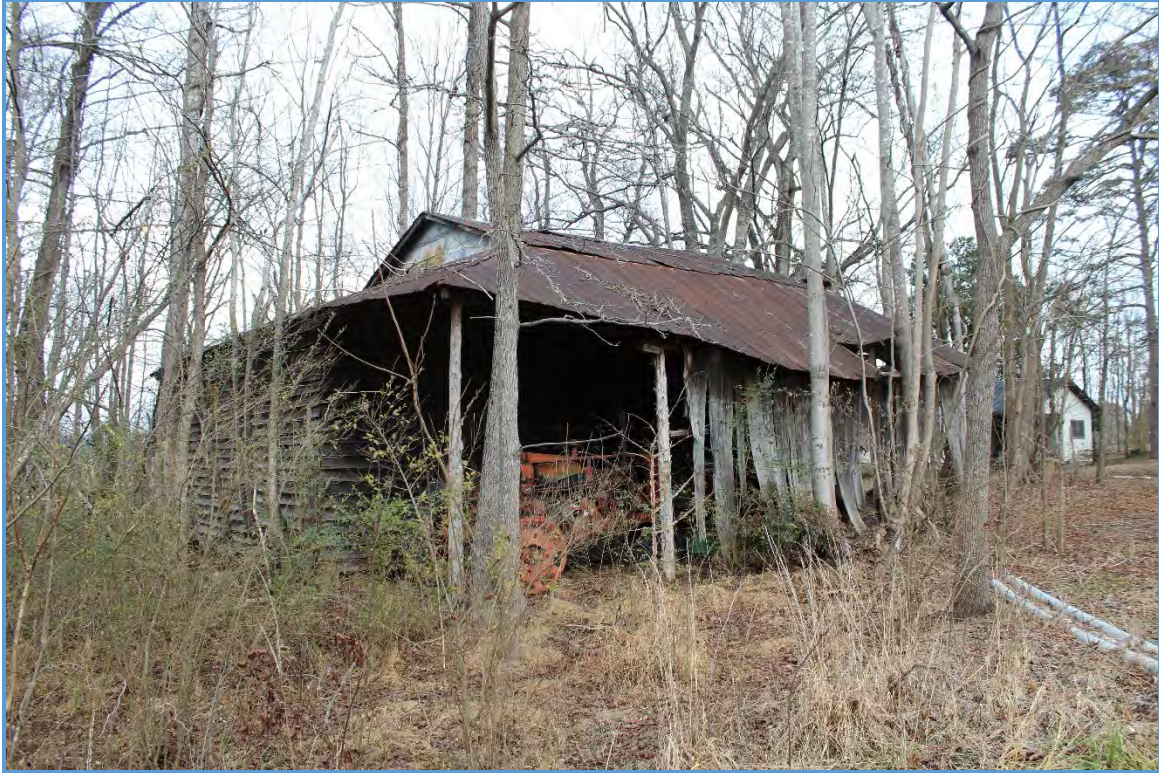
Figure 5.272. RK1758 pack house; view is northeast featuring the northwest and southwest elevations.
