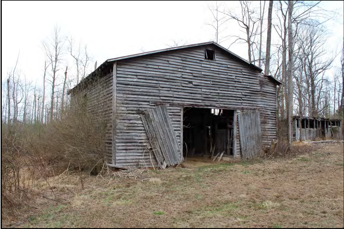
Figure 5.276. RK1758 feed barn; view is northeast featuring the façade and northwest elevation.
