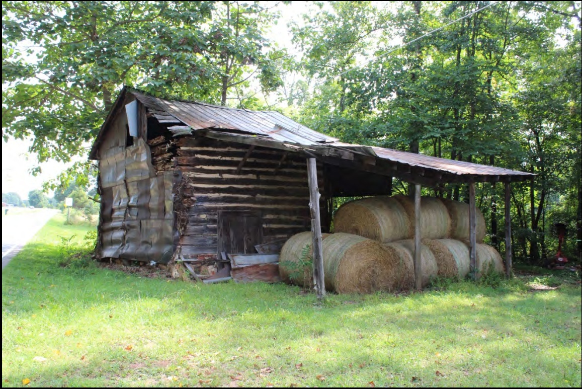
Figure 6.100. Architectural resource AM2516; view is southwest and features the log tobacco barn.
