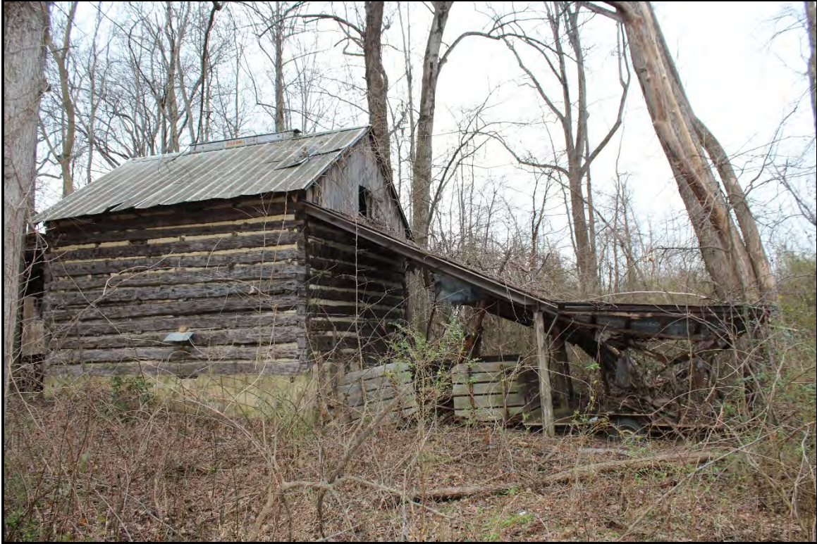
Figure 5.278. RK1758 tobacco barn #1; view is northeast featuring the façade and southwest elevation.
