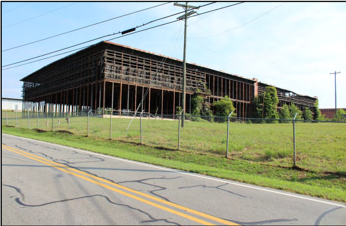
Figure 5.153. Architectural resource RK1704; oblique view northeast toward a partially demolished former warehouse.
