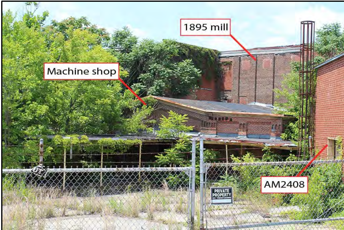
Figure 6.243. Architectural resource AM2407; view is west featuring the northeast corner of mill building and attached machine shop.
