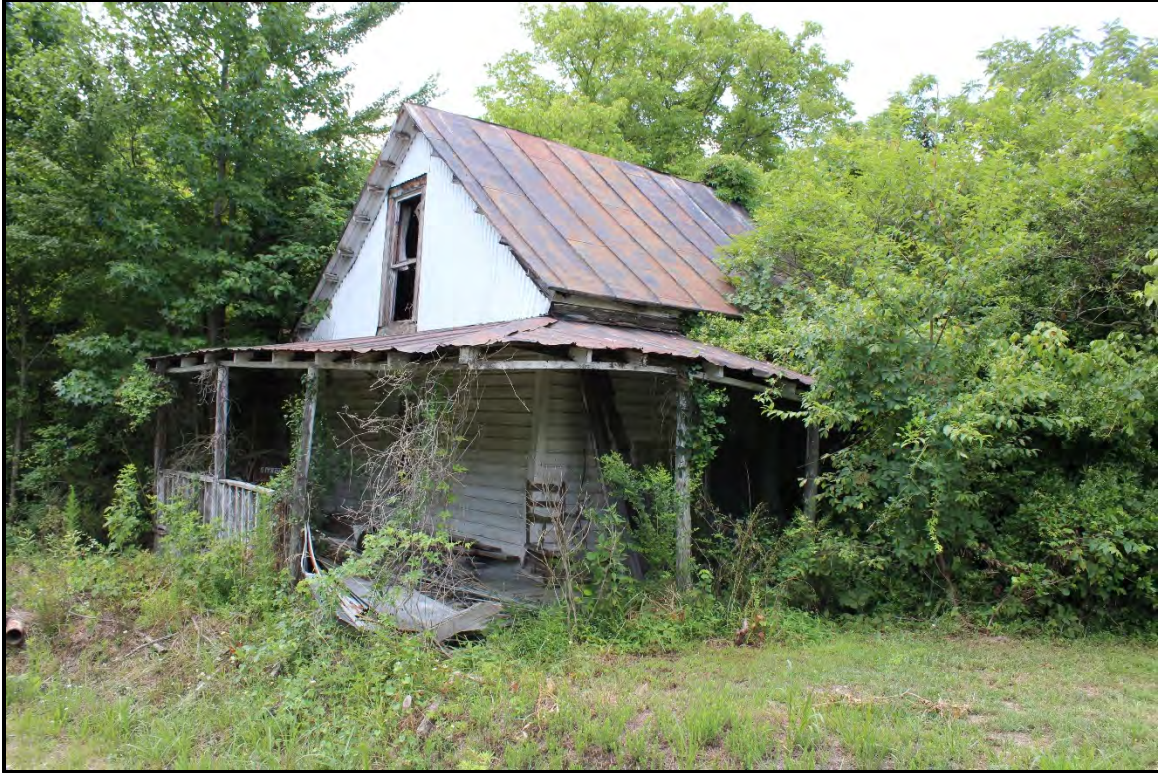
Figure 5.140. Architectural resource RK1701; oblique view south showing the exposed eastern gable end and porch.
