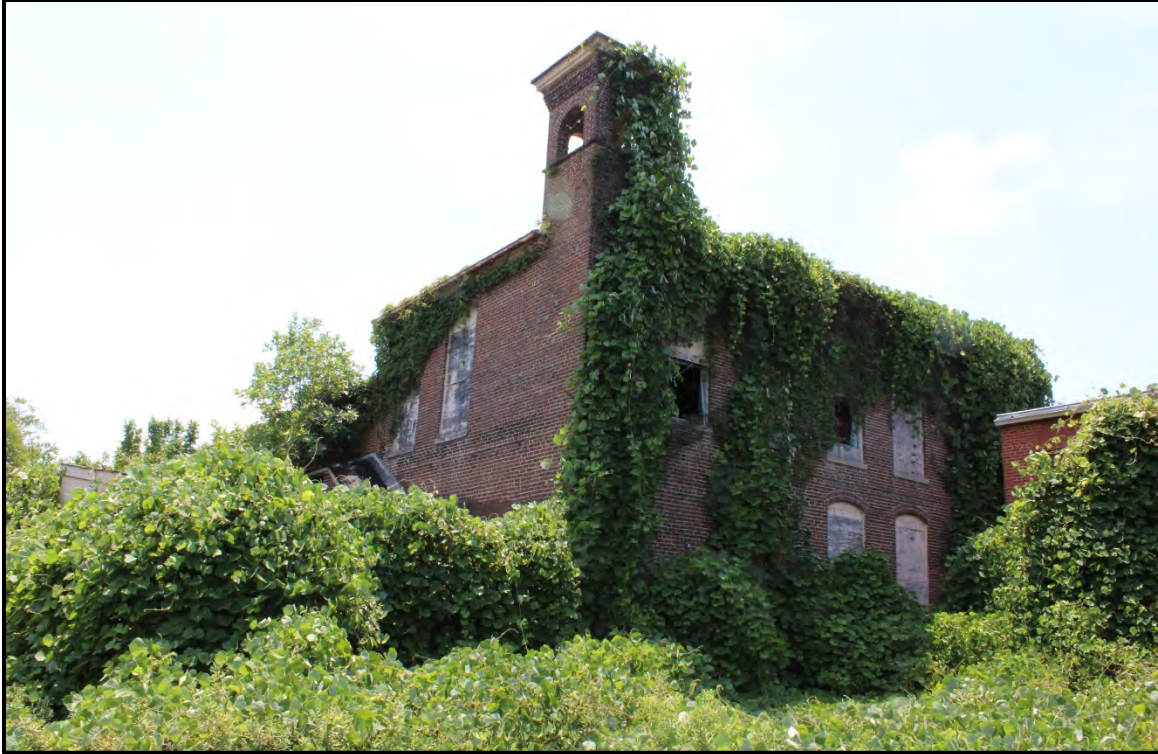
Figure 6.231. T.M. Holt Manufacturing Company; view is southwest featuring the 1892 mill building with the associated stair tower and partially collapsed wall.
