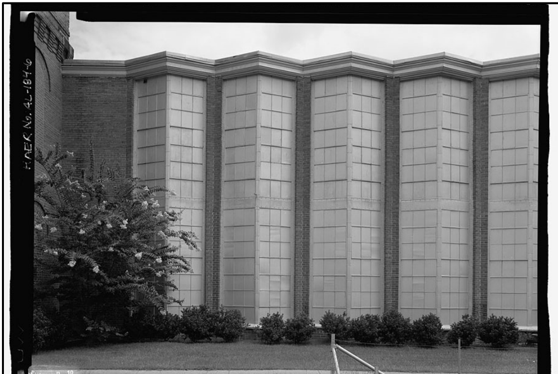
Figure 6.244. Praray windows at the Selma Cotton Mill (image courtesy of the Library of Congress HAER AL-184).
