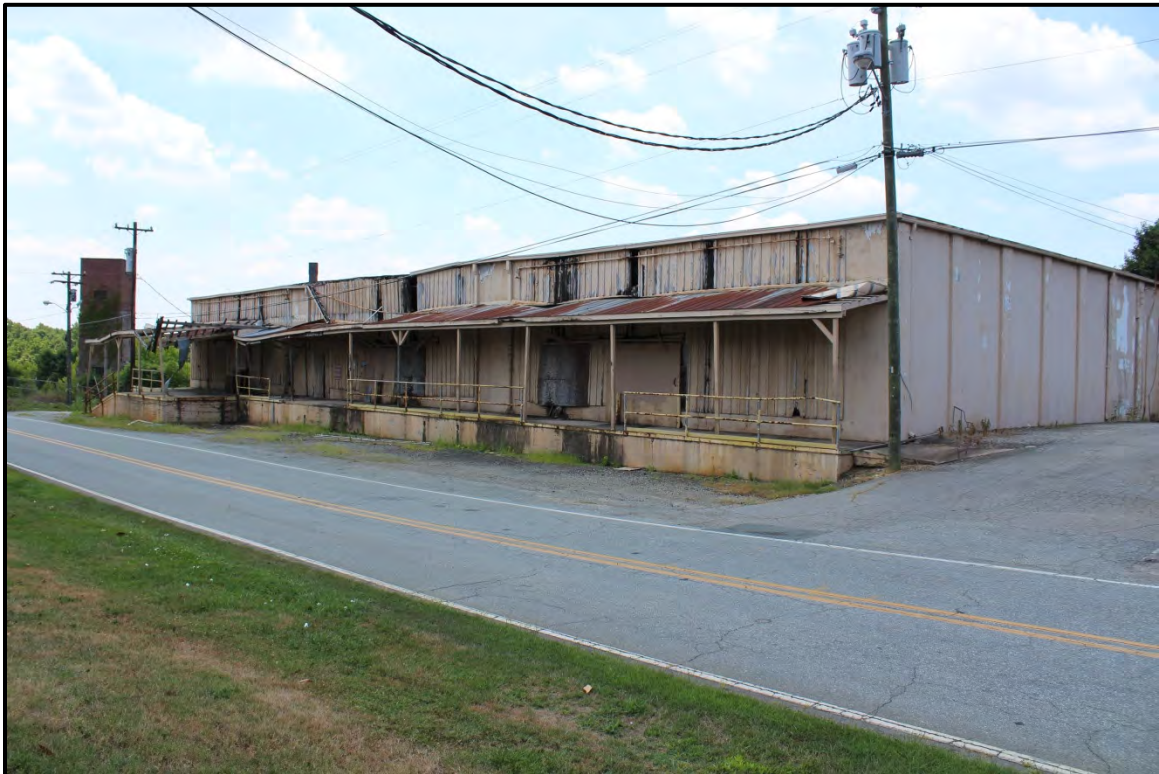
Figure 6.251. Architectural resource AM2408; view is southeast featuring the east and north elevations.
