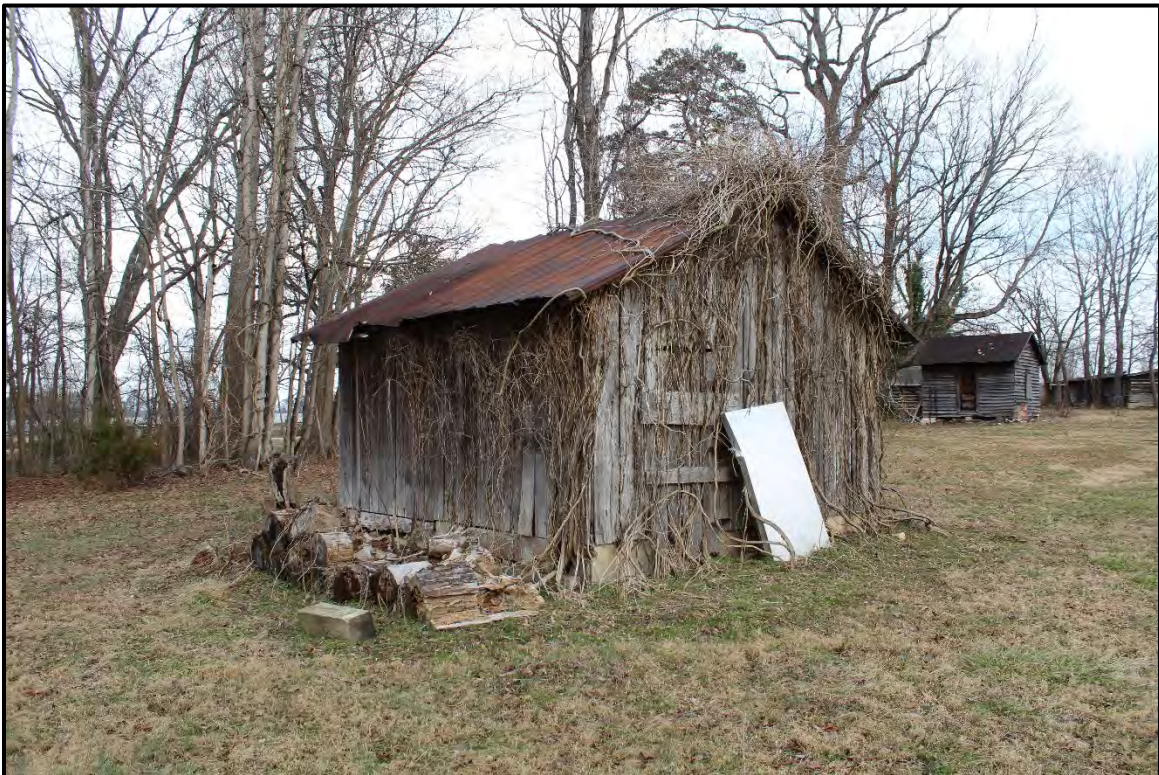
Figure 5.269. RK1758 hog house; view is northeast featuring the south (rear) and west elevation.
