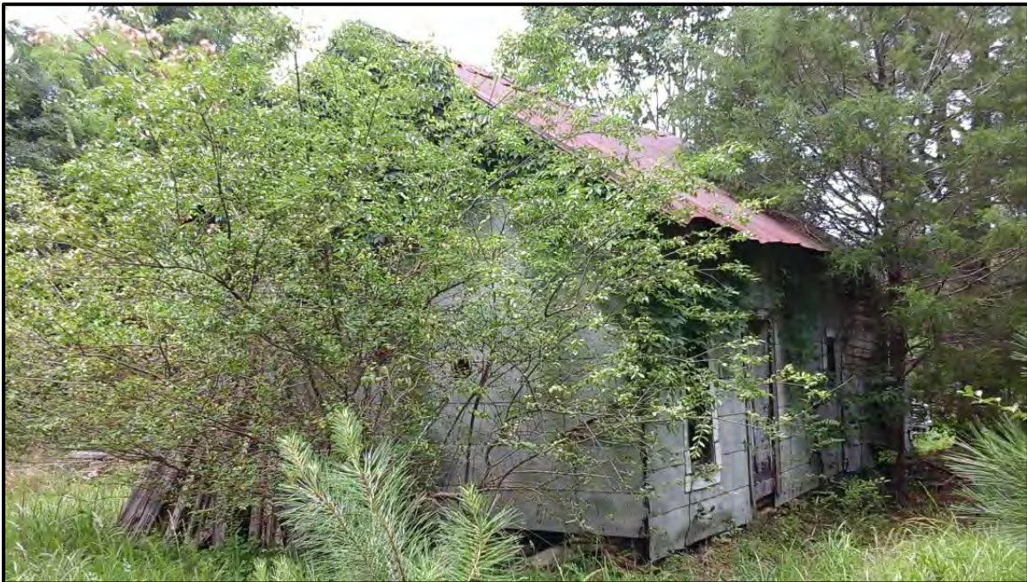
Figure 5.80. Architectural resource RK1678; view is north featuring the façade and south elevation.
