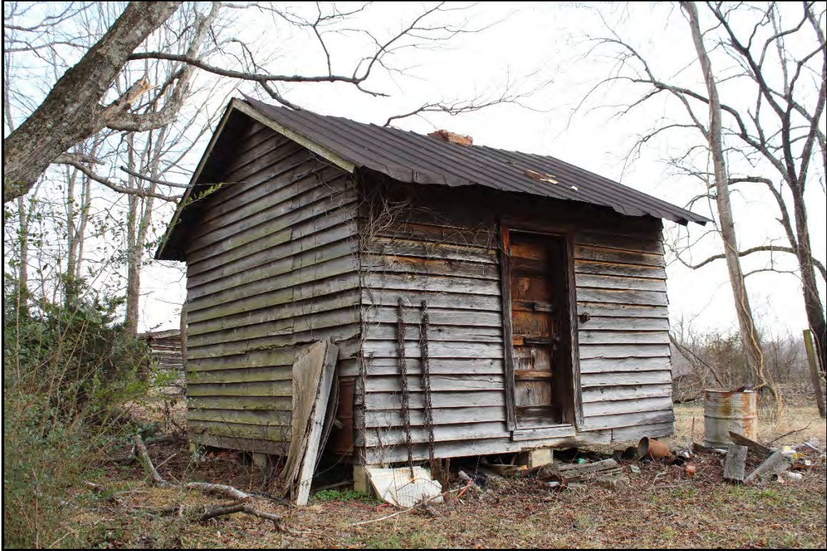
Figure 5.258. RK1758 work shop; view is southeast featuring the façade and north elevation.
