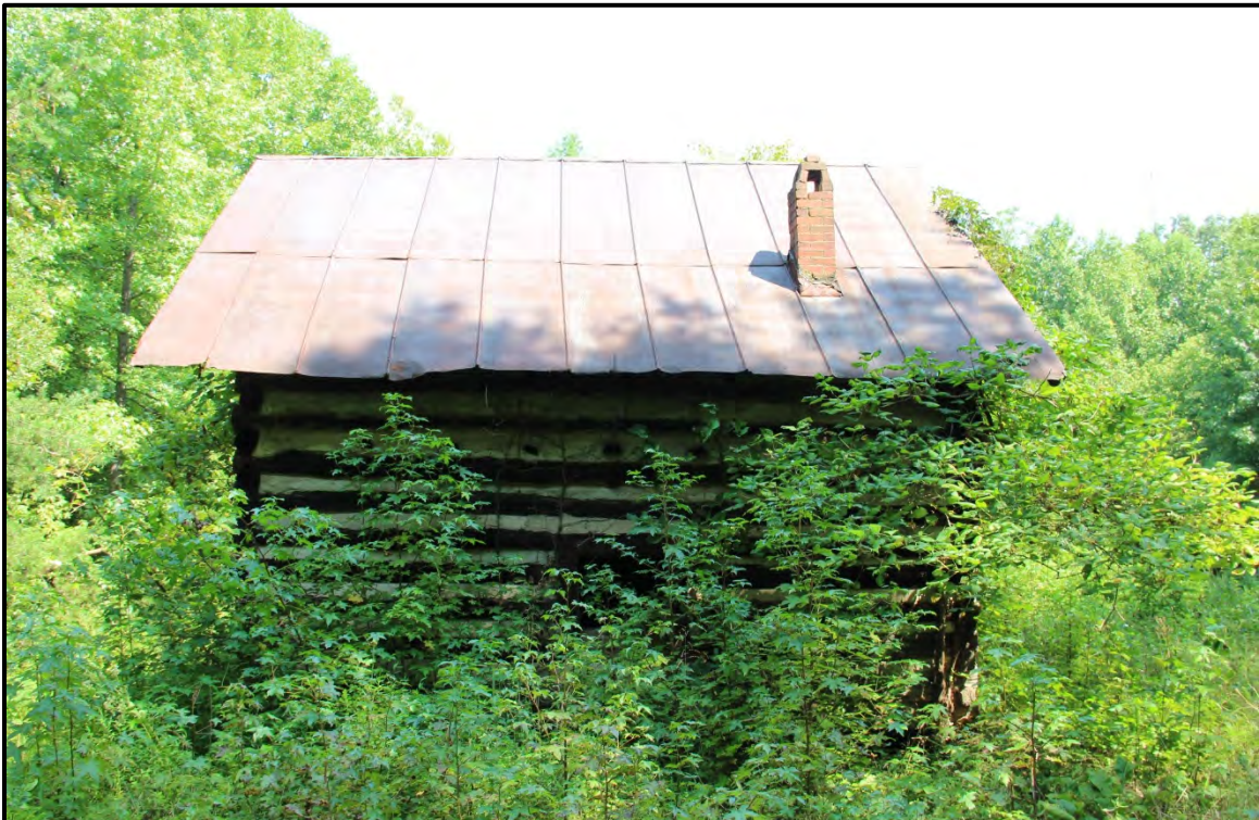
Figure 5.16. Architectural resource RK1656; view is northeast featuring the southwest (rear) elevation of the attached extension.
