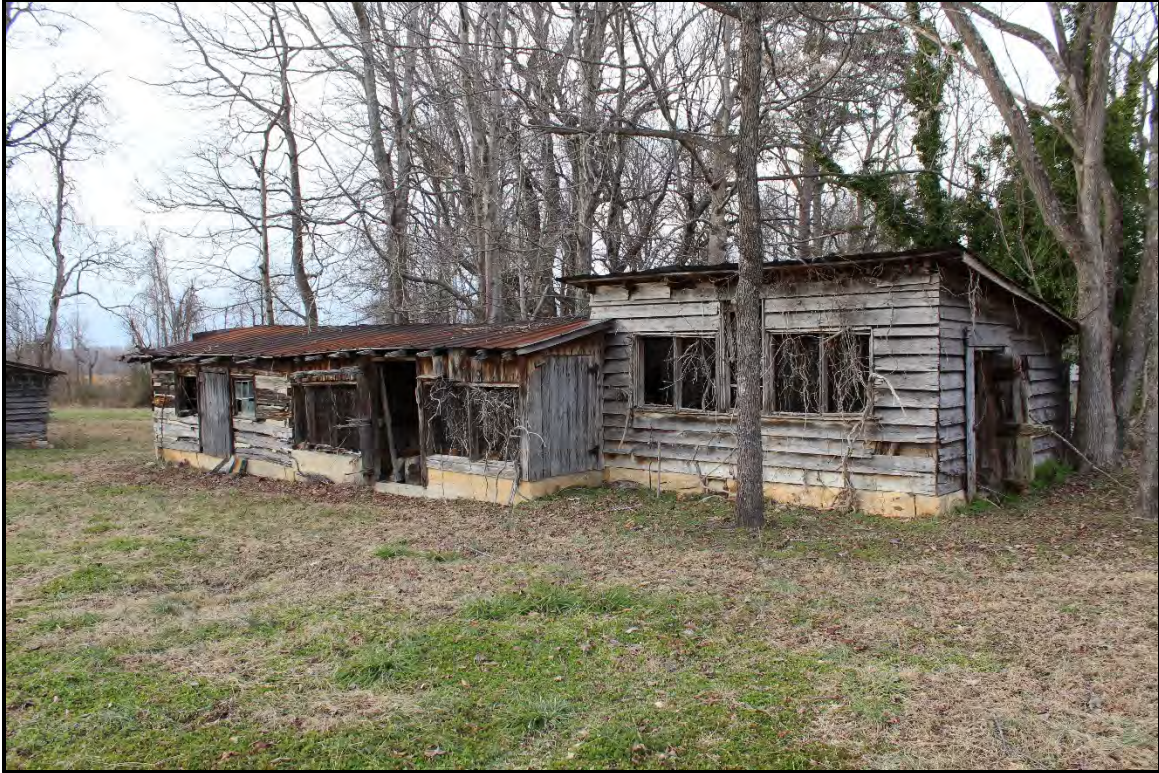
Figure 5.262. RK1758 chicken houses; view is northwest featuring the façade and northeast elevation.
