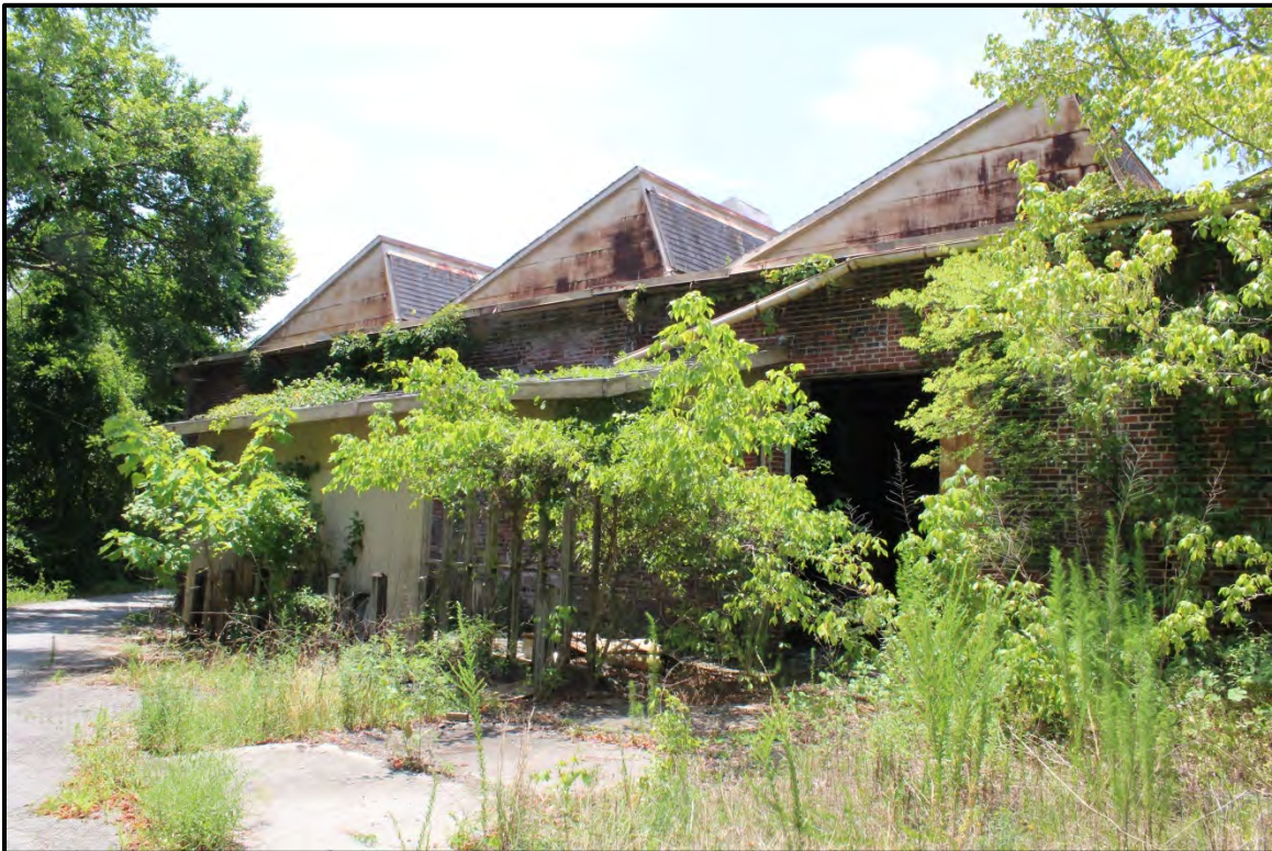
Figure 6.234. T.M. Holt Manufacturing Company; view is southwest featuring the dye house bay topped with saw-tooth roofs.
