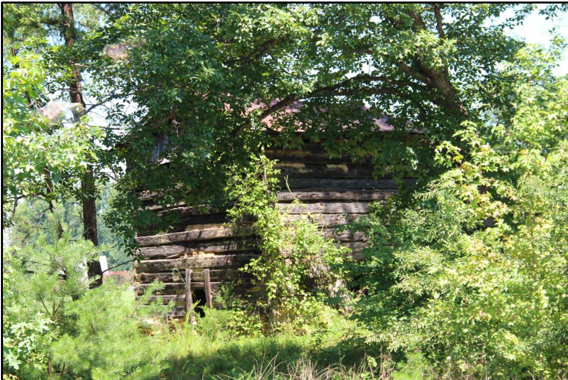
Figure 5.296. Architectural resource RK1760; view is northeast and features the south and west elevations.
