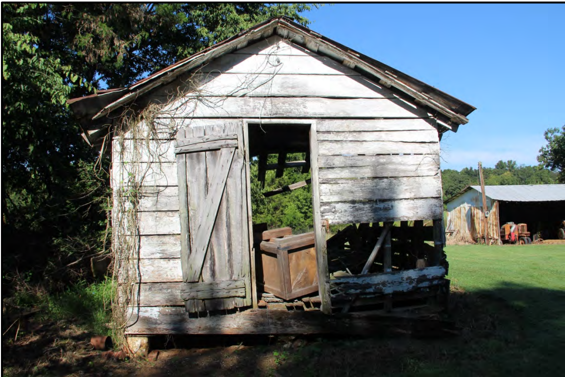
Figure 6.91. Architectural resource AM2514; view is west featuring a partially collapsed storage shed.
