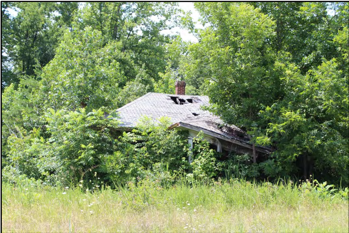
Figure 5.185. Architectural resource RK1724; view is southwest showing collapsed hipped-roofed house overgrown with vegetation.
