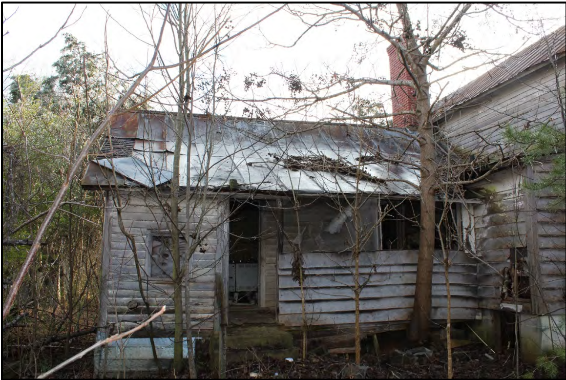
Figure 6.3. Architectural resource AM1520; view is southeast featuring the rear ell and interior brick chimney.
