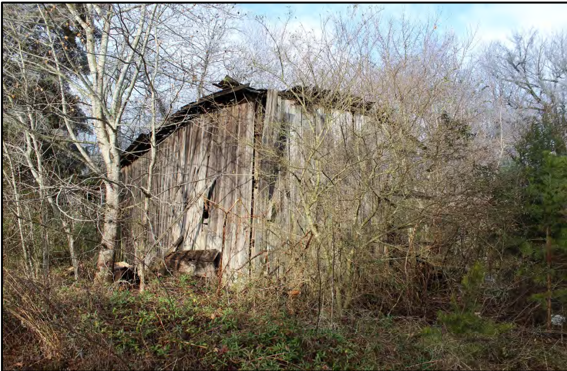
Figure 6.11. Architectural resource AM1520; view is north featuring the southeast corner of the collapsed outbuilding near Troxler Mill Road.
