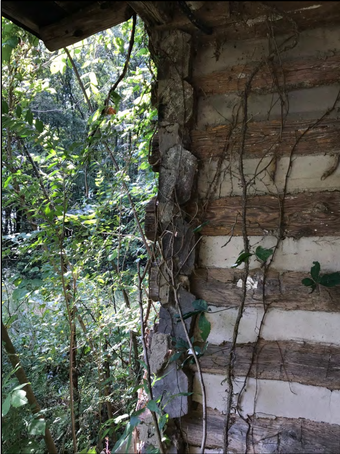
Figure 5.12. Architectural resource RK1656; view is north featuring v-notching at the southwest corner of the main block.
