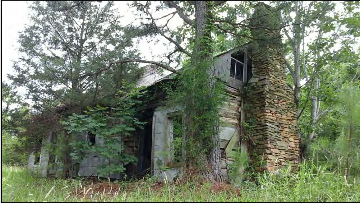
Figure 5.79. Architectural resource RK1678; view is south featuring the façade and north elevation.
