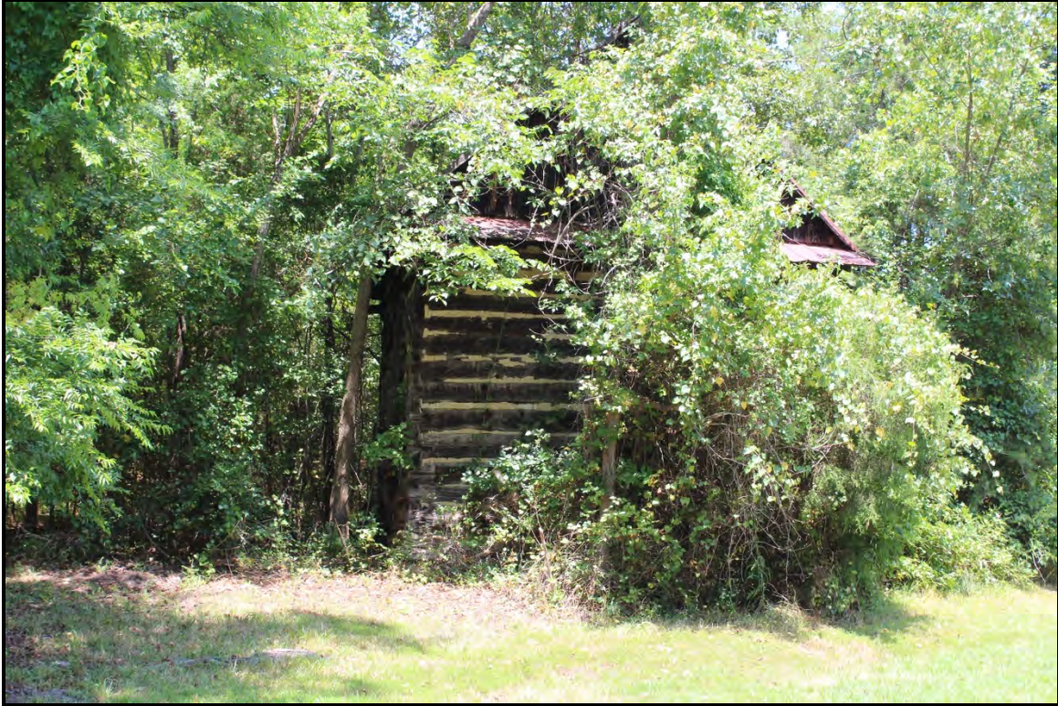
Figure 6.138. Architectural resource AM0122; view is north featuring the early-twentieth century tobacco barn.
