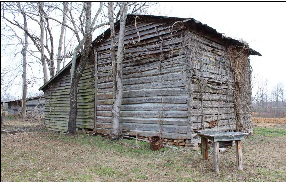
Figure 5.267. RK1758 granary and tractor shed; view is southeast featuring the northwest (rear) and southwest elevation.
