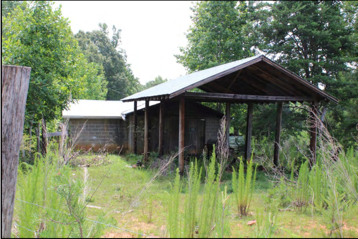
Figure 5.60. Architectural resource RK1668; view is southeast featuring the primary façade and attached pole shed.
