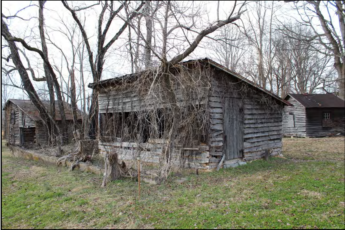
Figure 5.264. RK1758 dog kennel; view is northwest featuring the façade and northeast elevation.
