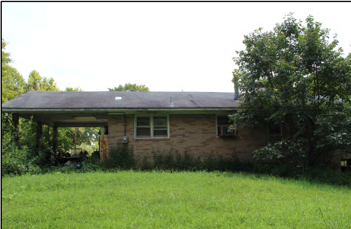
Figure 5.246. Architectural resource RK1753; view is southeast and features the northwest (rear) elevation.
