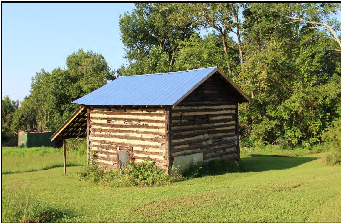
Figure 5.221. Architectural resource RK1744; view is southwest and features the north and east elevations.
