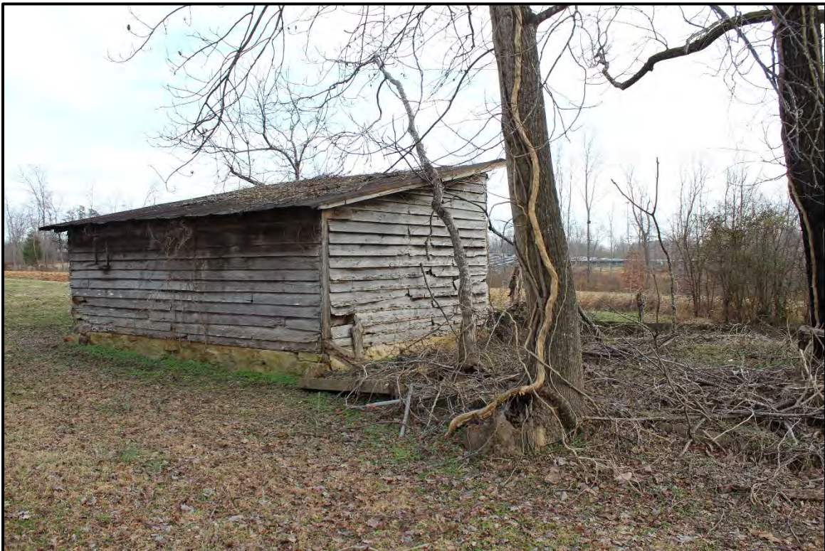
Figure 5.265. RK1758 dog kennel; view is southeast featuring the northwest (rear) and southwest elevations.
