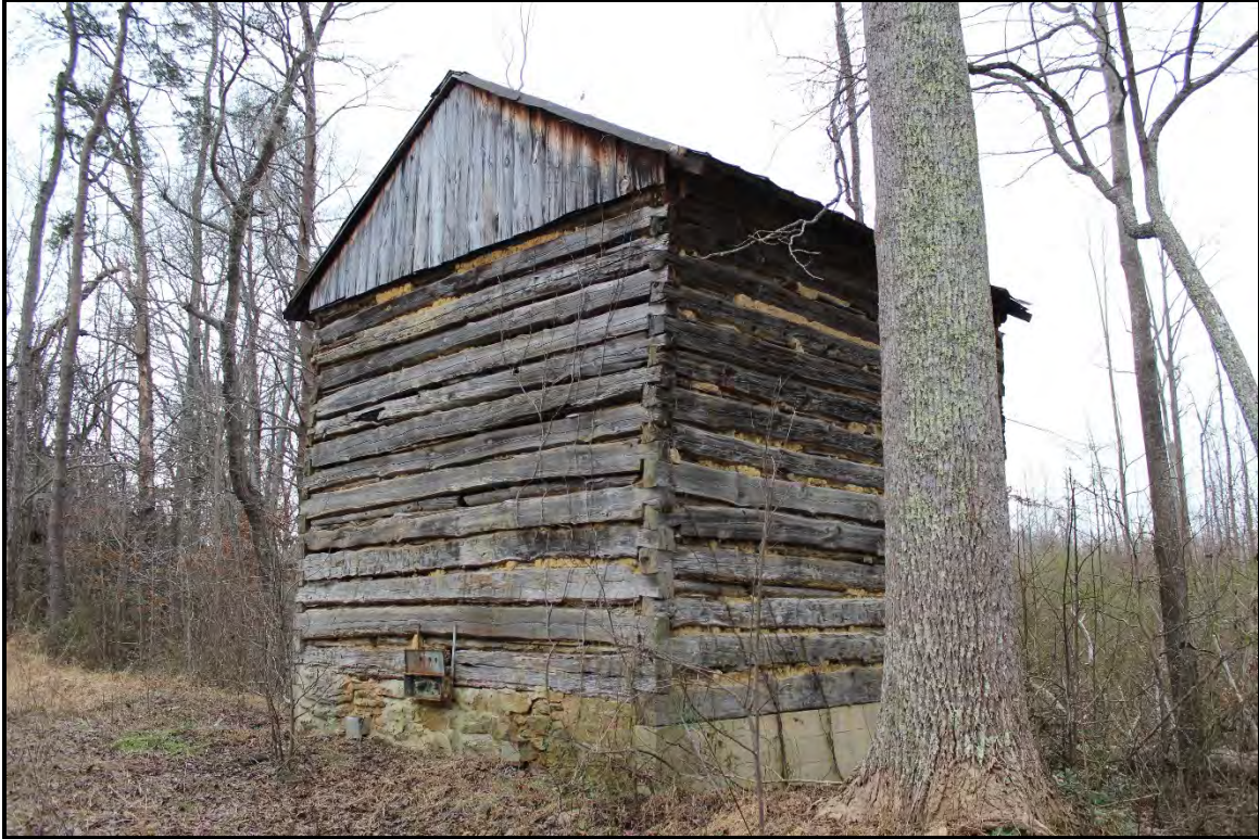
Figure 5.282. RK1758 tobacco barn #3; view is southeast featuring the northeast and northwest elevations.
