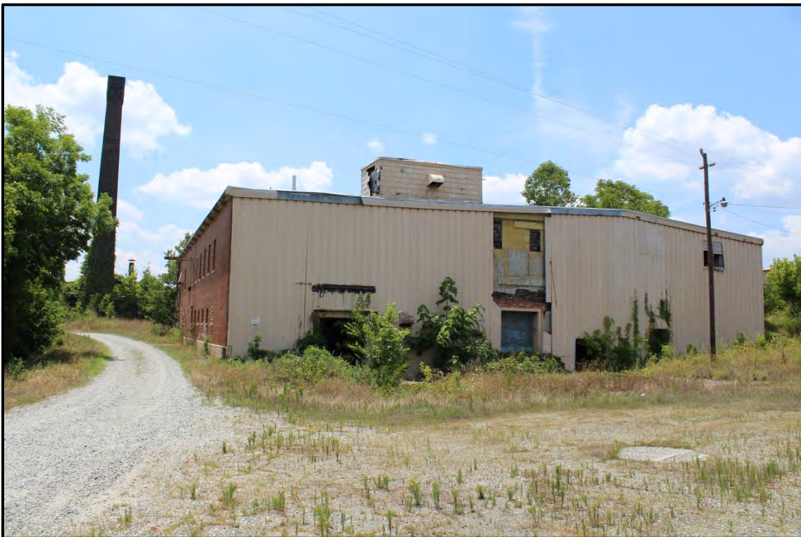
Figure 6.236. T.M. Holt Manufacturing Company; view is southwest featuring the north elevation of the ca. 1934 Holt-Tabardrey Mill (AM1516)
