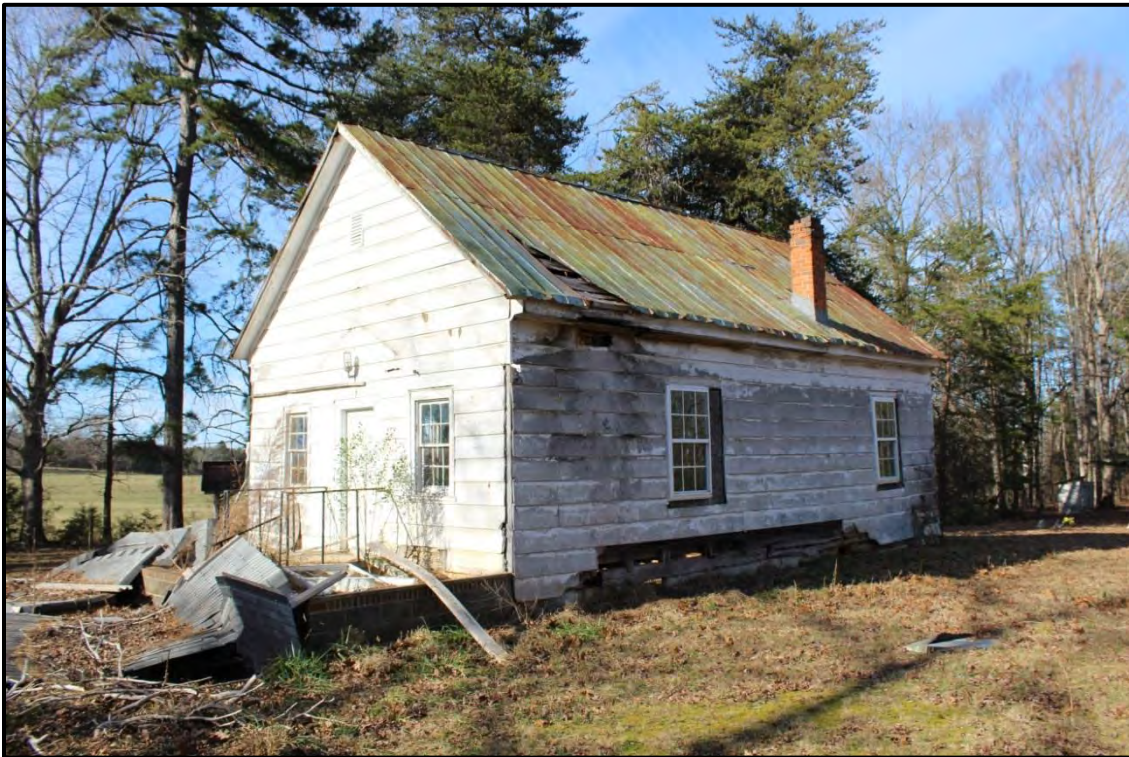
Figure 4.61. Architectural resource AM1603; view is northwest featuring the façade and east elevation.
