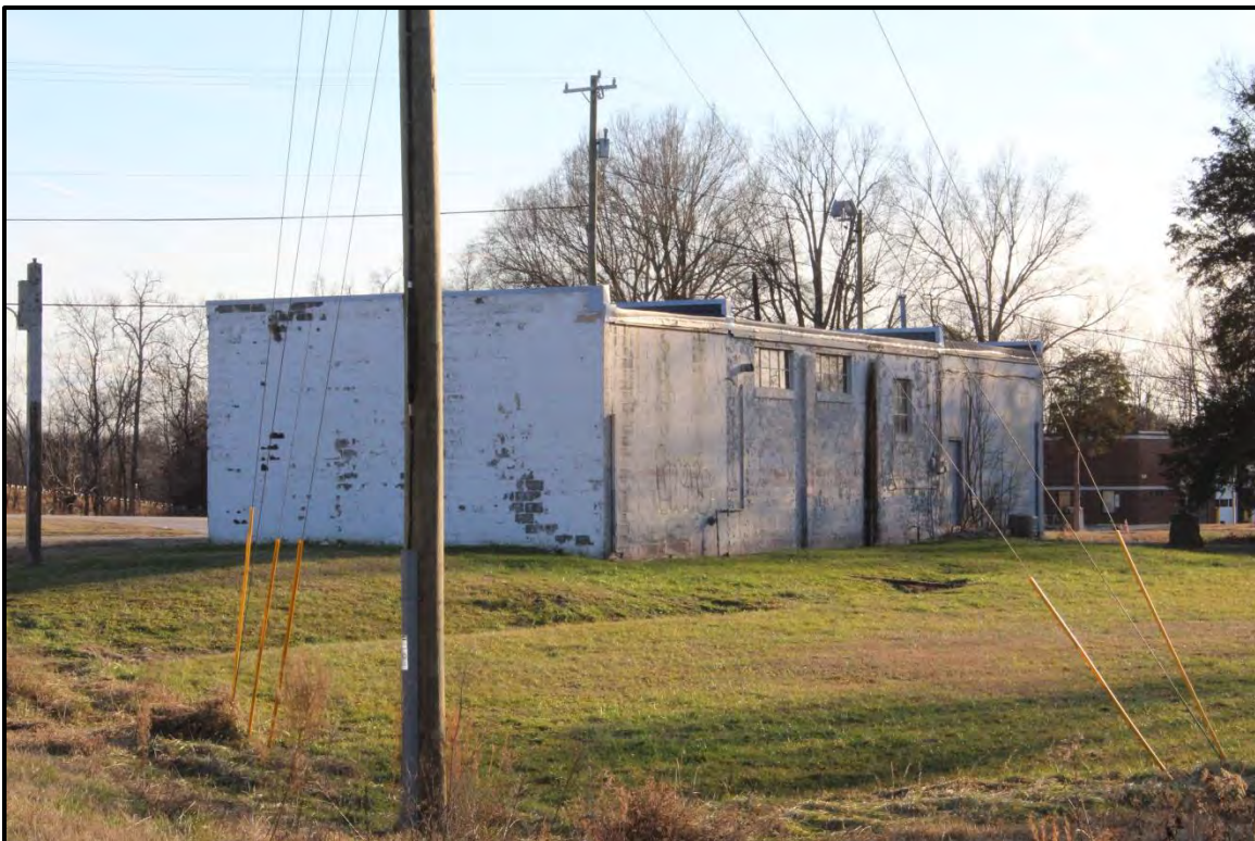
Figure 3.6. Architectural resource GF9108; view is northwest featuring the south (rear) and east elevations.
