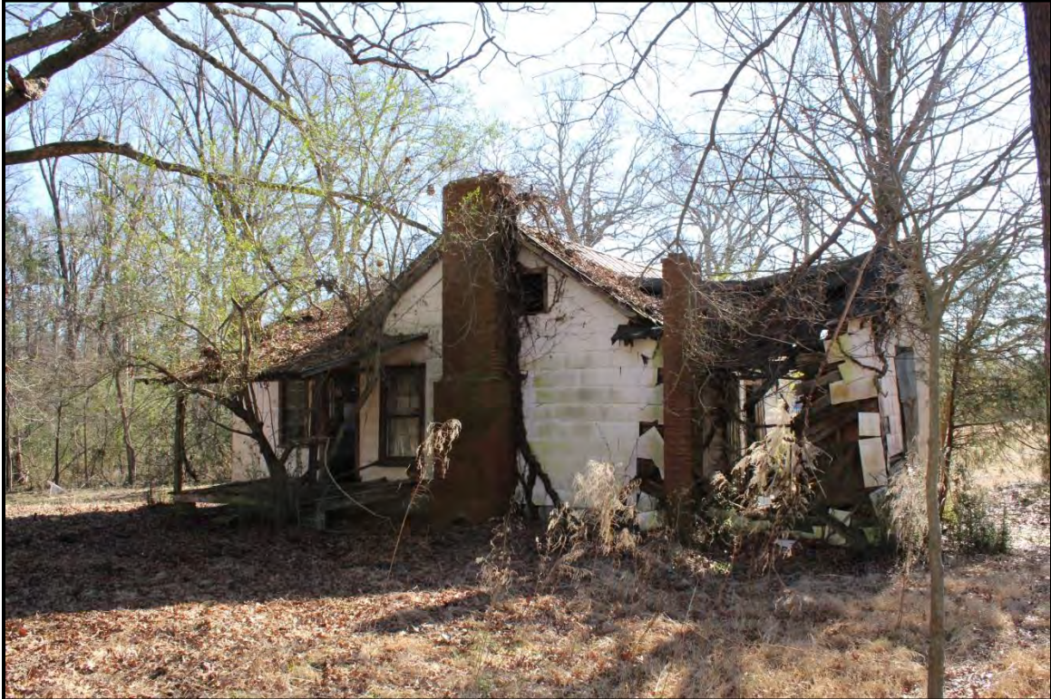
Figure 4.104. Architectural resource AM2632; view is south featuring the partial collapse of the north elevation.
