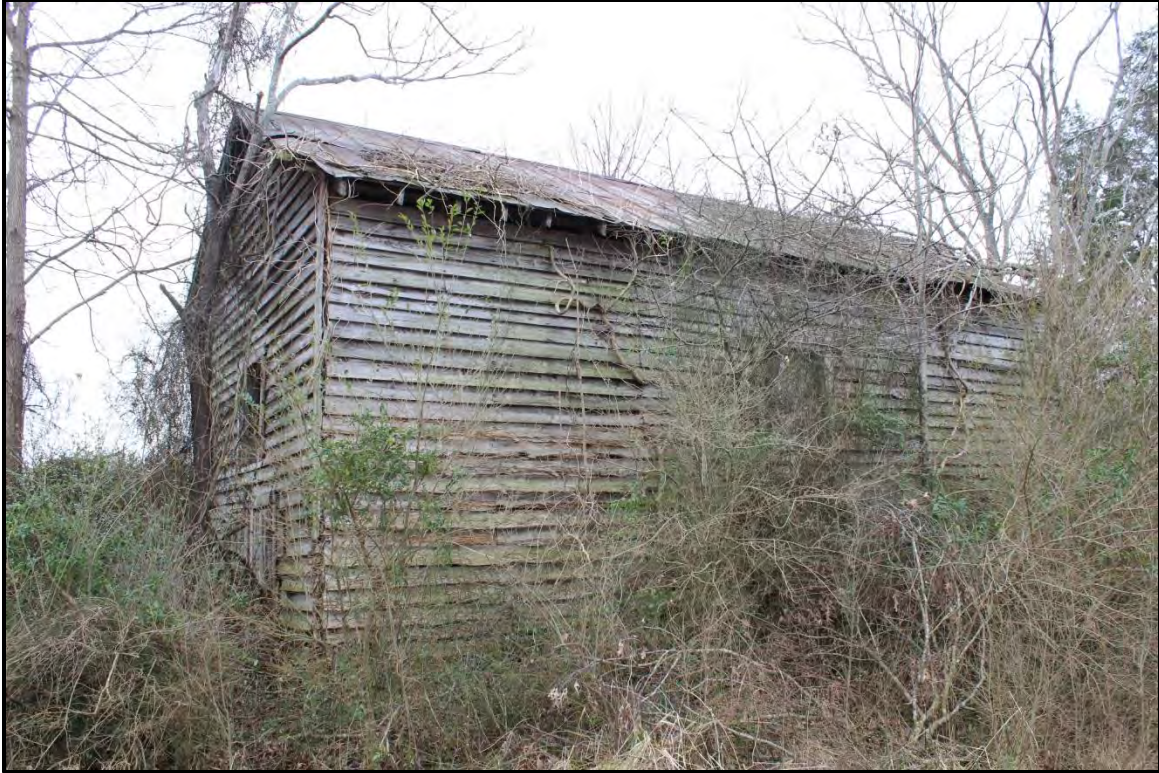
Figure 2.89. Architectural resource RK1818; view is west featuring the early twentieth century equipment/workshop building.
