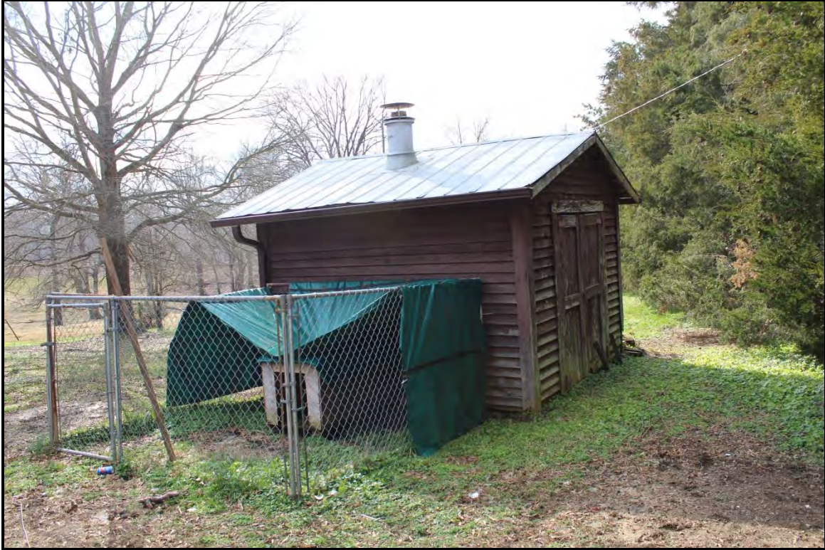
Figure 2.63. Architectural resource RK1820; view is east and features the ca. 1985 storage shed.
