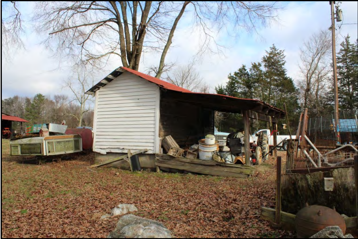
Figure 4.86. Architectural resource AM2631; view is northeast featuring the west (rear) of the single-bay garage and the open shed-roof extension attached to the south elevation.
