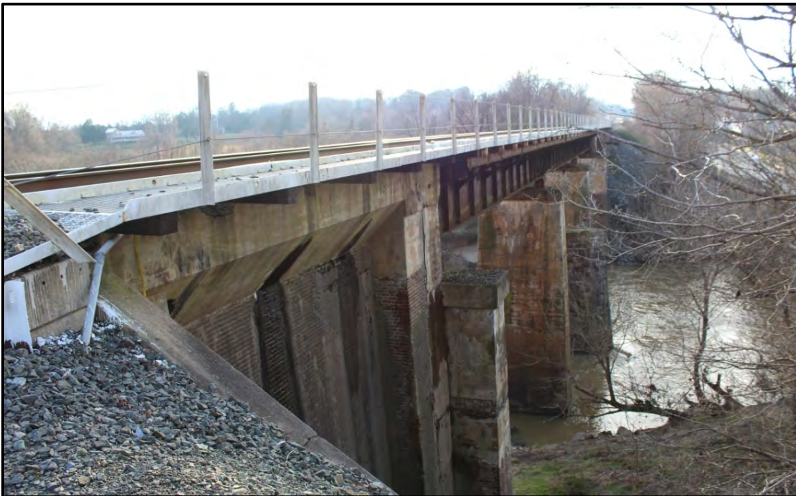
Figure 4.153. Architectural resource AM1324; view is northeast featuring the south elevation of the bridge with the attached walkway.
