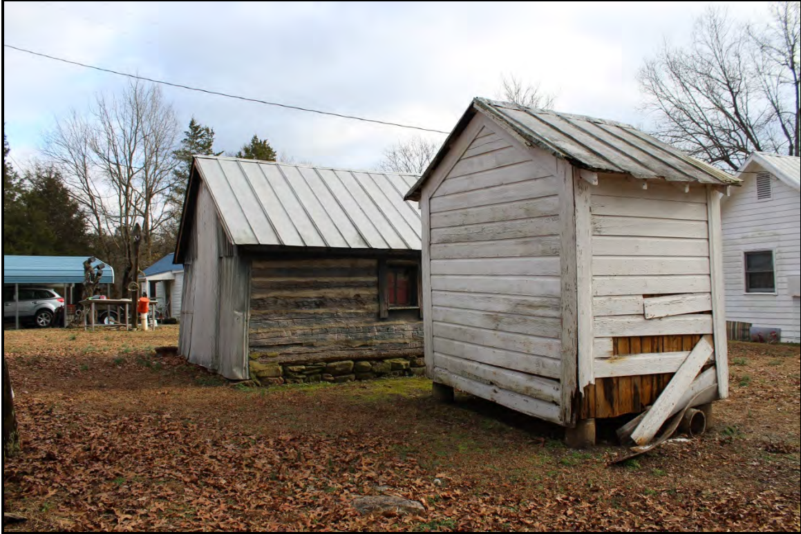
Figure 4.84. Architectural resource AM2631; view is southeast featuring the north (rear) and east elevations of the ca. 1900 log kitchen and adjacent mid-twentieth century shed.
