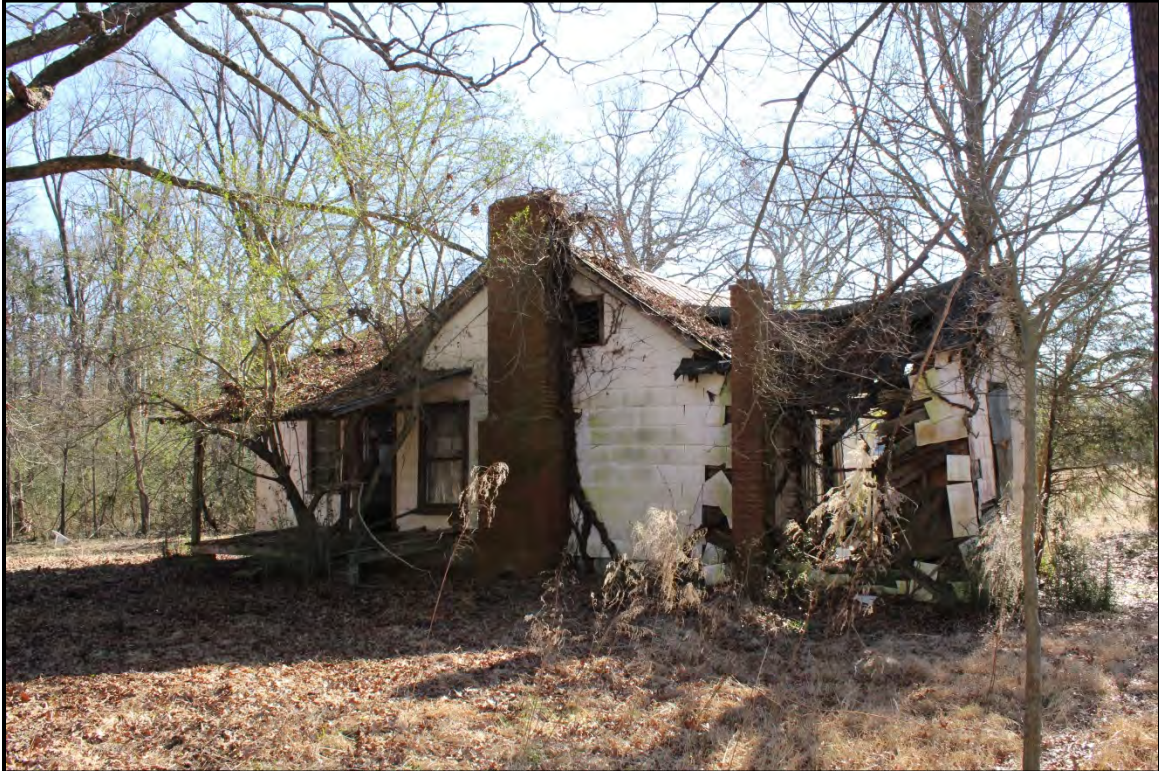
Figure 4.104. Architectural resource AM2632; view is south featuring the partial collapse of the north elevation.
