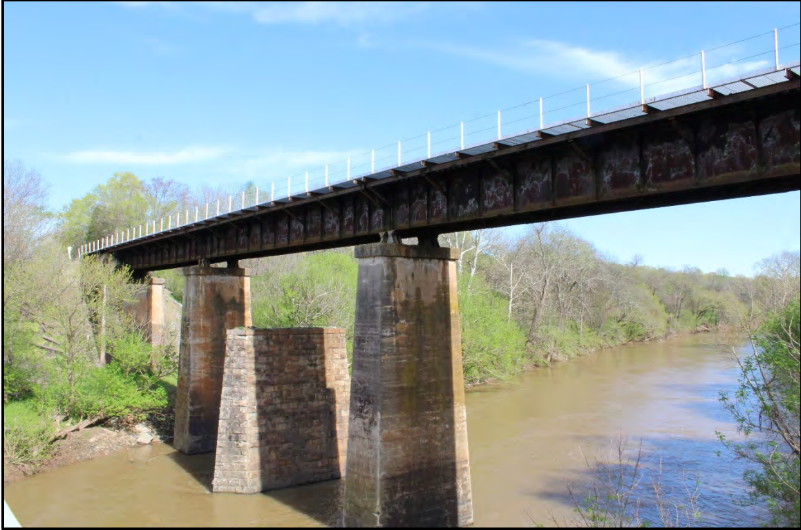
Figure 4.154. Architectural resource AM1324; view is east featuring the north elevation of the bridge.
