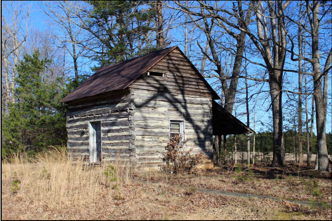
Figure 4.32. Architectural resource AM0209; view is northeast featuring the façade and south elevation with non-historic window sash.
