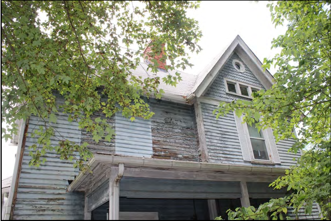
Figure 3.15. Architectural resource AM0447; detail view of former location of second story porch on east elevation. Note modern beaded board siding where the door was once located.
