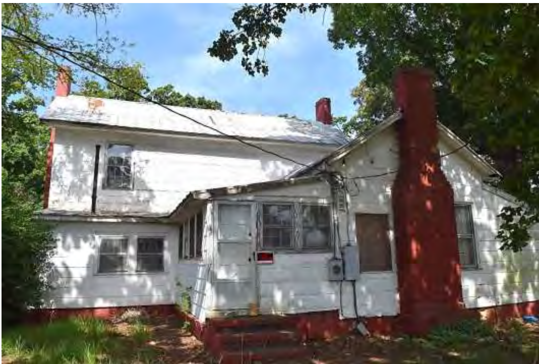
Alexander Farm, Alexander House, Rear (East) Elevation and Rear Ell, Looking West.
