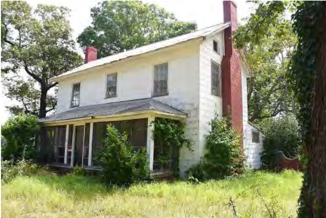
Alexander Farm, Alexander House, Façade (West Elevation) and Side (South) Elevation, Looking Northeast.
