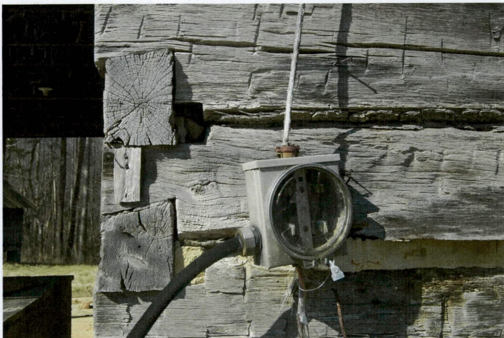
Clapp Family Log House, Detail of Half-Dovetail Notching on Side (East) Elevation.
