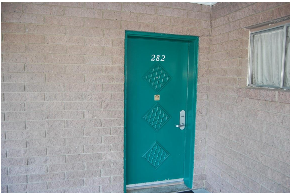
Plate 62. Ambassador Motel and Pancake House Restaurant, Detail of Original Door and Window.
