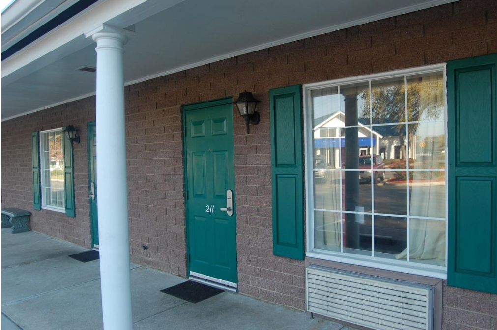
Plate 61. Ambassador Motel and Pancake House Restaurant, Room Door and Window Detail, Looking South.
