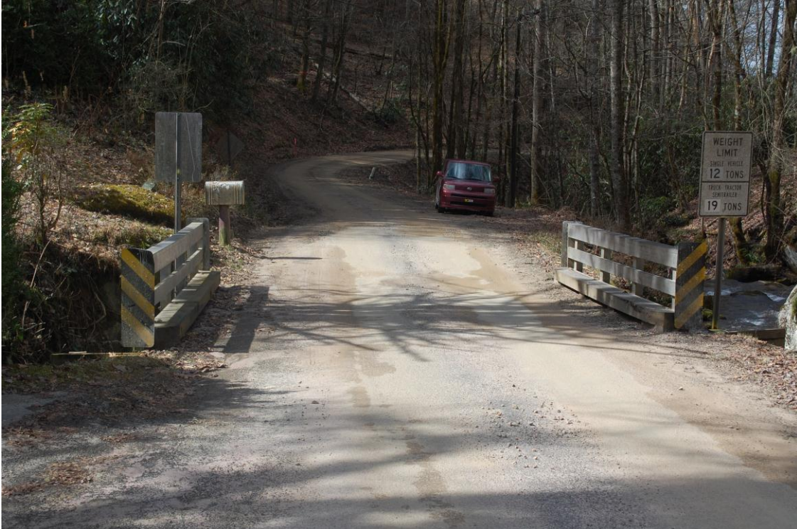
Figure 4: View to the south-southwest toward Bridge No. 192 along Little Ellijay Road. Vida and H. Roy Ahlgrim House is to the left
