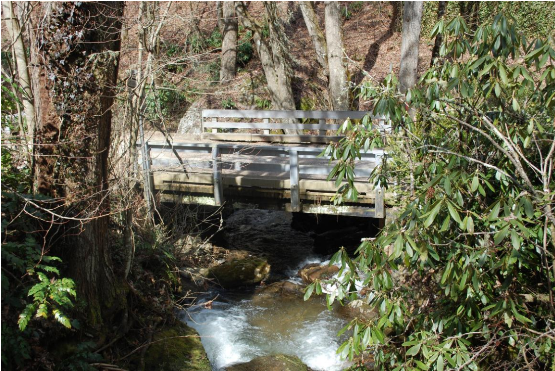
Figure 3: View of Indian Camp Branch and Bridge No. 192, view to the northwest
