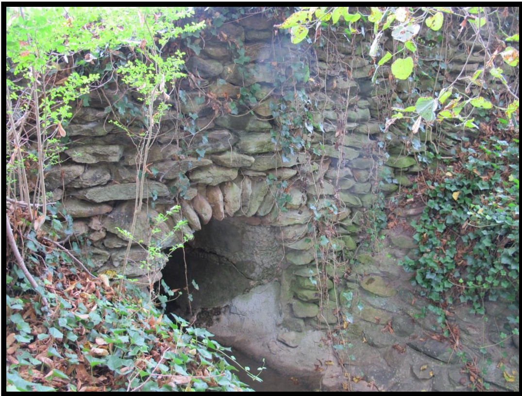
Figure 5: Detail of Stone-Faced Headwall and Culvert for Channelized Section of Unnamed Tributary of Michael Branch, Looking Southeast.
