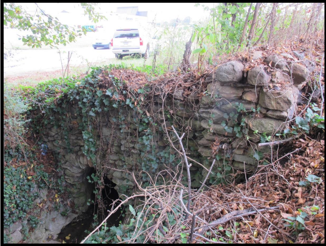
Figure 7: View of Channelized Section of Unnamed Tributary of Michael Branch and Stone-Faced Headwall, Looking East.
