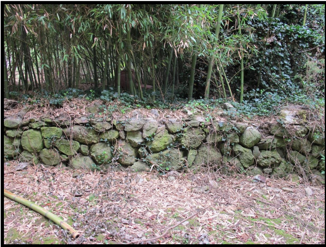
Figure 30: View of Stone Retaining at the Site of the Superintendent's House Looking West.
