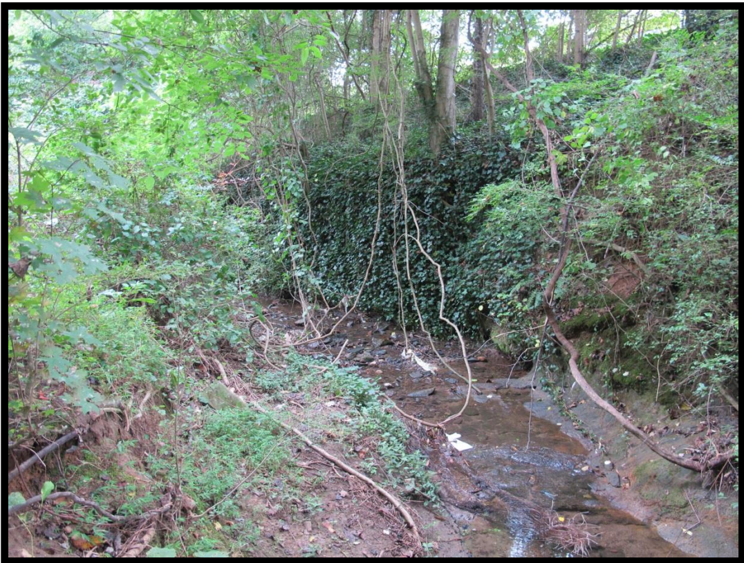
Figure 10: View of Natural Section of Unnamed Tributary of Michael Branch, Looking East.
