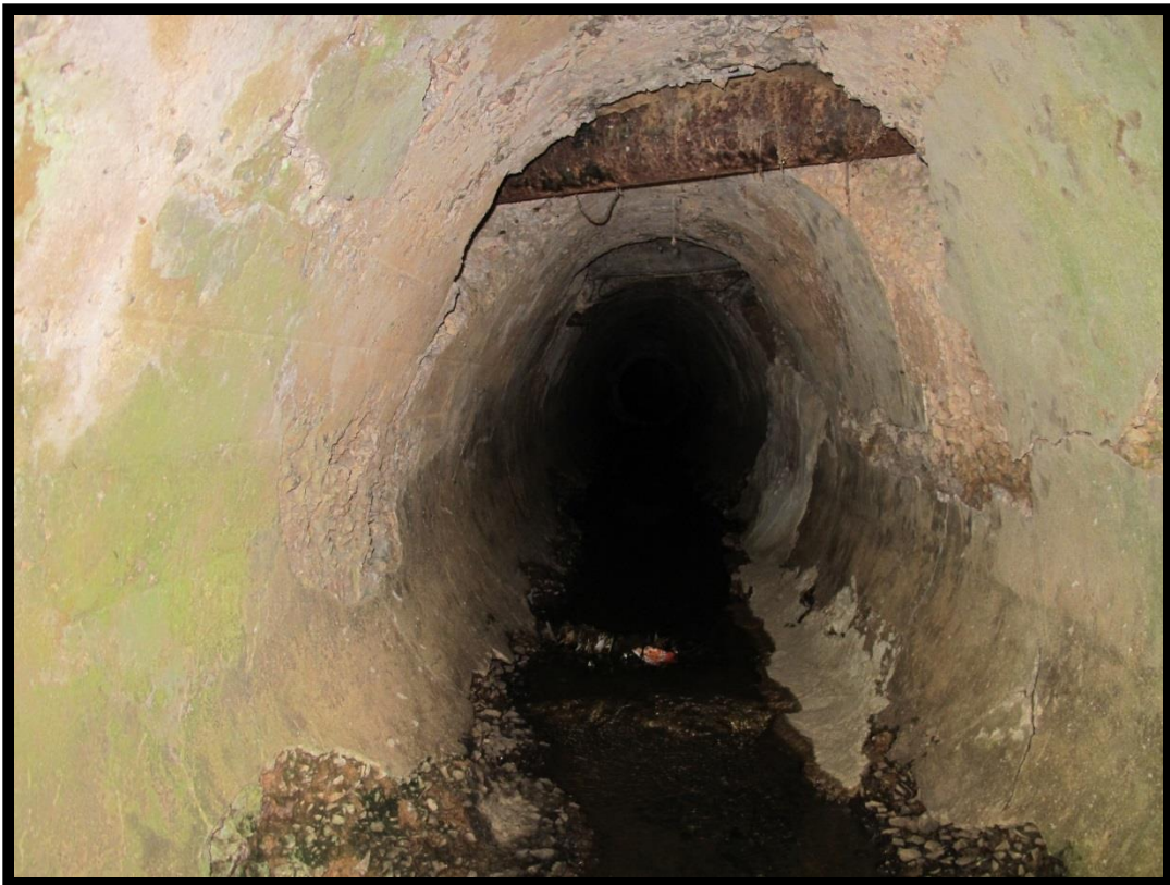
Figure 6: View of Interior of Concrete Culvert for Unnamed Tributary of Michael Branch, Looking East.
