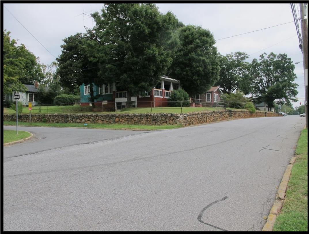
Figure 26: View of Stone Retaining Wall on the Corner of Fifth Street (now Ninth Street) and Broad Street, Looking Northeast.
