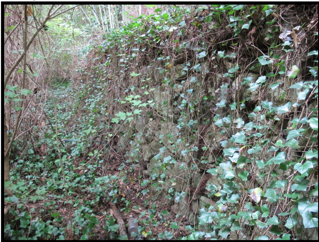
Figure 31: View of Stone Retaining at the Site of the Superintendent's House, Facing the Erlanger Mill Village, Looking Southeast.
