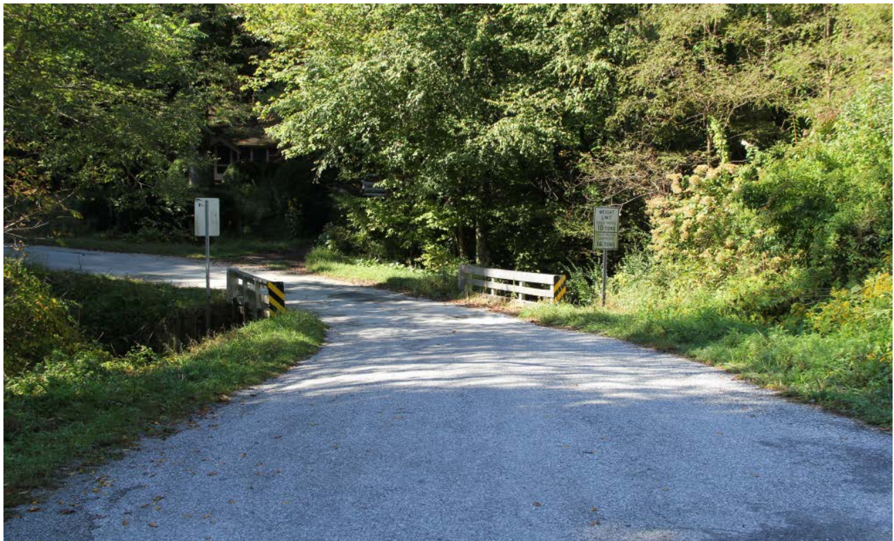
Bridge No. 261 on SR 1597 (Little Bearwallow Road) over Hickory Creek, view to southwest
