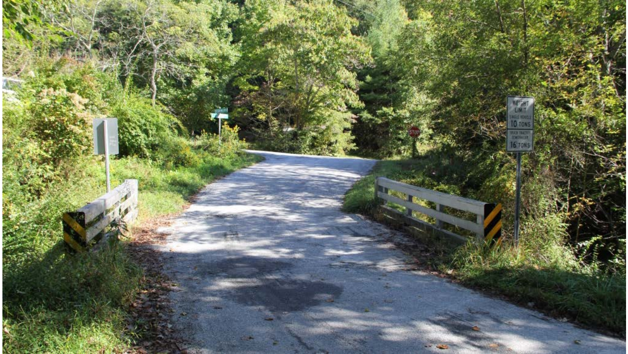
Bridge No. 261 on SR 1597, view northeast to intersection with Bearwallow Mountain Road (SR 1594)
