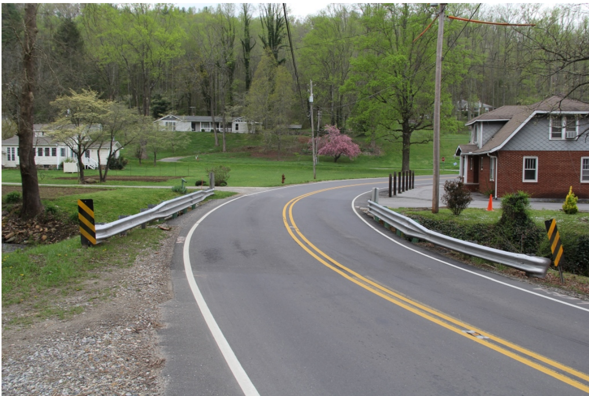
Bridge No. 11 on NC 143B/SR 1127 (Snowbird Road) over Long Creek, view to southwest [Bemis Lumber Company Office at right]
