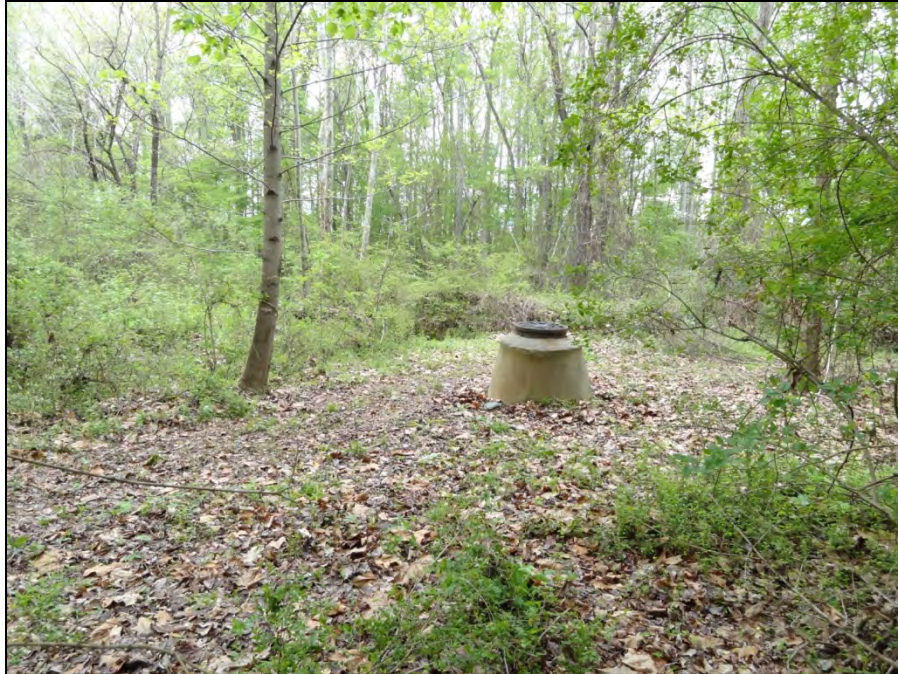
Figure 97. Access Road and Sewer Line/Culvert (foreground) and Stream (background) Northeast of STP 4A-a9, View Northeast.
