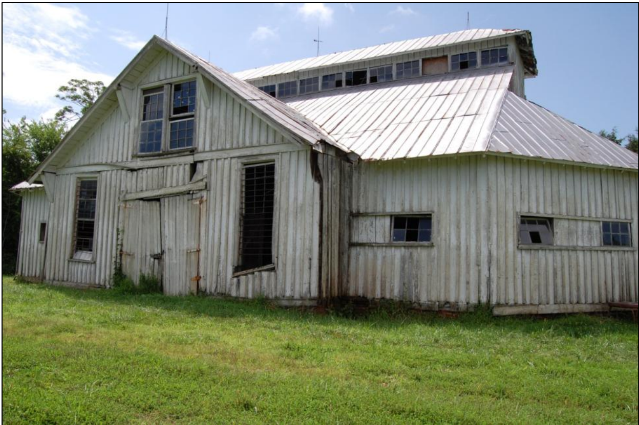
Campbell-Gray barn looking SW from lane that passes between the house and barn (Marvin Brown, August 2013)
