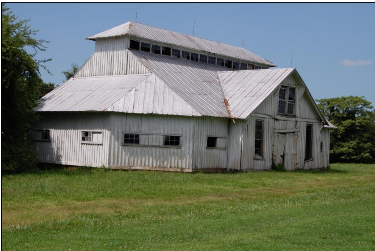
Campbell-Gray barn looking NW from lane that passes between the house and barn (Marvin Brown, August 2013)
