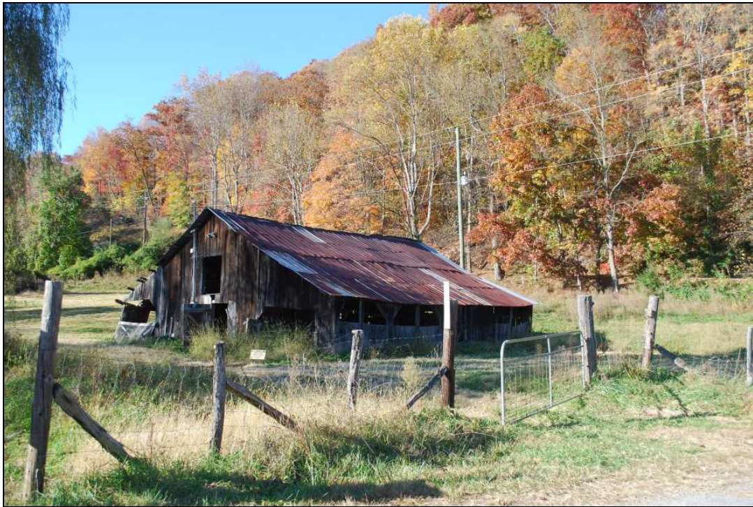
Two-story frame barn, looking northwest. Plott Creek runs in front of this structure.
