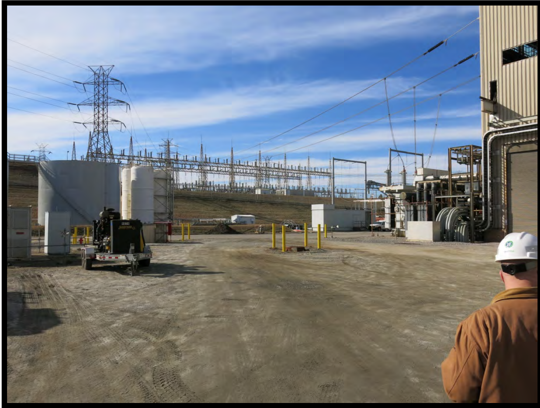
Figure 71: Marshall Steam Station (# 99), Fuel & Urea Tanks (left) and Switchyard (center), Looking West.
