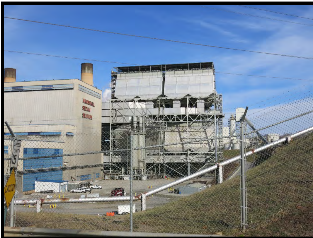
Figure 70: Marshall Steam Station (# 99), Precipitator for Units 3 & 4 (No. 4), Looking Northeast.
