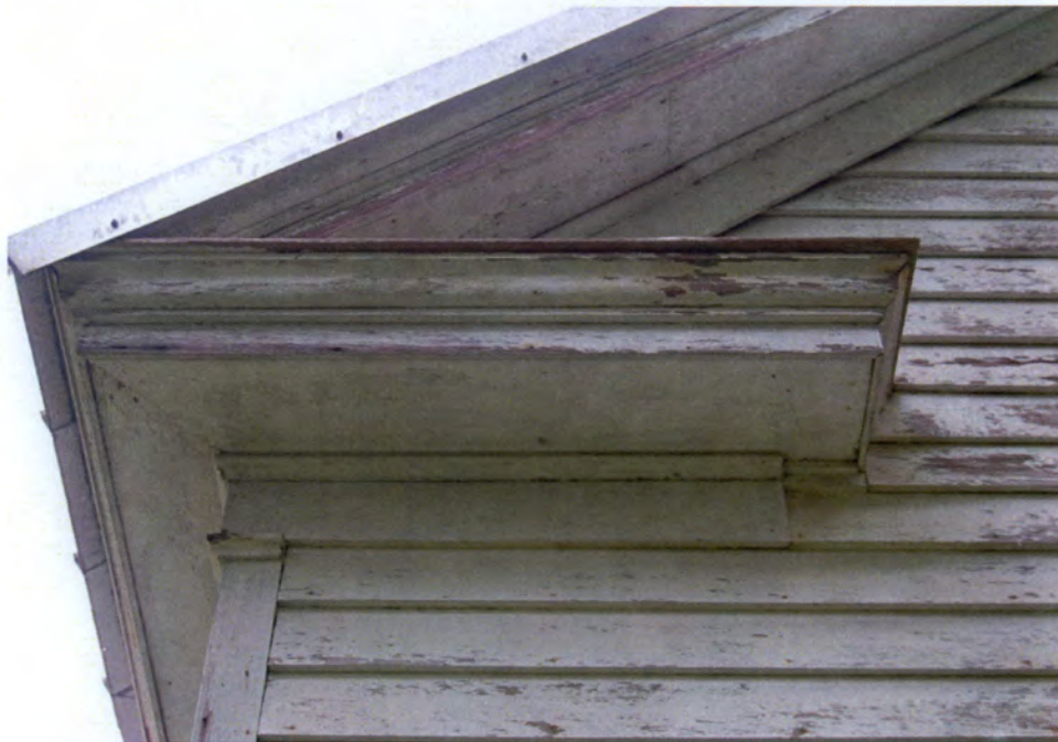
Plate 112. William Watts House, Detail of Cornice and Eaves, West Elevation, Looking East.
