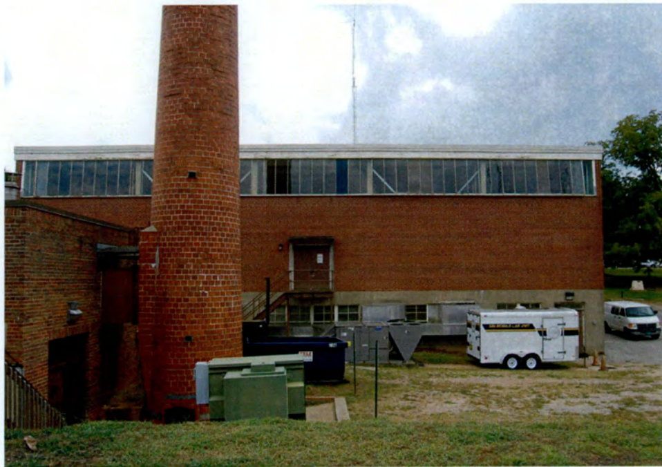
Plate 86. Governor Morehead School, Colored Department, Historic District, Gymnasium (circa 1960), North Elevation, Looking South.
