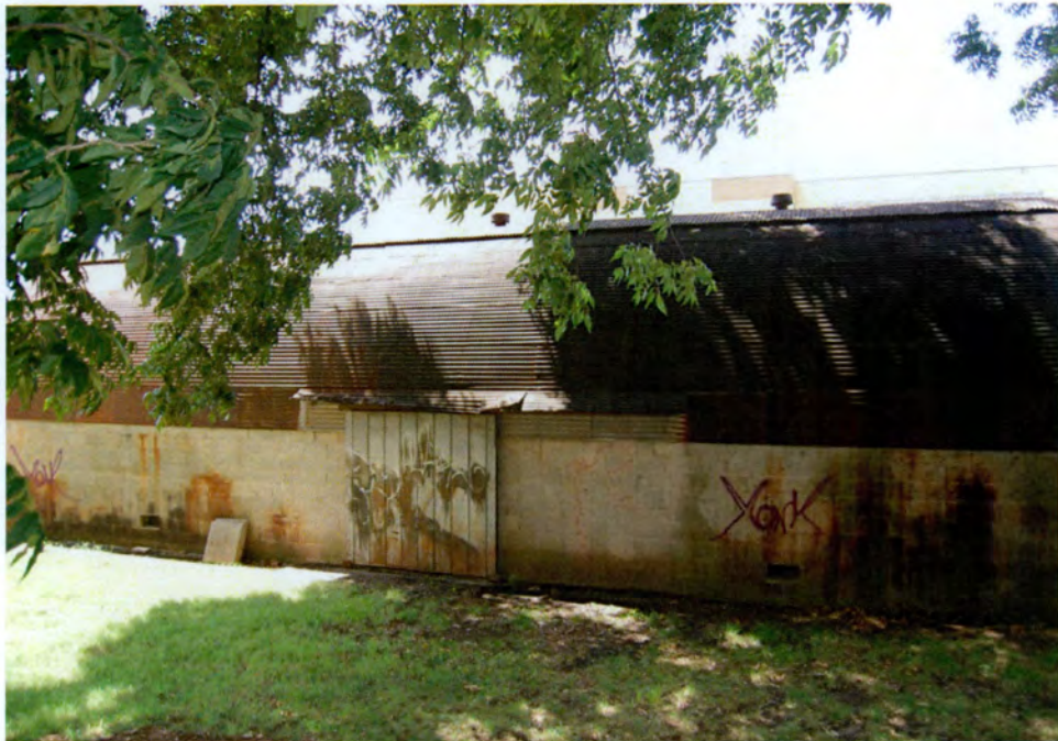
Plate 29. Raleigh Hosiery Company Building, Storage Building (1940s) in the Railroad Right-of-Way, Looking South.
