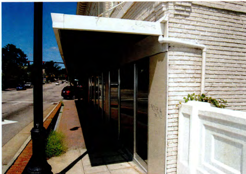
Plate 119. Commercial Block, First Story of Front Elevation, Looking West along Hillsborough Street.
