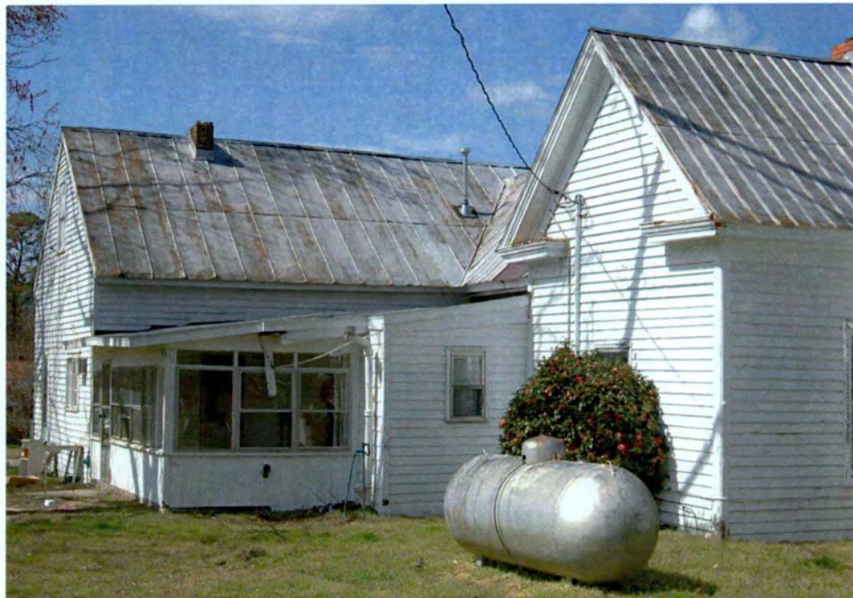
Plate 164. Watts Store and House, Rear Porch at junction of Store and House, Looking West.
