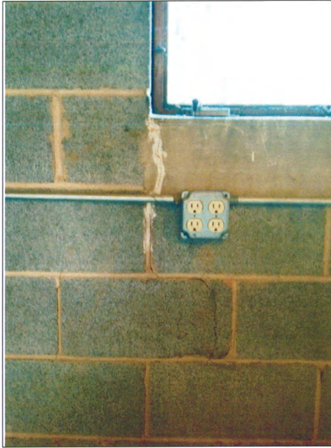
Figure 5.12. Detail of damage to interior of building 3502.
