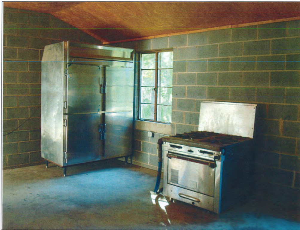
Figure 5.6. Building 3501 interior with stove and refrigerator.
