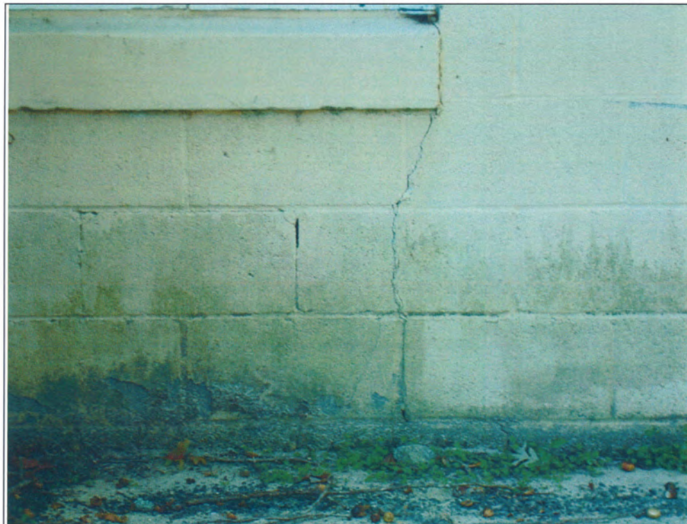
Figure 5.7. Detail of crack below window of Building 3501.
