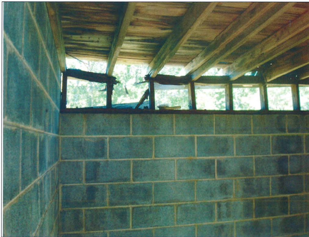
Figure 5.33. Interior of latrine showing deteriorated wood.
