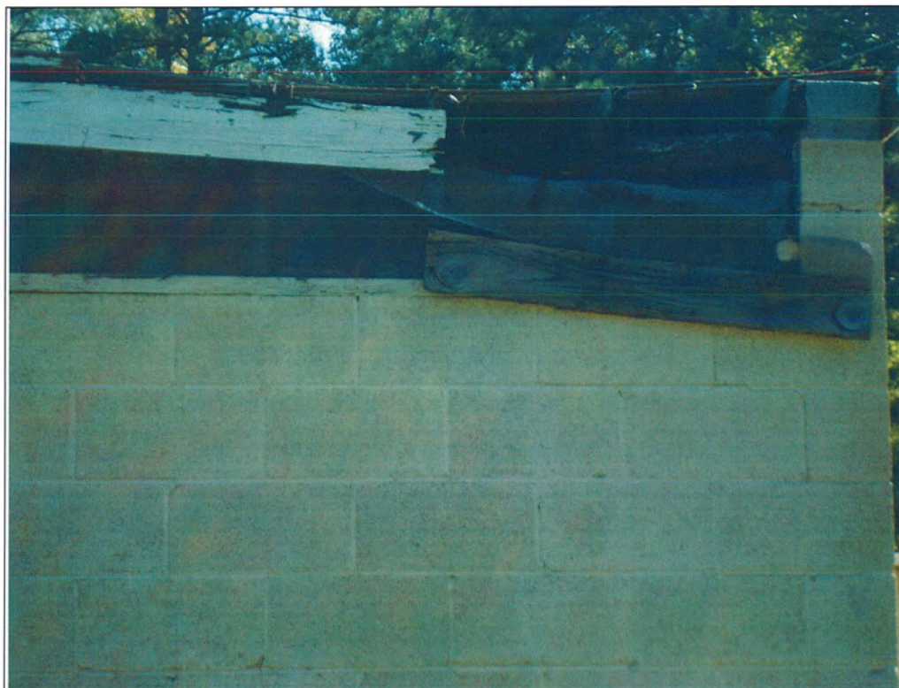
Figure 5.34. Exterior deterioration on the north elevation.
