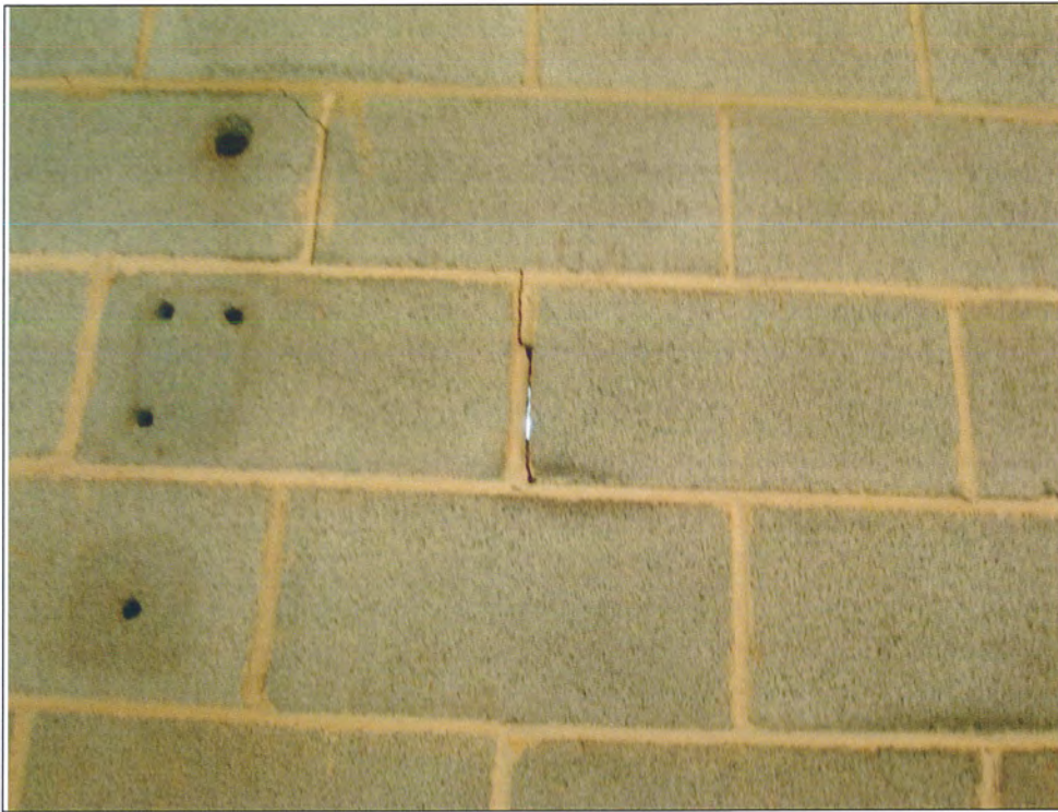
Figure 5.8. Detail of interior damage in Building 3501.
