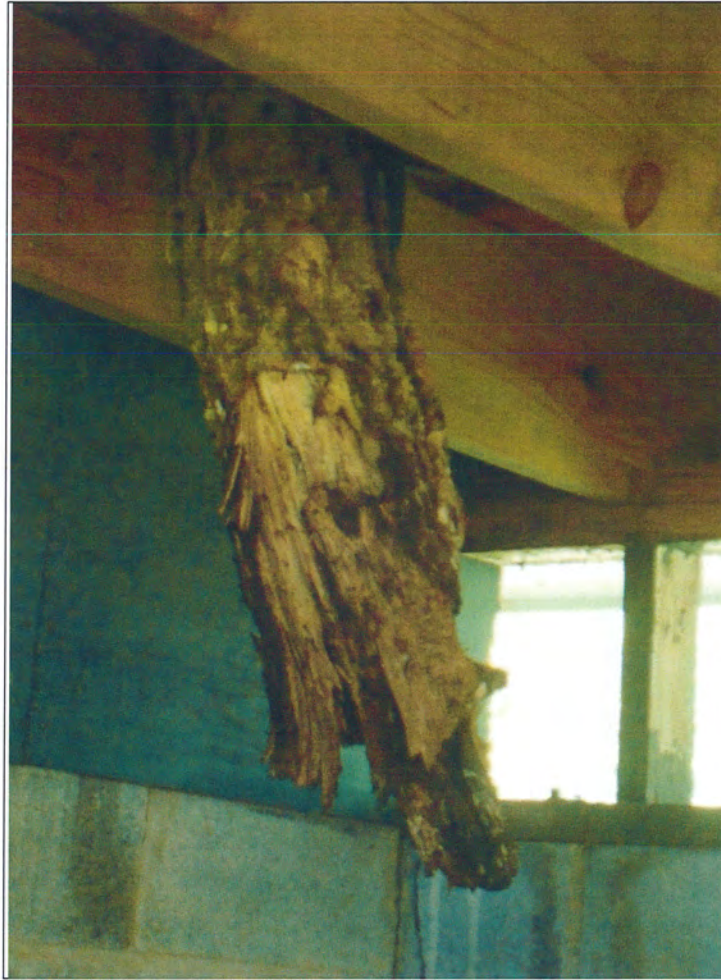
Figure 5.20. Tree limb protruding through roof and ceiling of male latrine in Building 3505.
