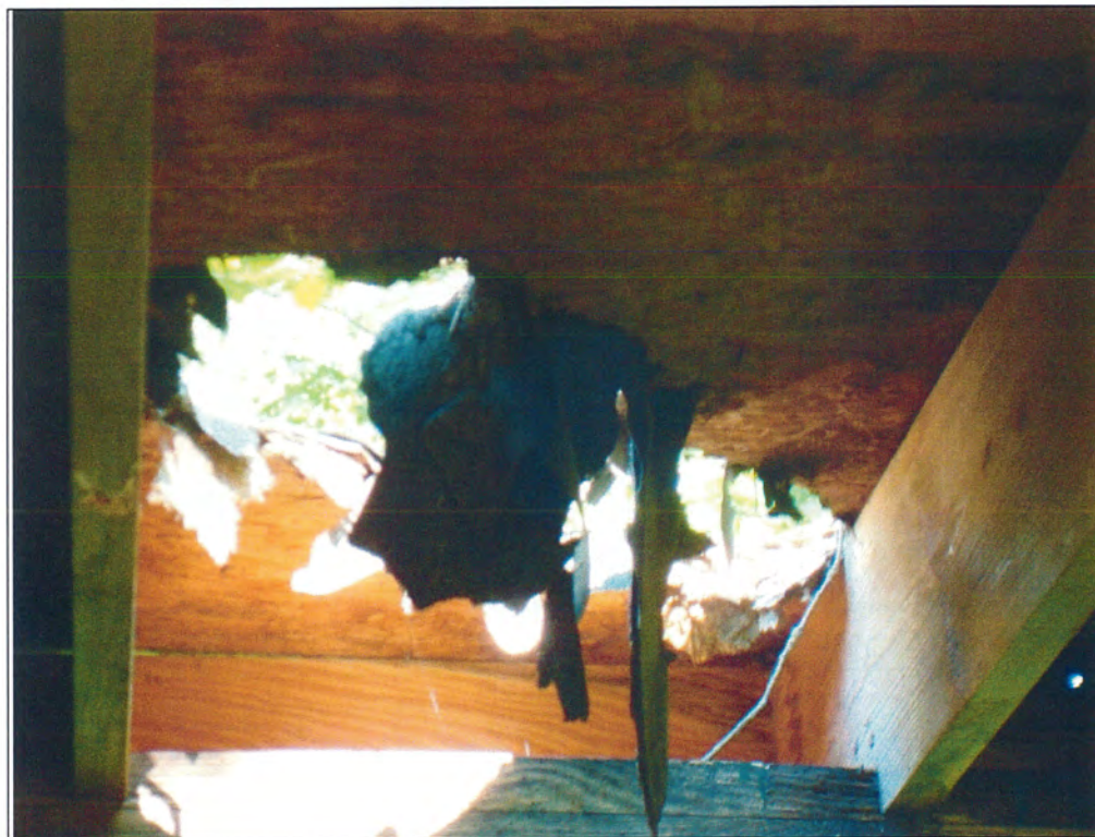
Figure 5.19. Hole in the roof of the female side of latrine in building 3505.
