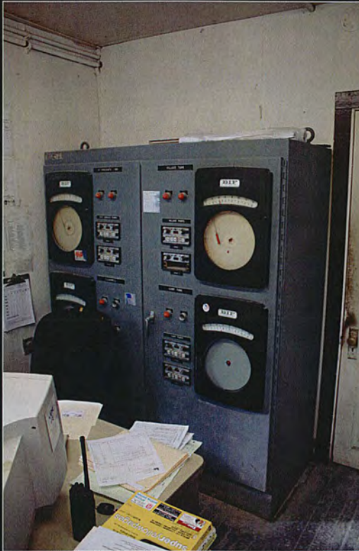
C. Original Plant Control System
