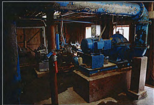
E. Water Pumps, View East
