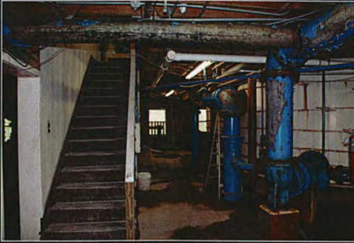
A. Stairway, Pumps, and Holding Tanks, View South
