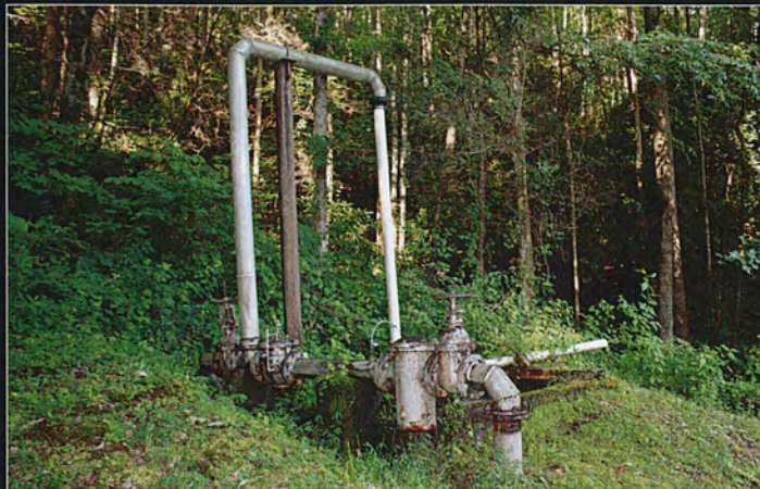
C. Intake Pump, View Southwest
