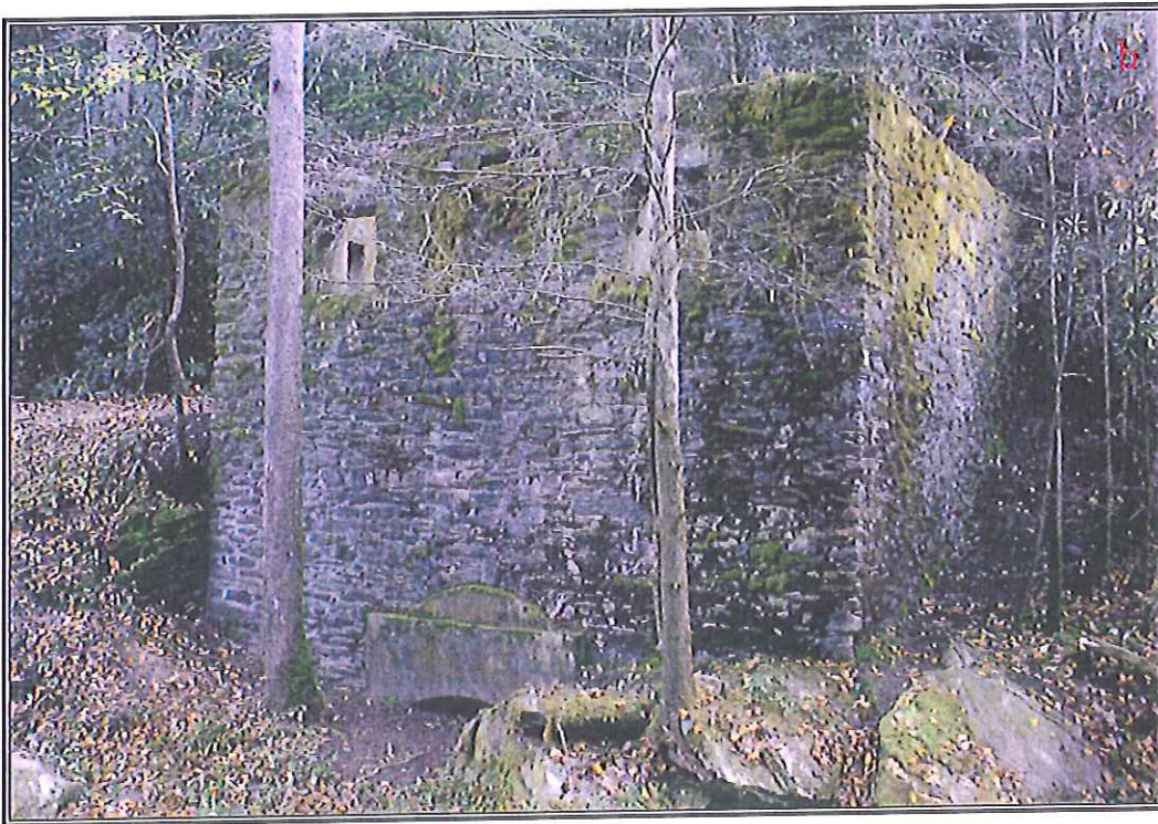
Figure 16. a) North wall front view of Power House No. 2, view to south; b) oblique view of north and west walls of Power House No. 2, view to southeast.
