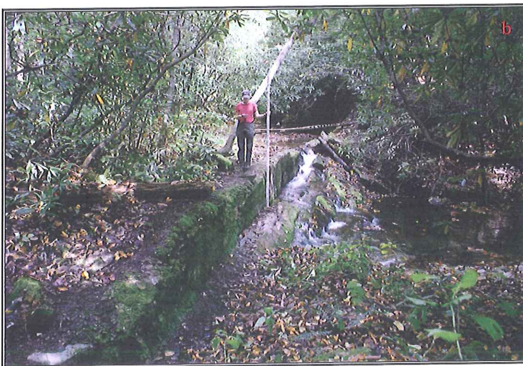
Figure 28. a) Front view photograph of Dam No. 2 at MC 209, view to north/northwest; b) oblique view of Dam No. 2, view to northeast.
