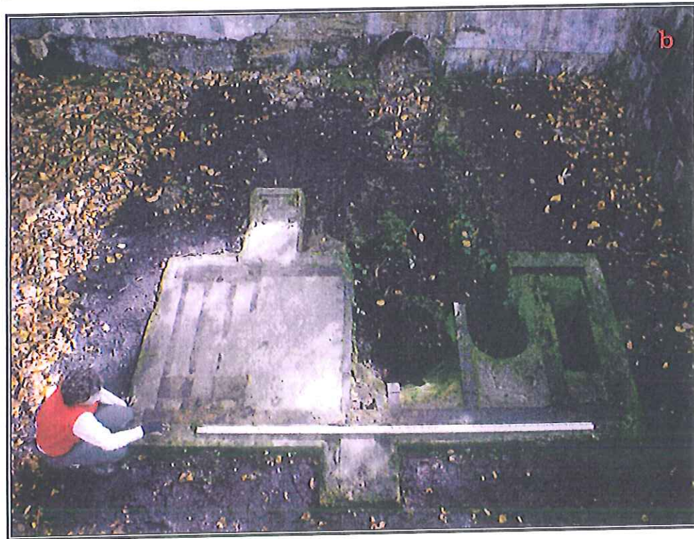
Figure 21. Photographs of generator platform at Power House No. 2: a) view to north; b) view to south.
