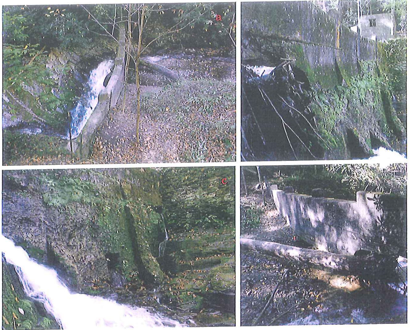
Figure 8a-d. Overview photographs of Dam No. 1 at MC 207: a) interior wall, view to southeast; b) exterior wall (top), view to west; c) exterior wall (bottom), view to west; d) breach at southeast end of dam, view to the north.
