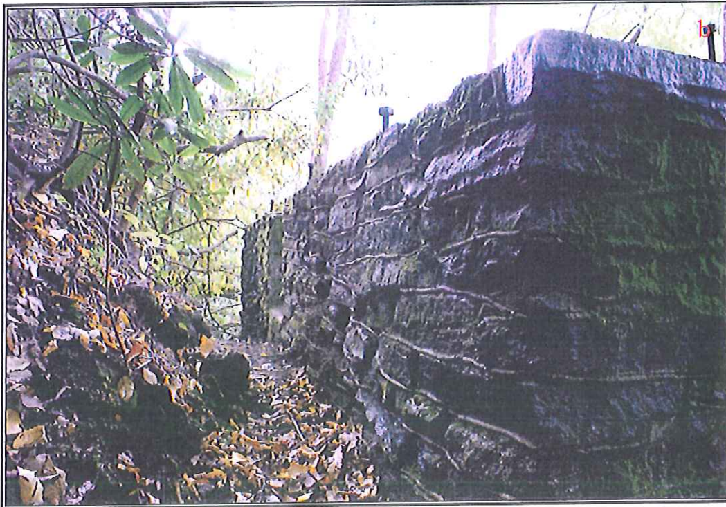
Figure 18. a) Oblique view of east wall at Power House No. 2, view to southwest; b) oblique view of south wall, view to west/northwest.
