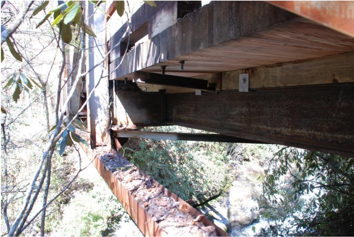
Photo 12. View of south side, looking west at lower portion of truss and underside of the roadbed.
