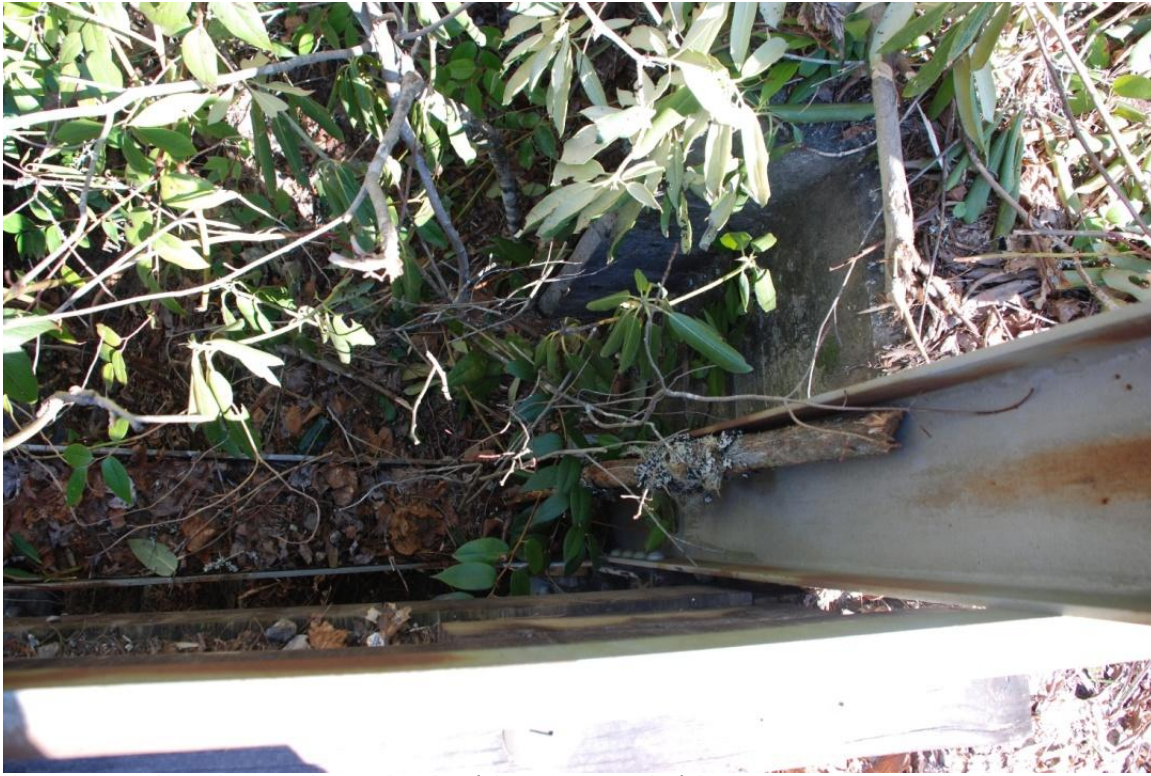
Photo 13. Looking down at the north side of the eastern end of the bridge (NL6) Note the heavy accumulation of debris on the lower chord of the truss and the heavy vegetation surrounding the foundation.
