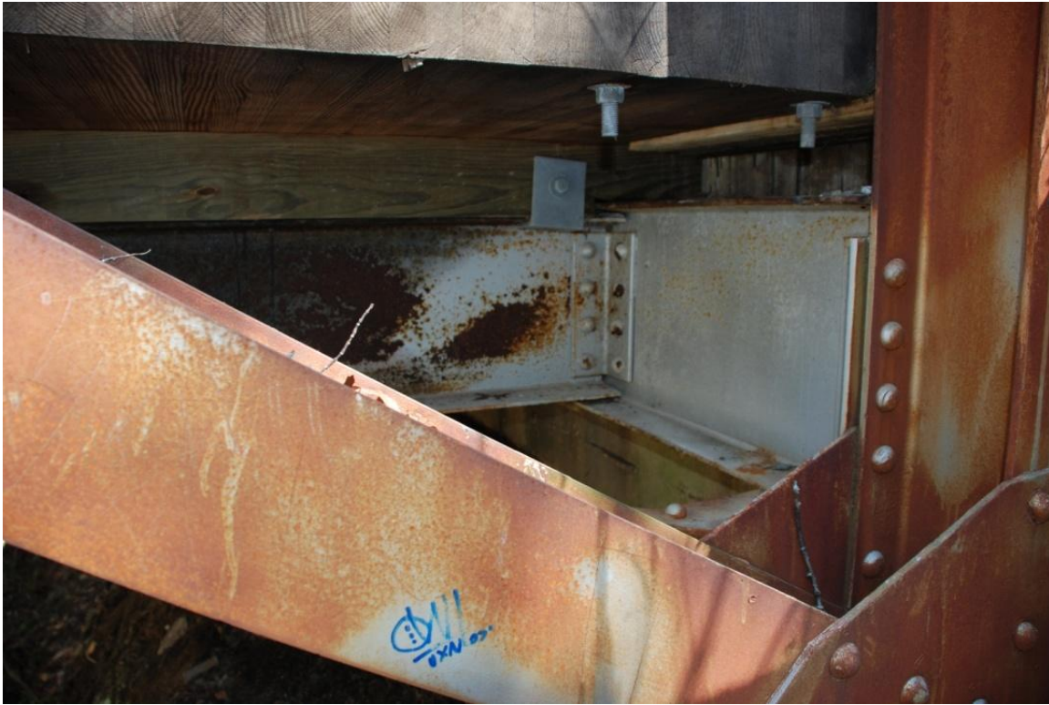
Photo 11. Base connection at the eastern end, including the underside of the wood road bed.
