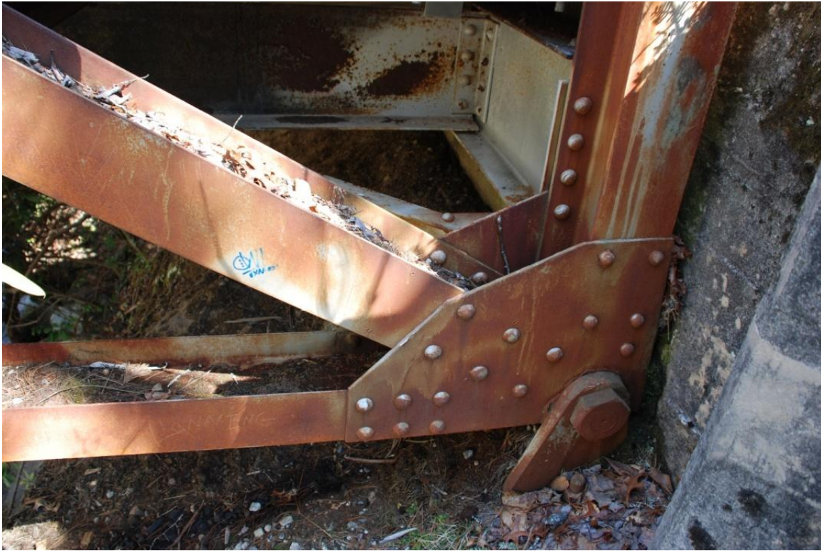
Photo 10. East base connection at S6L showing a fixed connection to the concrete foundation.
