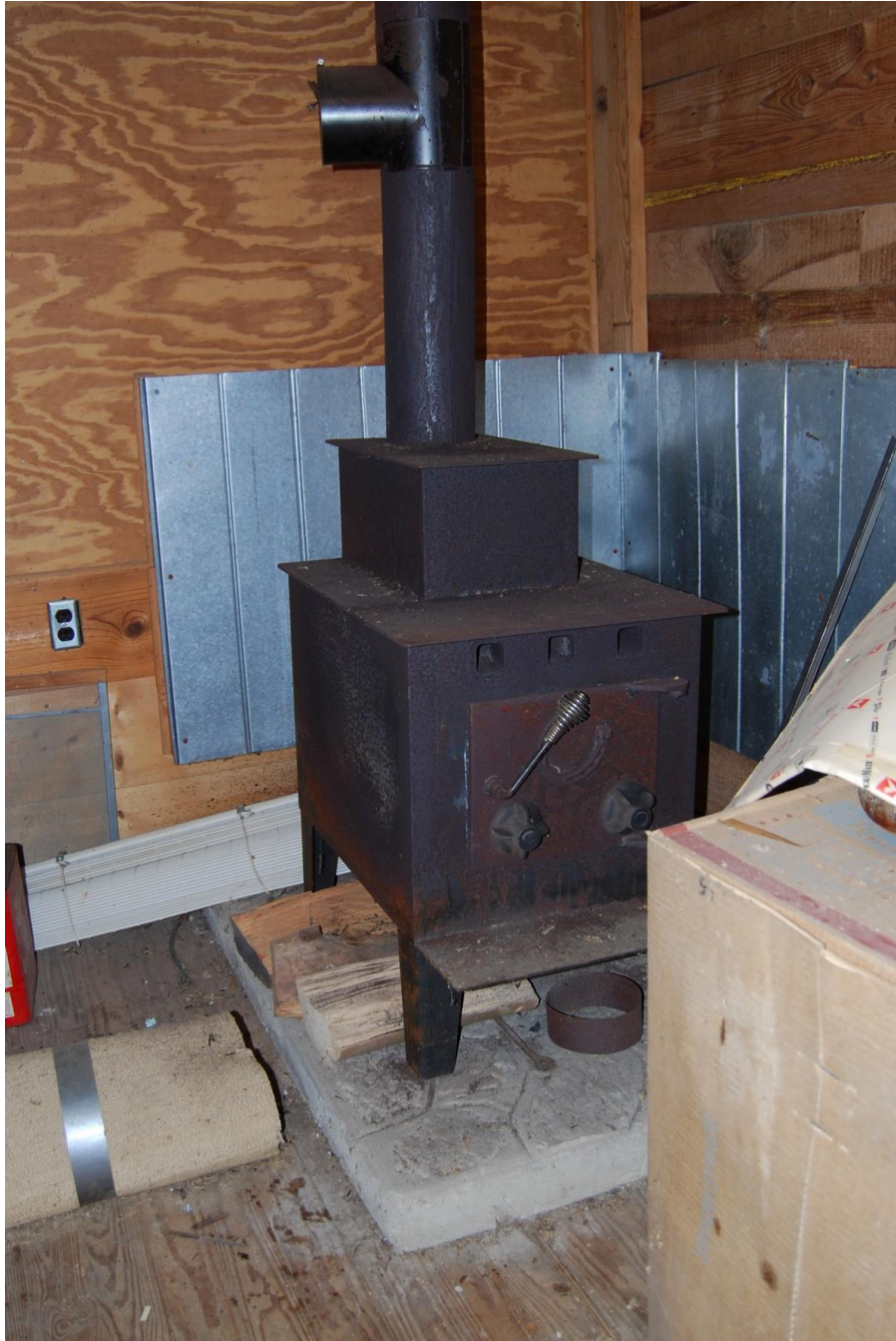
Wood stove on first floor of addition
