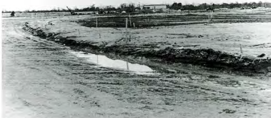
Figure 4-47. SAC alert complex under construction, ca. 1959. Note Building 2130 in background (Source: 4 th Wing History Office, Seymour Johnson Air Force Base, North Carolina).
