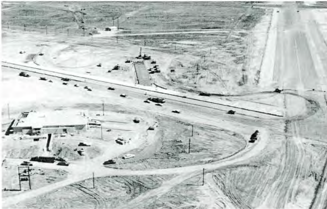
Figure 4-48. SAC alert complex under construction, March 19, 1959. Note Building 2130 on left hand side of photograph (Source: 4 th Wing History Office, Seymour Johnson Air Force Base, North Carolina).
