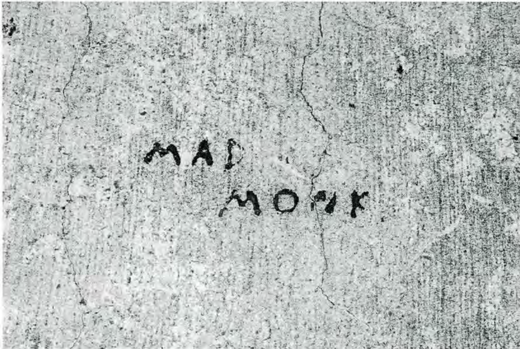
Figure 4-65. Graffiti on Christmas tree apron (Photograph by Joe C. Freeman, 2004).
