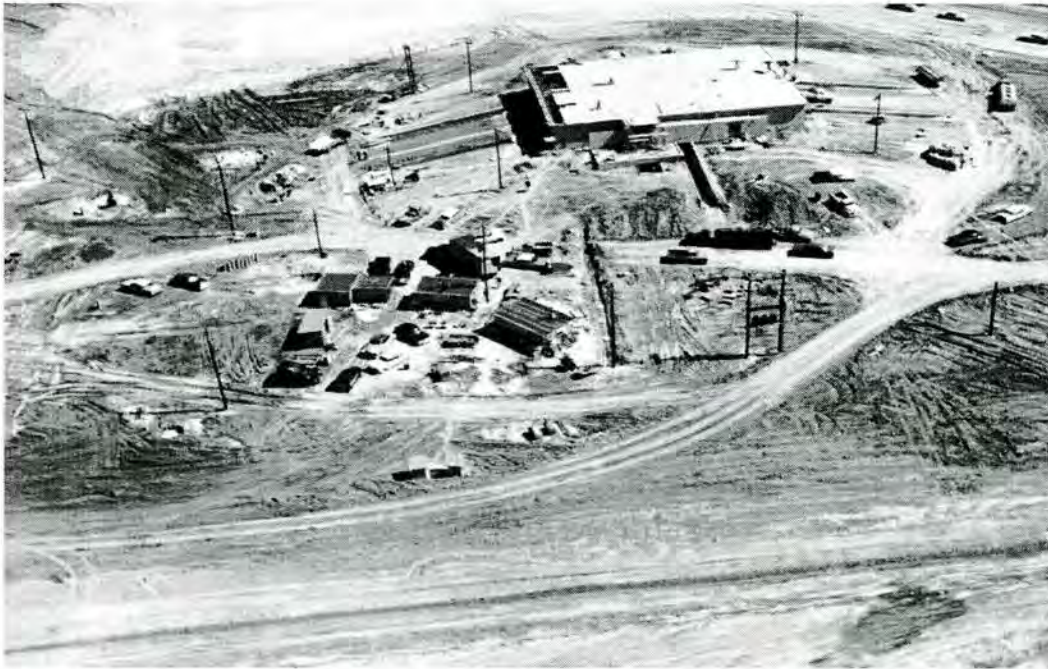
Figure 4-46. SAC alert complex under construction, March 19, 1959 (Source: 4 th Wing History Office, Seymour Johnson Air Force Base, North Carolina).
