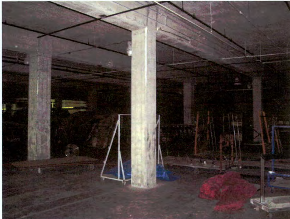
Plate 27. Chadbourn Hosiery Mills, Interior, Knitting Room, First Floor.
