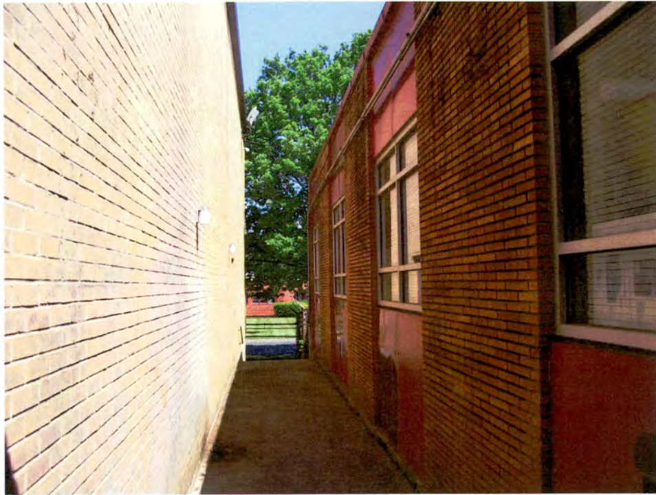
Plate 46. Standard Chemical Products Plant, Ramp Separating Office (Rear Elevation) and Warehouse, Looking North.
