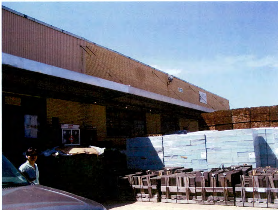
Plate 49. Standard Chemical Products Plant, Rear Warehouse and Loading Dock, North Elevation, Looking Southwest.
