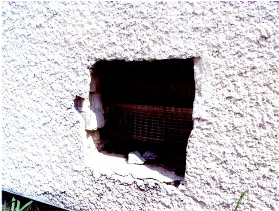
Kaiser Fluid Technologies Company Building (No. 72), Rear Warehouse, Detail of Stucco Covering Original Brick Veneer.
