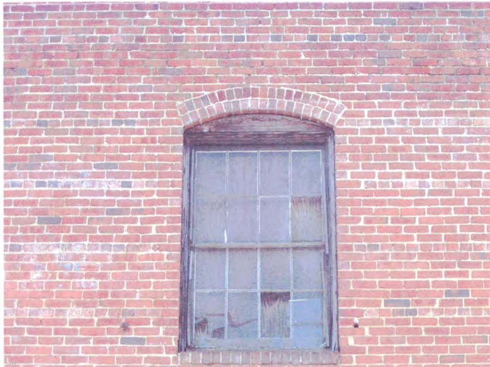
Plate 12. McNeil Paper Company Warehouse Complex, 301-303 East 8 th Street, Rear Elevation, Window Detail.
