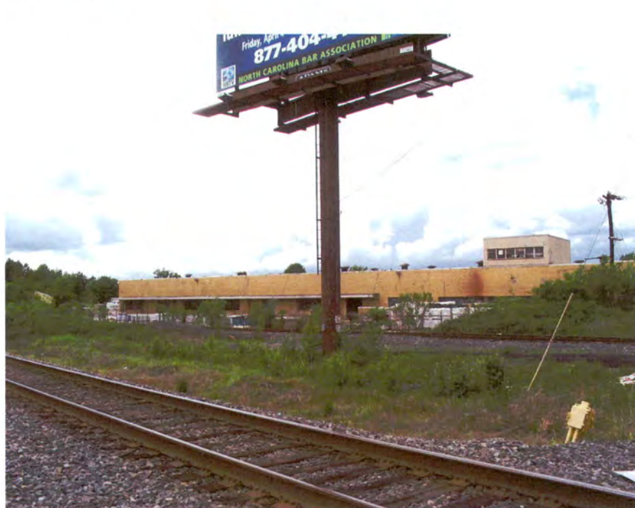
Standard Chemical Products Plant, Warehouse, East Elevation, Looking West From Railroad Corridor.
