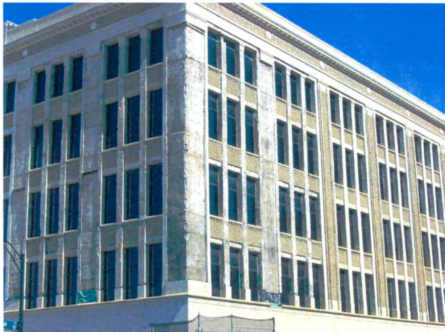
No. 2 Coddington Building (Polk Building), Deteriorated Walls.
