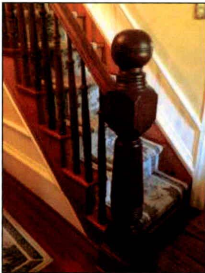
Figure 15: Interior of the William T. Smith House, newel post and stair detail
