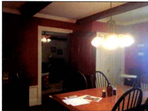
Figure 18: William T. Smith House, interior of dining room showing later dropped ceilings, facing southeast
