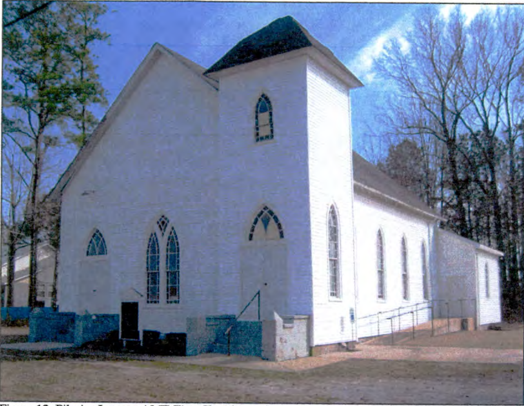
Figure 12: Pilgrim Journey AME Zion Church, north elevation in March 2006 after 2003 hurricane damage to steeple
