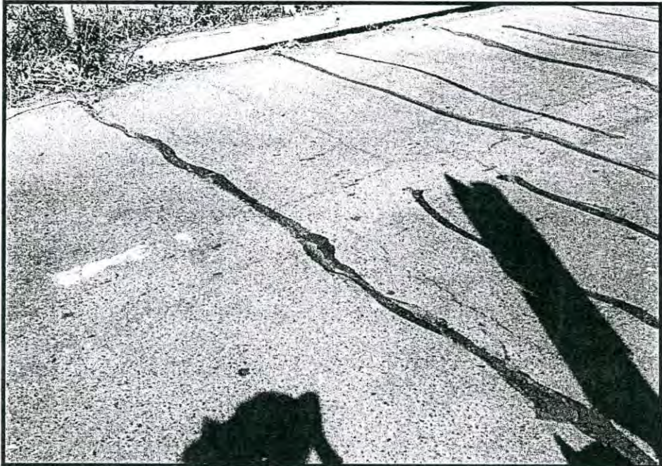
CRACK IN ASPHALT WEARING SURFACE AT ABUTMENT 1
