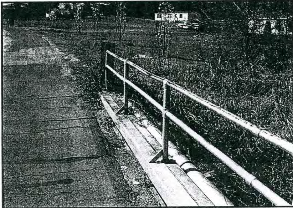
DAMAGED RAIL AT NORTHWEST CORNER OF SPAN A NEAR ABUTMENT 1
