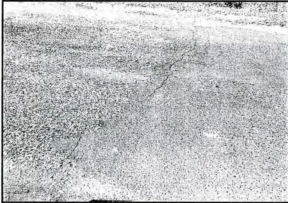
TRANSVERSE CRACK IN ASPHALT WEARING SURFACE ON WEST APPROACH ROADWAY
