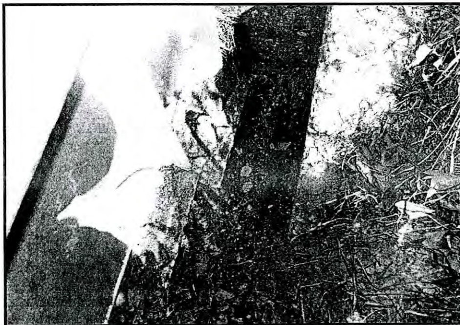
SOIL ON BEARING UNDER GIRDER 2 AT ABUTMENT 2
