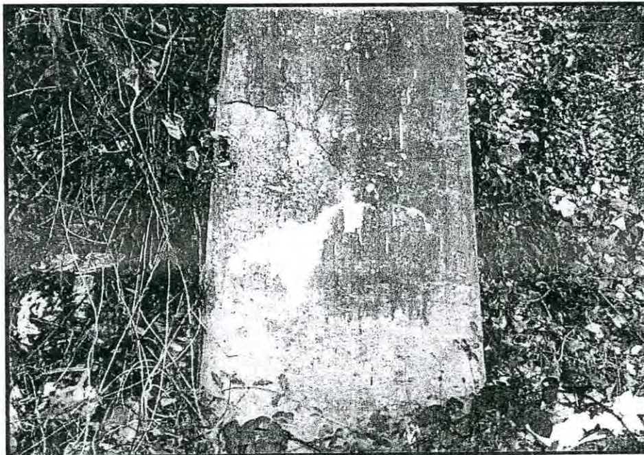
DIAGONAL CRACKS WITH EFFLORESCENCE IN CONCRETE PEDESTAL AT COLUMN 1 OF BENT 1
