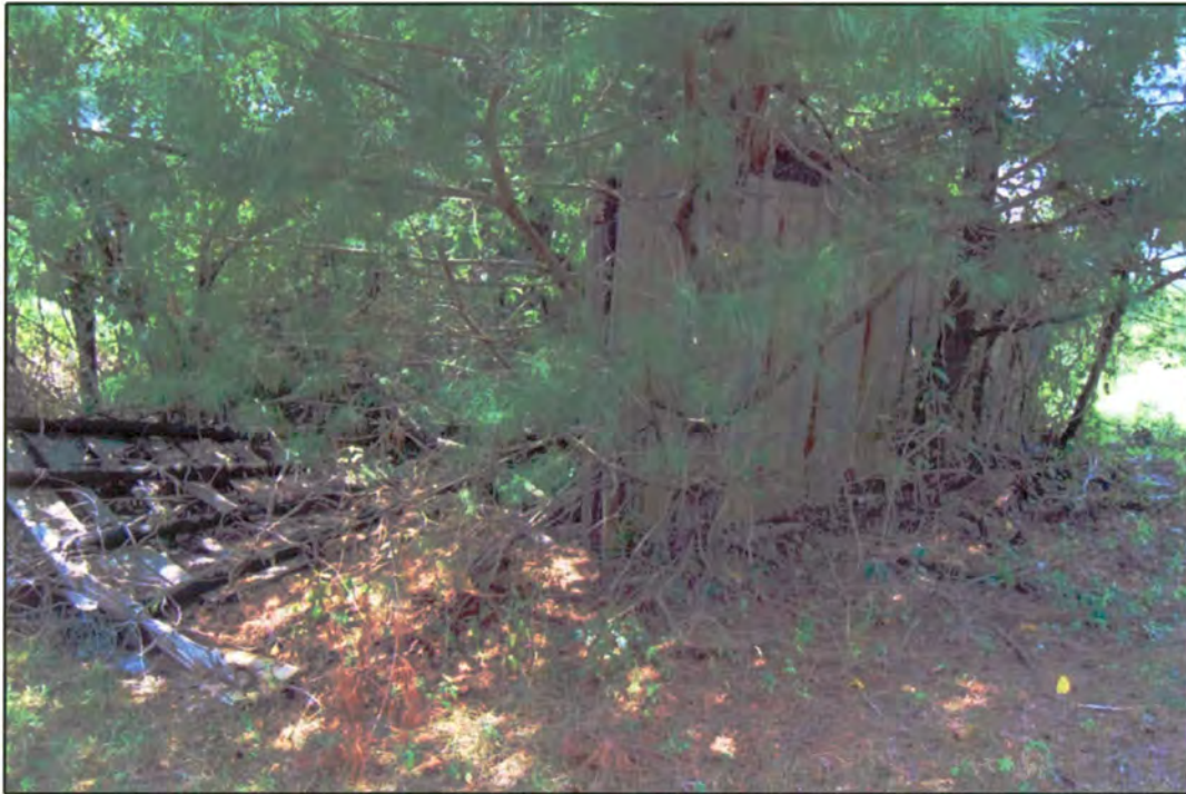
Figure 23. G. Haywood Hartley House: looking northwest at collapsed shed [F]
