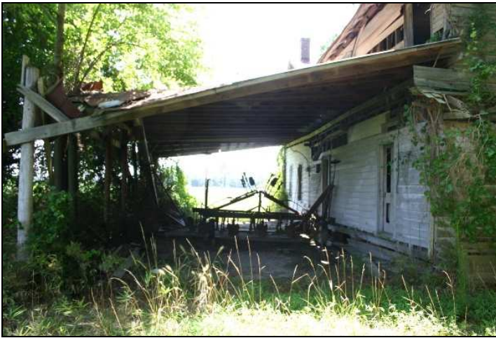
Figure 87: Whitmel Hill House, east elevation (with improvised tractor shed). Penne Sandbeck, NCDOT, August 2009.
