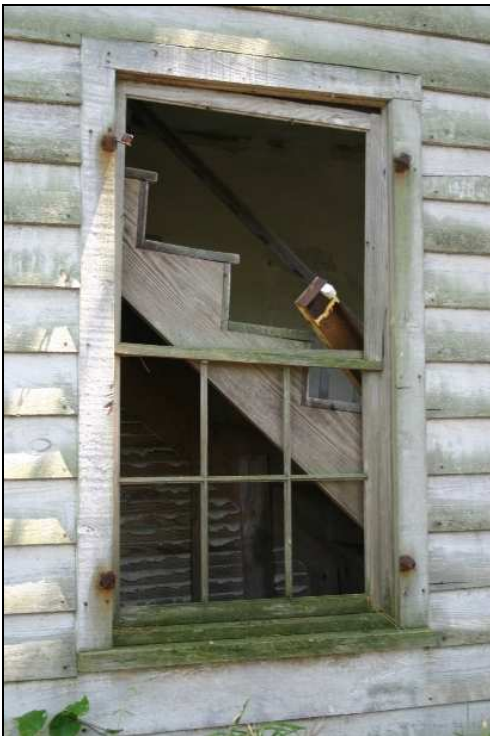
Figure 89: Whitmel Hill House, detail of window at west elevation. Penne Sandbeck, NCDOT, August 2009.
