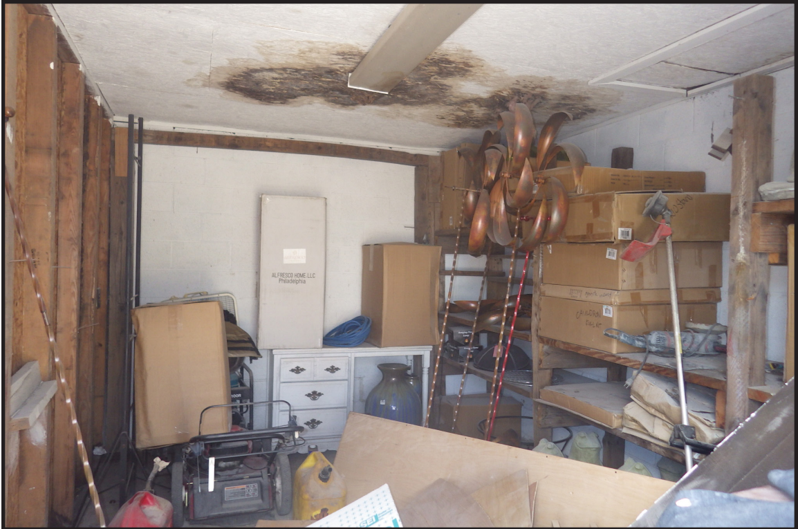
Figure 22. Typical Partitioned Room in Storage Building
