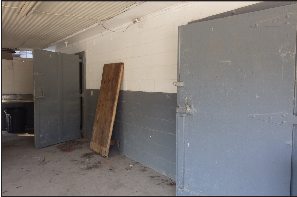
Figure 14. Processing Building, Southwest Side Under Shed Showing Middle and West Cooler Doors
