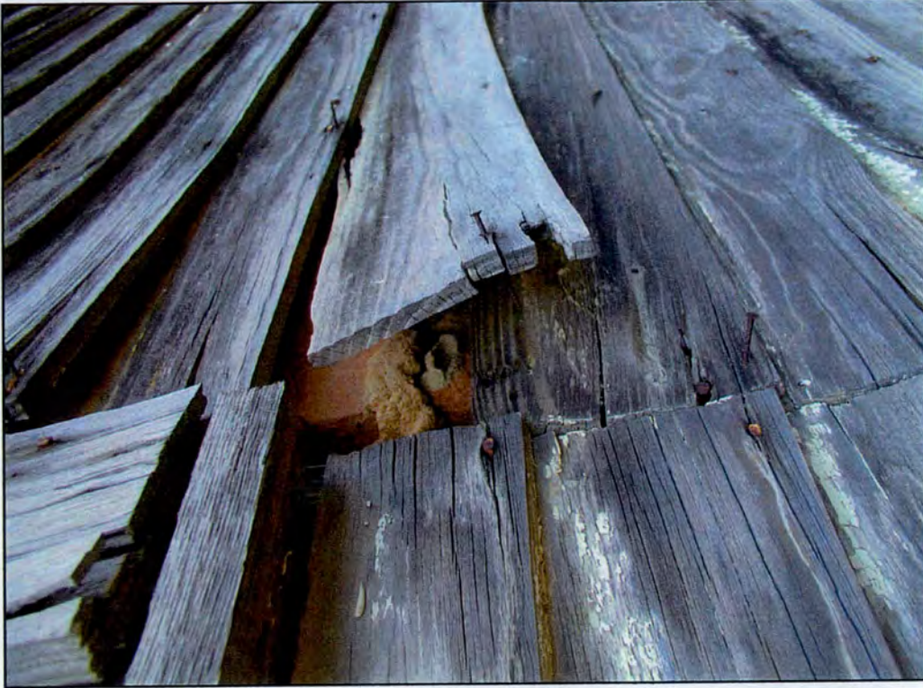
Detail of brick nogging in rear ell of Charlie Tucker House. NOT IN U-4909 PROJECT APE.
