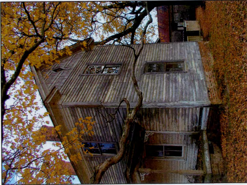
Detail of shingled eave, gable returns, and cornerboard and porch of Charlie Tucker House, looking southeast. NOT IN U-4909 PROJECT APE.
