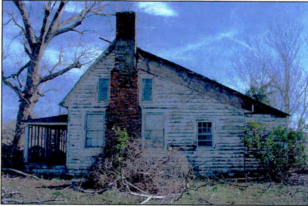
Photo 3: West side elevation. Note alteration of roofline and jalousie windows.
