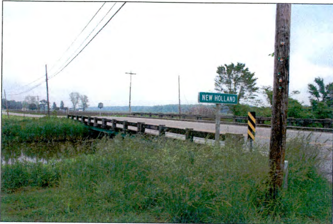
Property 6: Bridge No. 45 on US 264, over Central (N)/Outfall (S) Canal, from west
