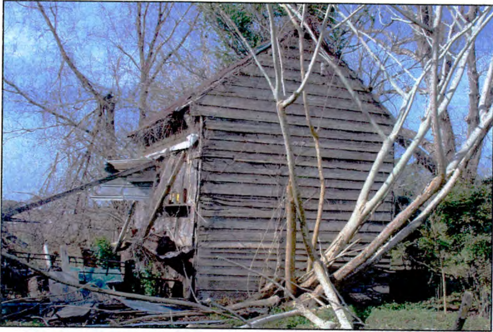
Photo 7: Smokehouse. Dilapidated shed addition on left side.
