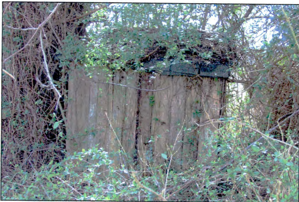
Photo 8: Deteriorated shed in dense thicket.
