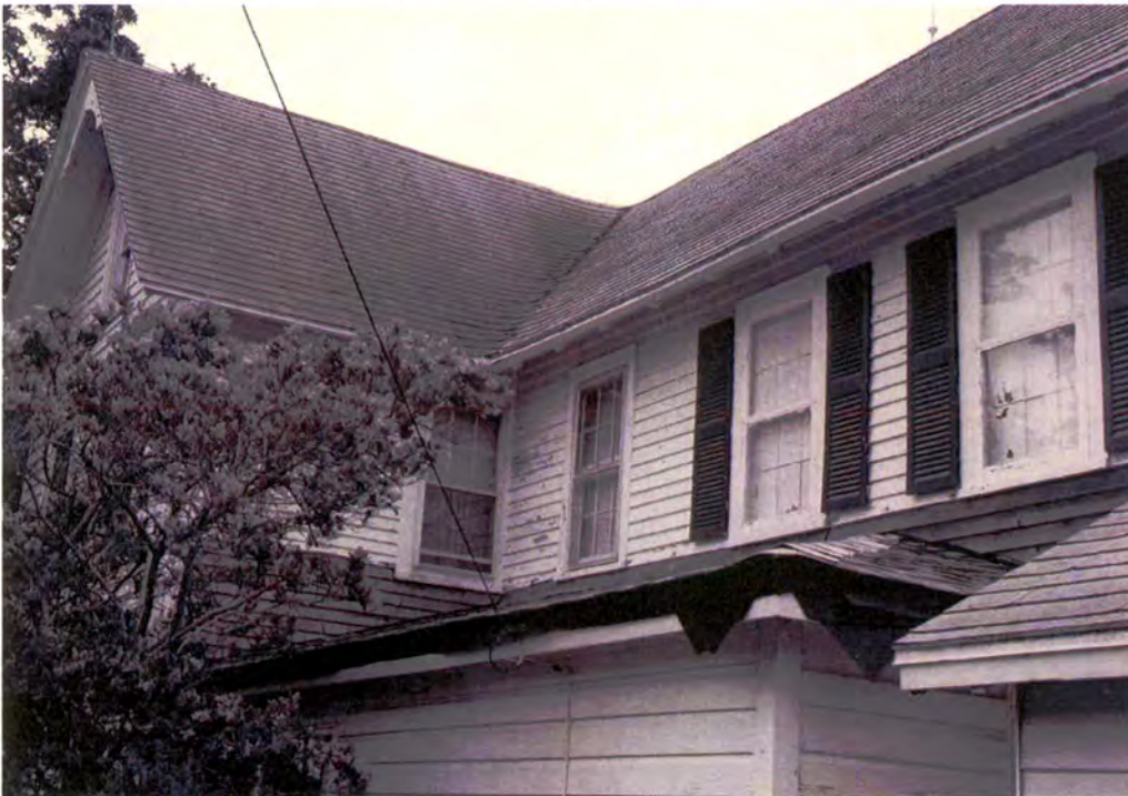
Plate 247: Urias O. and Caddie Midgett Gaskins House and Gaskins Cemetery (#8) – detail of east side and north rear elevations of house
