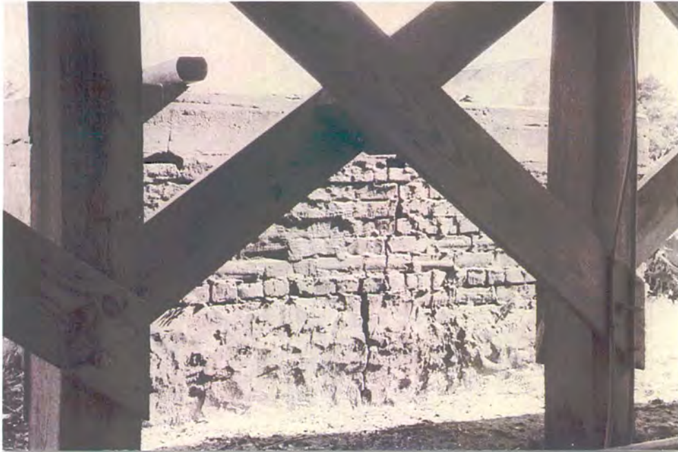
Plate 33: Rectangular brick cistern to rear of Avon's late nineteenth-century Oliver J. and Mary Midgett Gray House (#48), through modern house piers
