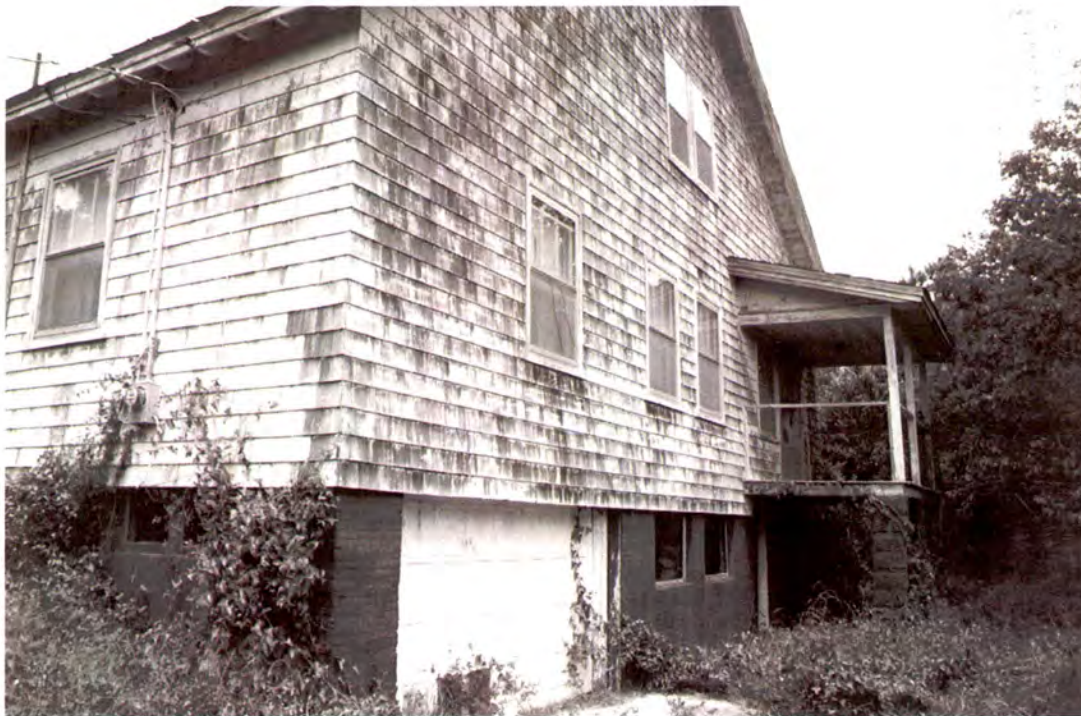
Plate 182: William L. and Courtney Gaskill Scarborough House (#27) in Buxton, south rear and west side elevations
