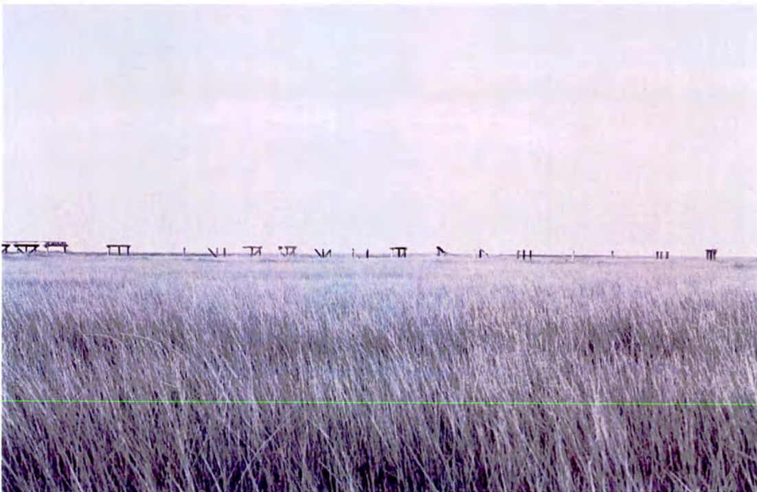
Plate 46: New Inlet Bridges – remnants of northern bents of northern bridge, looking northwest
