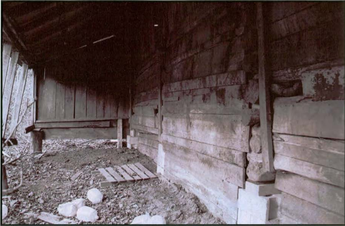
Plate 21: R.L. Hall Log Barn – west side elevation with frame infill at right center
