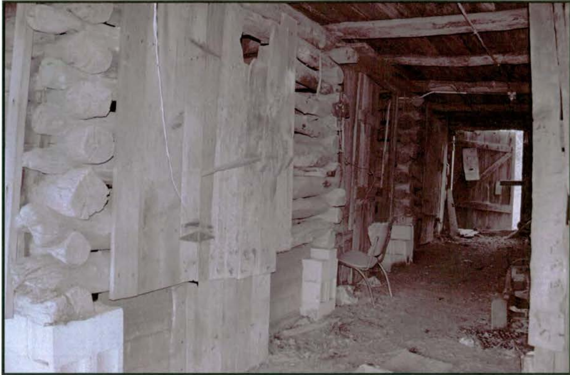
Plate 19: R.L. Hall Log Barn – transverse passage with southwest log crib/stall at left; note frame infill at center left near chair and also the altered base of the barn
