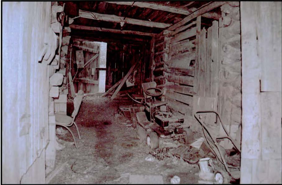
Plate 24: R.L. Hall Log Barn – looking north down transverse passage; note frame infill at right center
