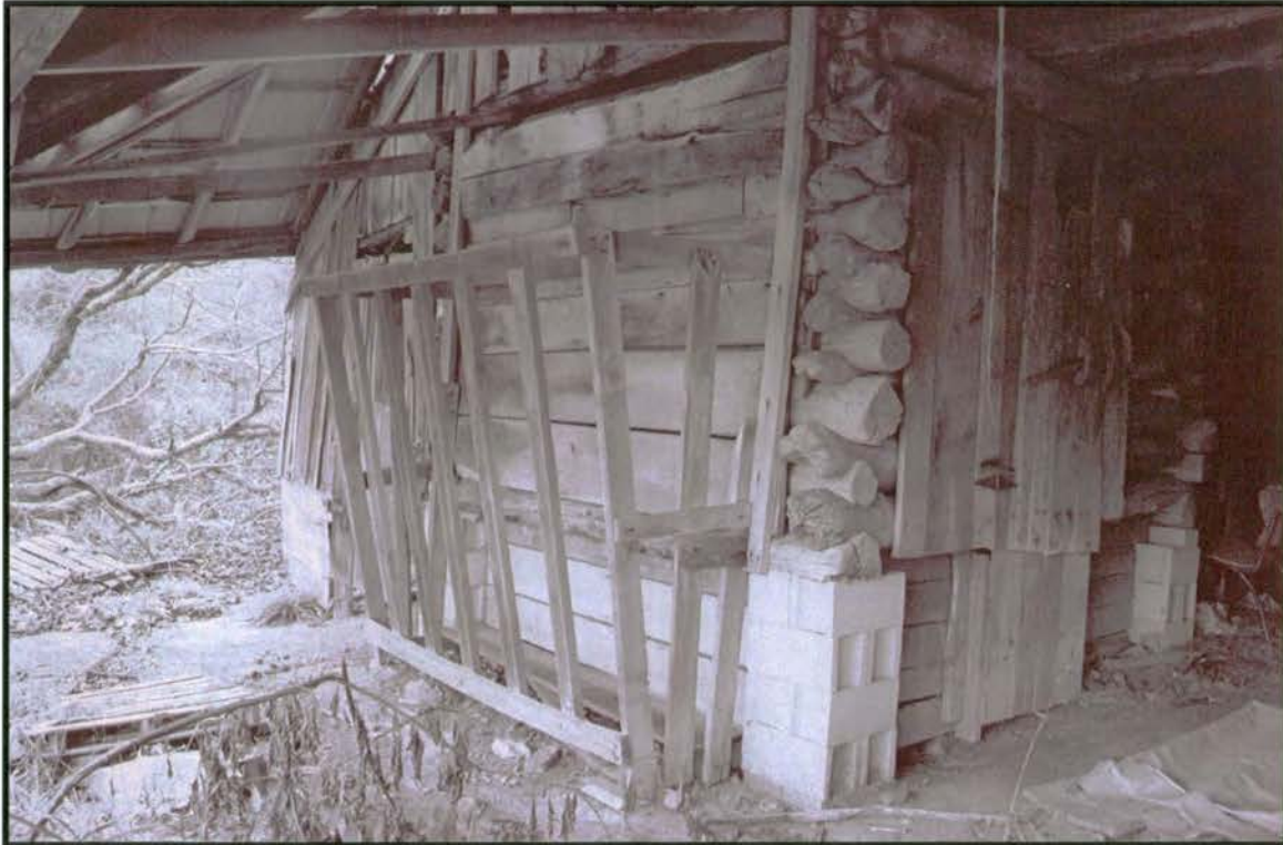
Plate 20: R.L. Hall Log Barn – east front elevation showing southwest log crib/stall and manger; note replacement of bottom logs and foundation with frame, boards, and cinder blocks
