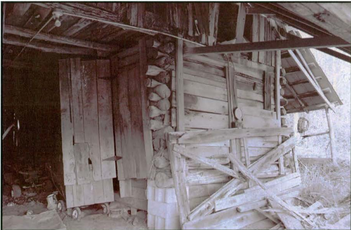
Plate 18: R.L. Hall Log Barn – east front elevation showing southeast log crib; note replacement of bottom logs and foundation with frame, boards, and cinder blocks
