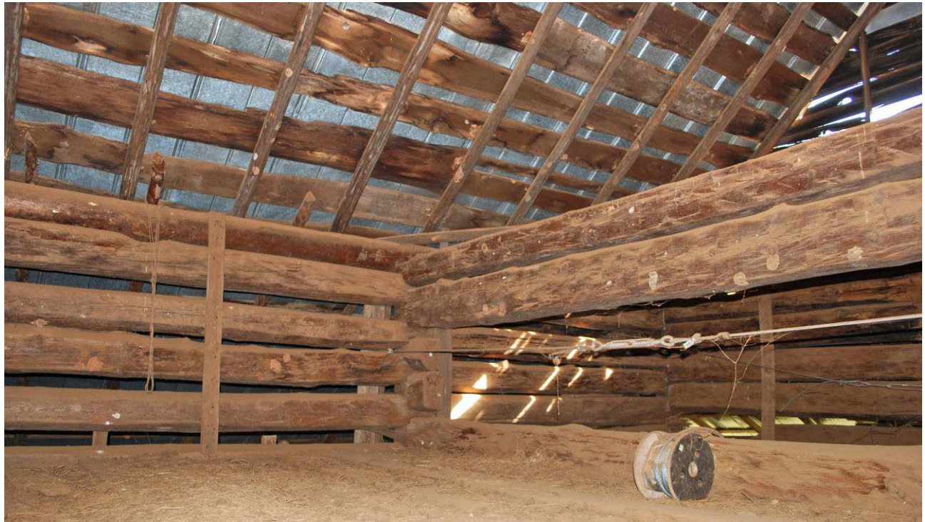
Barn loft, log walls, and roof system, looking northeast in central section
