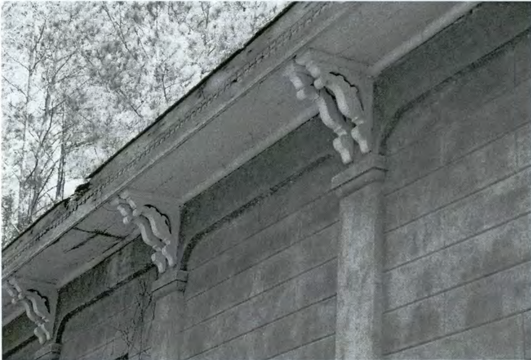
Penny Hill Doctor's Office, Detail of Scored Wall, Pilasters and Cornice on North Elevation
