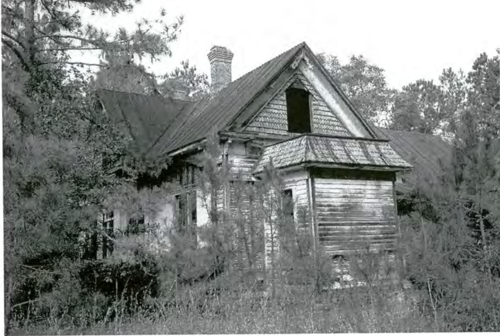
Property 37. Godfrey A. Stancill House (PT 612), circa 1880, east side of NC 33 0.2 mile north of intersection with SR 1409, Penny Hill, Pitt County
